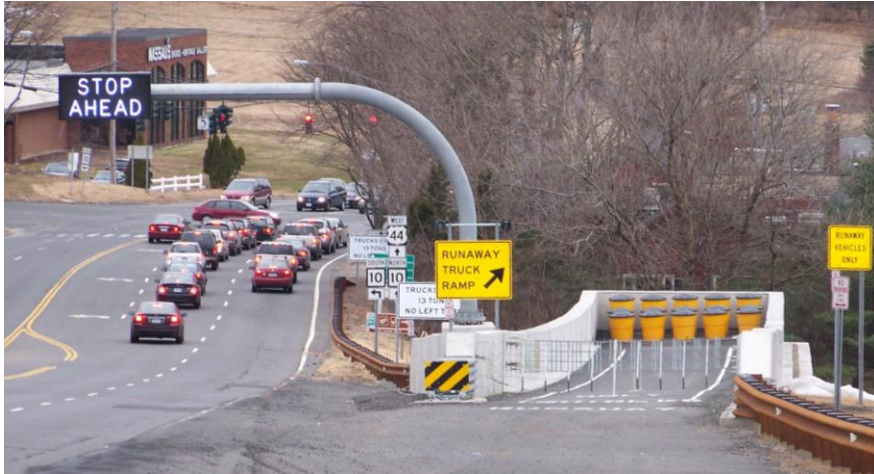
FIGURE 6. Truck Escape Ramp (TER) on Route 44 in Avon where Purinton Builders Inc. used the concrete maturity method during construction to complete the work in less than five months. Photo courtesy of Richard Hanley, et al. (14).
