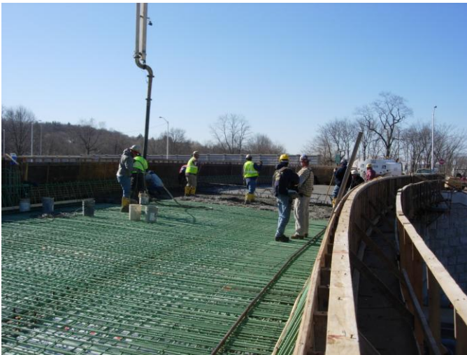
FIGURE 3. Concrete deck pour for Bridge No. 6610 where maturity probes were embedded on March 29, 2007.
