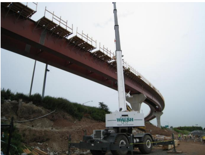
FIGURE 4. Route 34 ‘Flyover’ (Bridge No. 169) where concrete maturity and temperature monitoring was demonstrated at Project No. 92-619.
