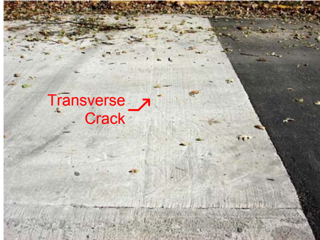
Figure 6–48. Transverse crack at North Riverside Drive SFSCC pavement located at NR-M3-A mix as of October 2008
