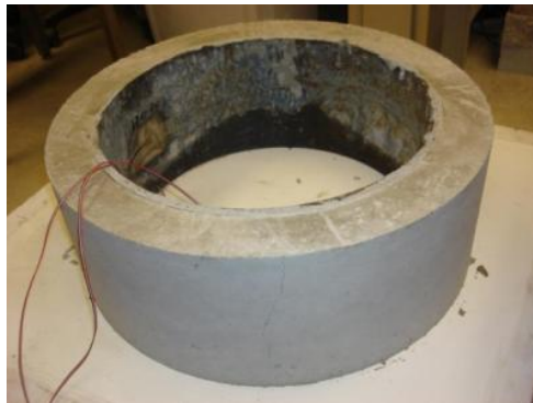
Cracked concrete ring
