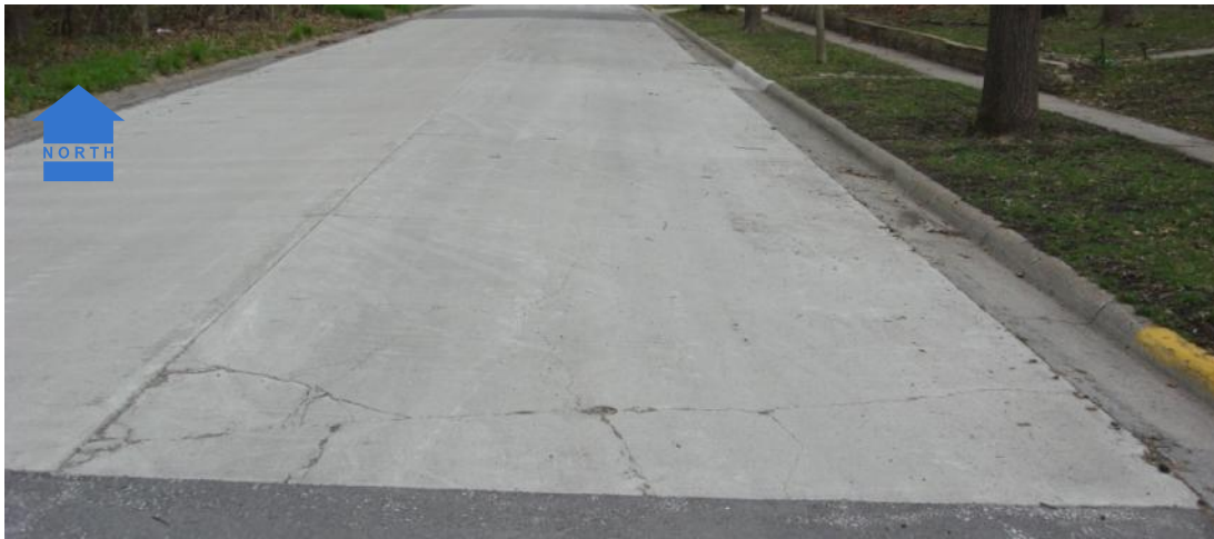
Figure 6-51. SFSCC pavement at North Riverside Drive as of April 2011
