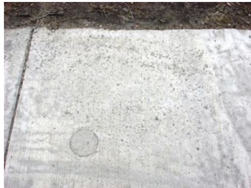
Figure 6–39. Scaling of SFSCC at South 4th Street in March 2009
