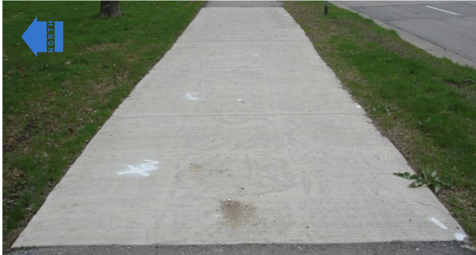
Figure 6–40. Condition of SFSCC pavement at South 4th Street on April 2011
