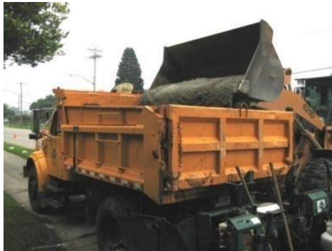
Figure 6–12. Concrete was first transported into a dump truck and then loaded into the paver
