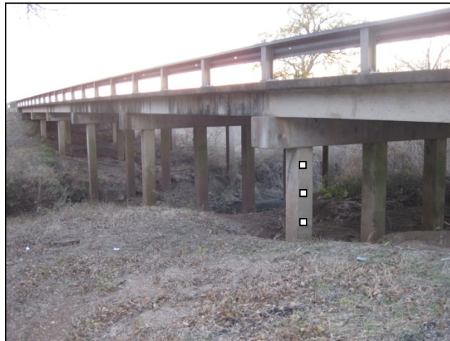
Figure 9-4. Accelerometers on Kountze Bayou Bridge.
