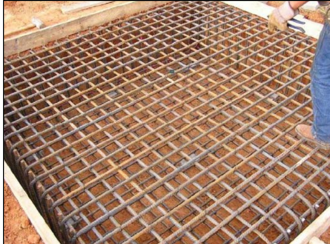
Figure 11-38. 3 \times 3 \times 1 \text{ m}^3 ( 9.84 \times 9.84 \times 3.28 \text{ ft}^3 ) Foundation during Construction (Dunn 2010).
