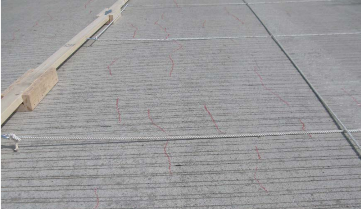
Figure 11 Traced Cracks on Bridge Deck with Grid
