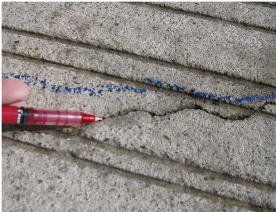
Figure 40 Structural Crack on Bridge Number ASD-42-0656
