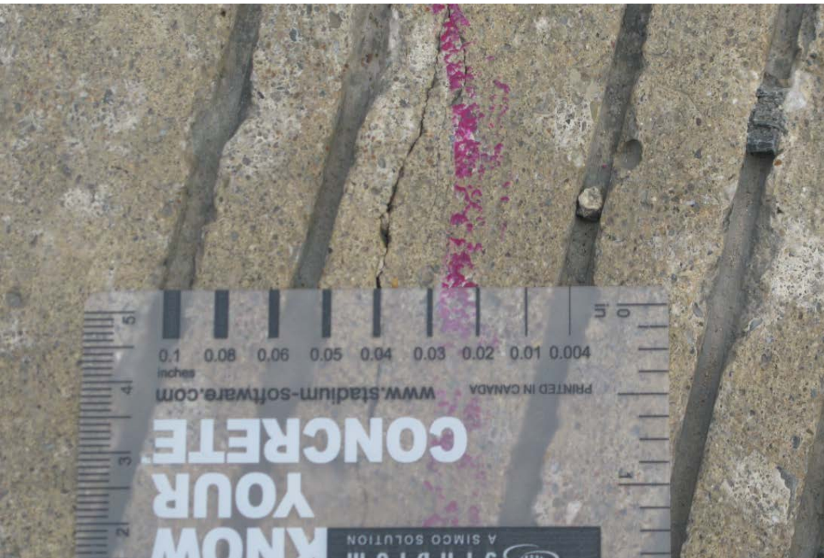
Figure 12 Example of Concrete Crack
