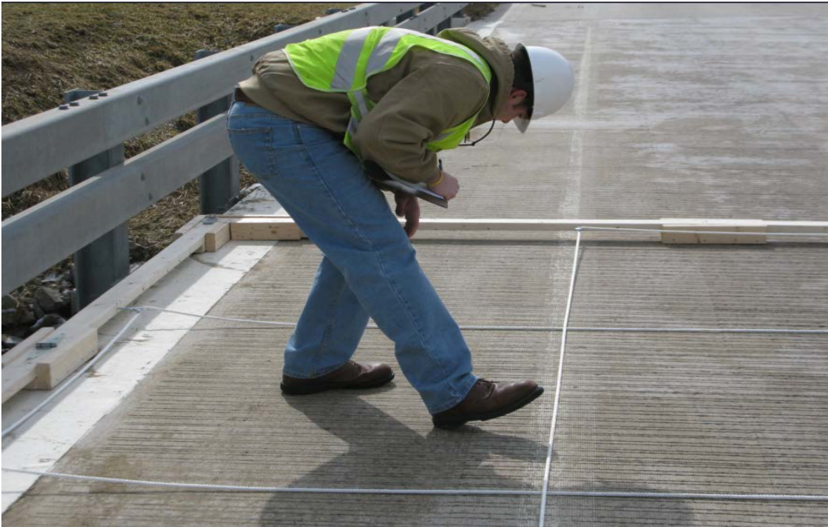
Figure 7 Typical Crack Survey
