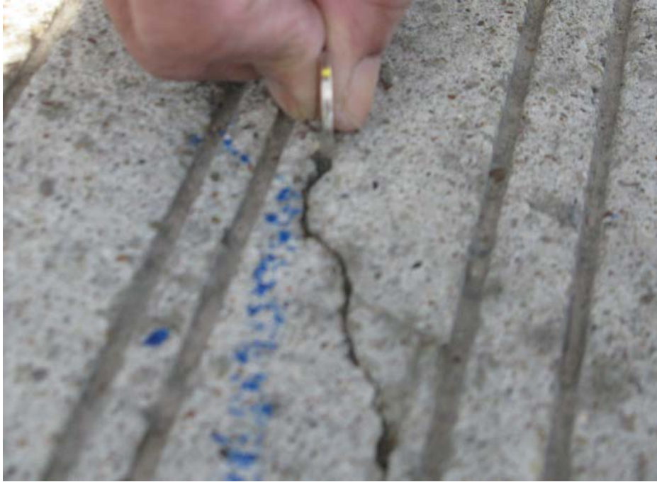
Figure 41 Structural Crack on Bridge Deck
