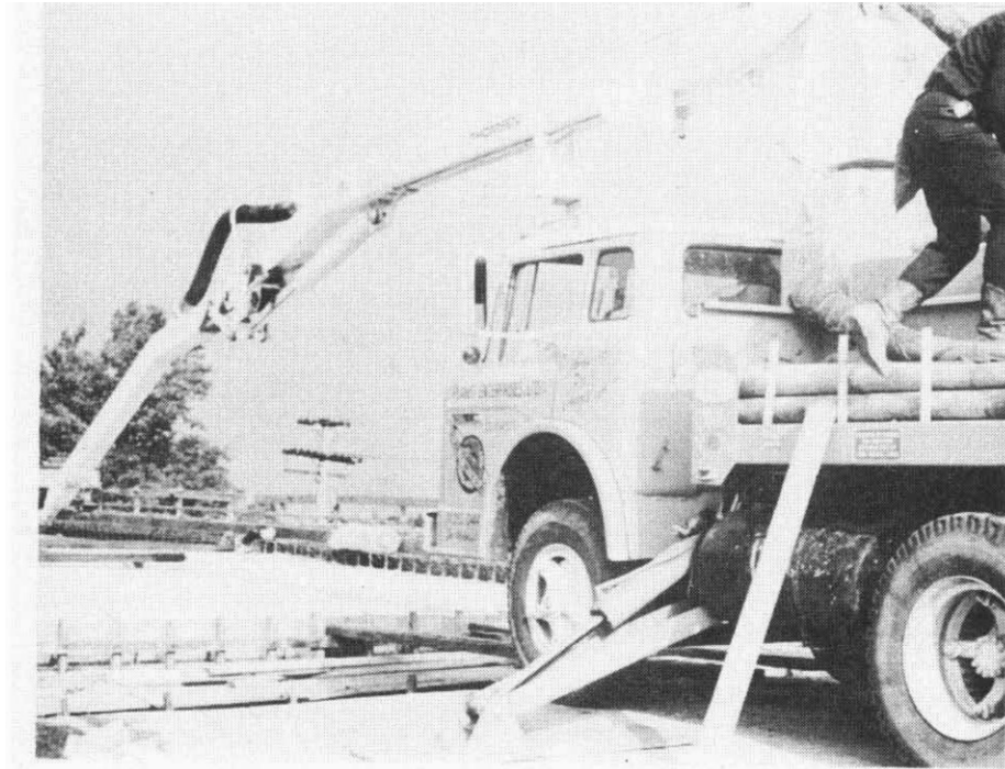
8 inch double piston pump with 5 inch discharge hose to the bridge floor.
