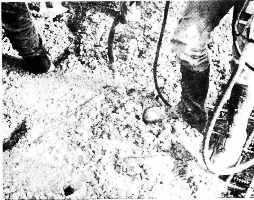
Vibrator not too effective after 40 to 50 minutes from batching - note hole left by vibrator in lower left of picture.
