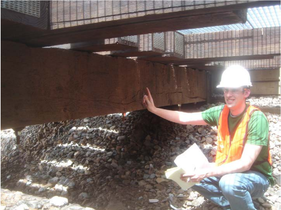
Figure C.2 Close up of crack in stringer 1, span 1. Coded 2A
