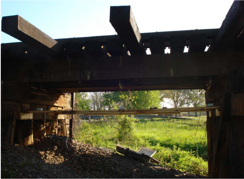
Figure B.3 String Potentiometers hung below bridge – Glidden Sub 69.11
