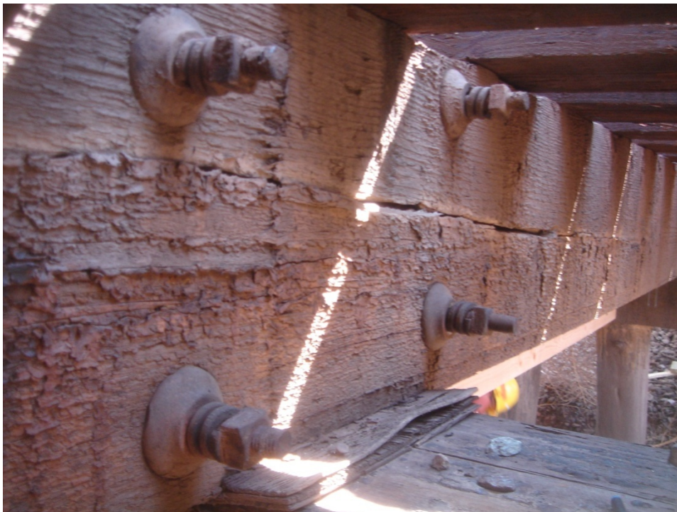
Figure C.14 Split at mid depth between lateral tie rods at Pier 2, stringer 4, spans 1 and 2.
