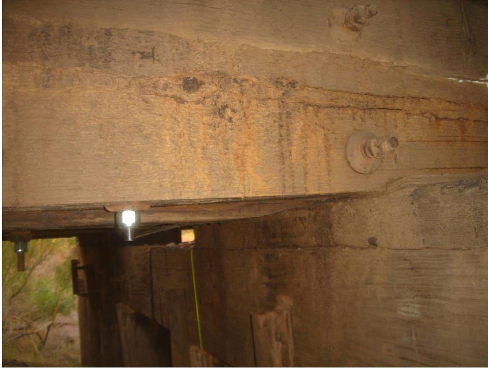
Figure C.25 View showing compressed Stringer 3, Span 1
