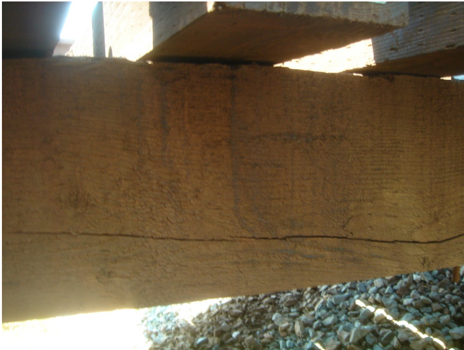
Figure C.8 Bad knots, flexural cracks - Span 1, mid span of Stringer 1.
