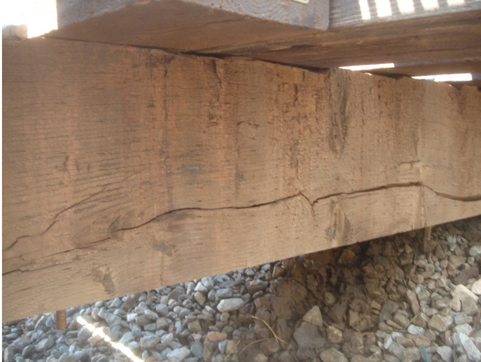
Figure C.7 Bad knots, flexural cracks - Span 1, mid span of Stringer 1.
