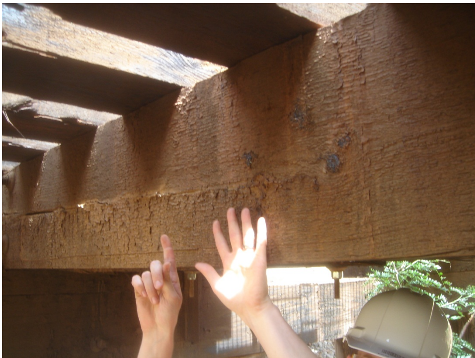
Figure C.12 Shear Crack in Stringer 4, Span 2. Coded 4A
