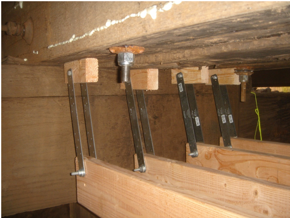
Figure C.26 View of showing compressed Stringer 3, Span 2
