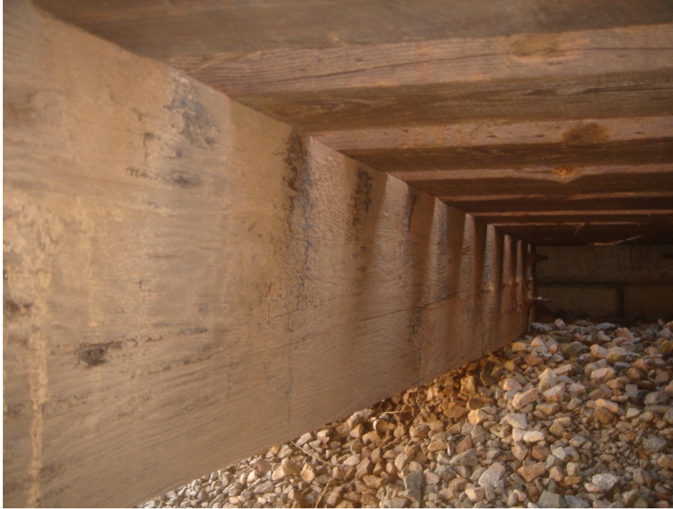
Figure C.21 Stringer 5, Span 1 – Horizontal Crack
