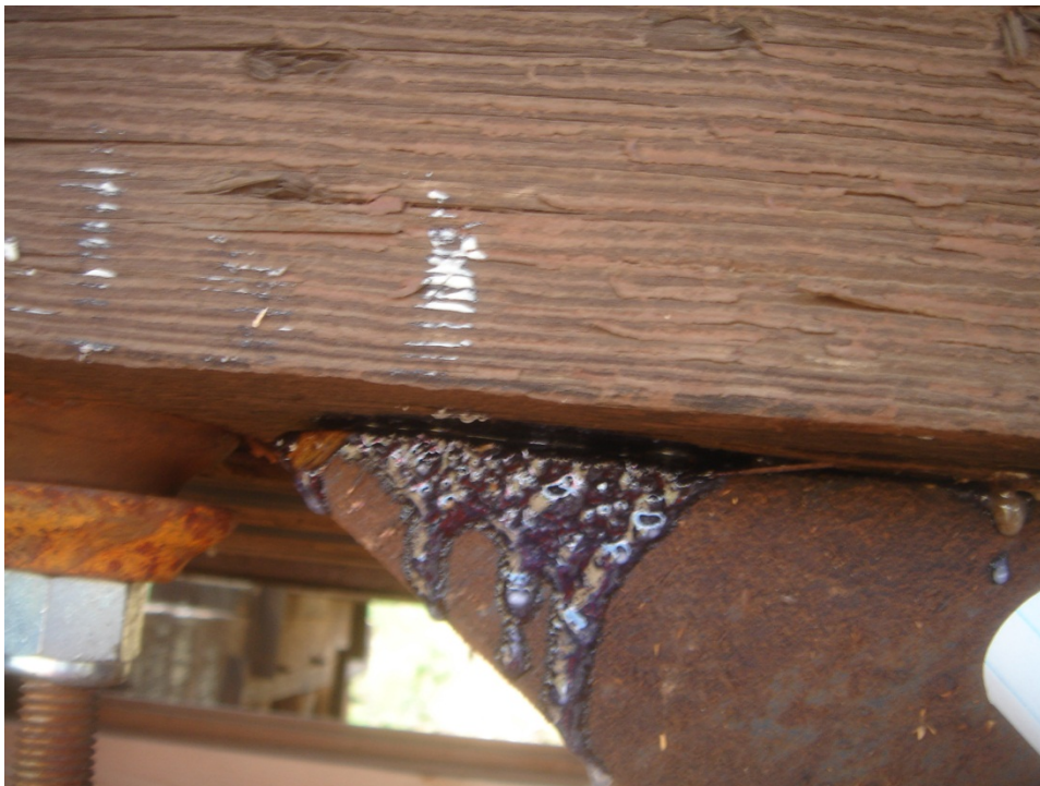
Figure C.42 Cardboard expediently nailed to bottom of beam to stop flow of epoxy through hole.
