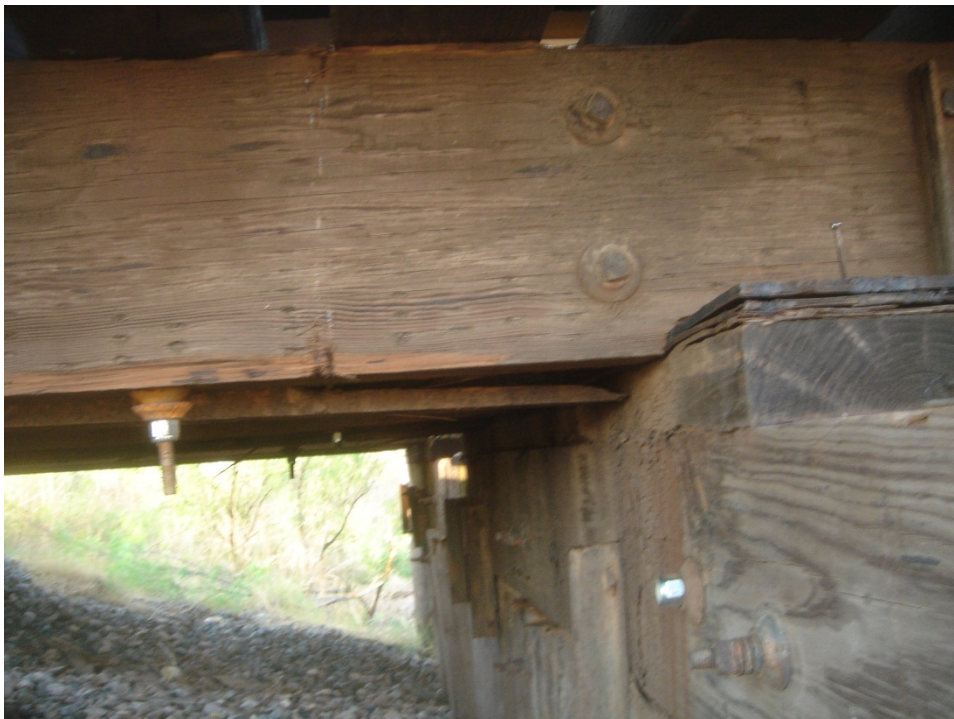
Figure C.54 Shimmed chord with stringer hanging below pier cap.
