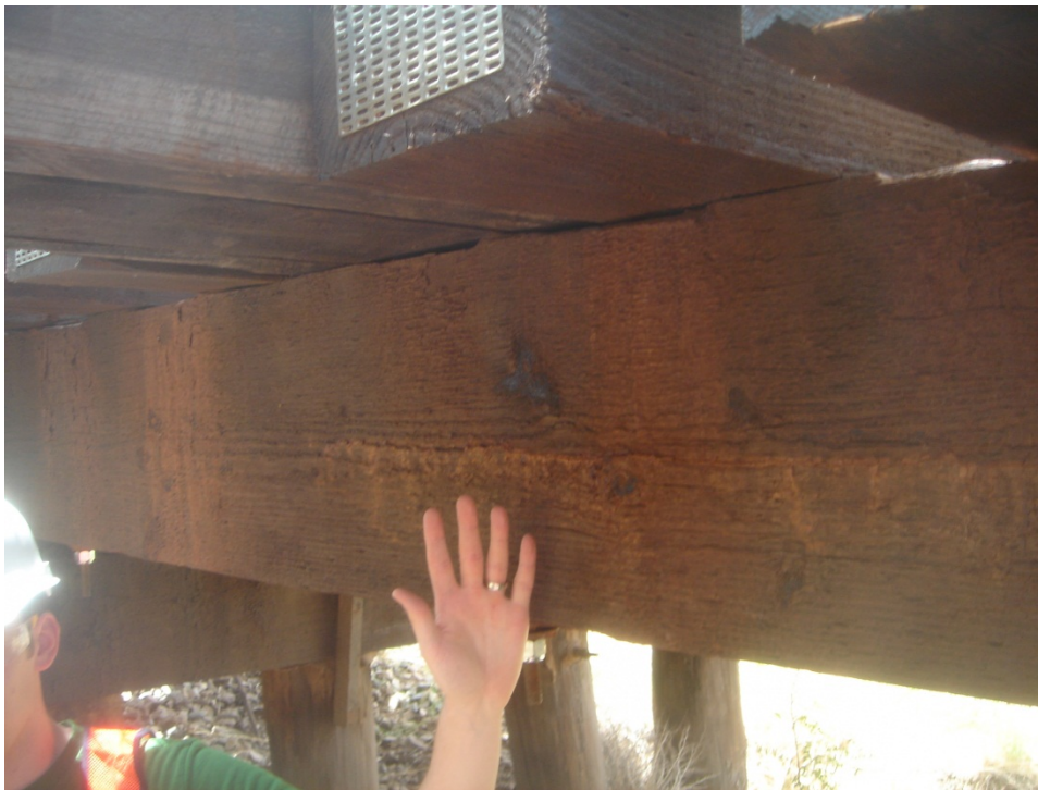
Figure C.10 Horizontal Shear Crack in Stringer 1, Span 2. Coded 4A
