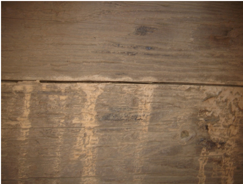
Figure C.18 Stringer 5, Span 1 – close up of horizontal crack.
