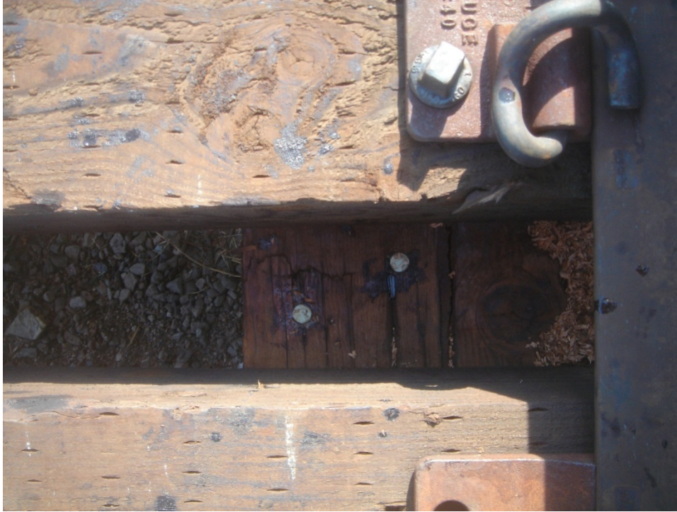
Figure C.45 Top view of spikes inserted in beams.
