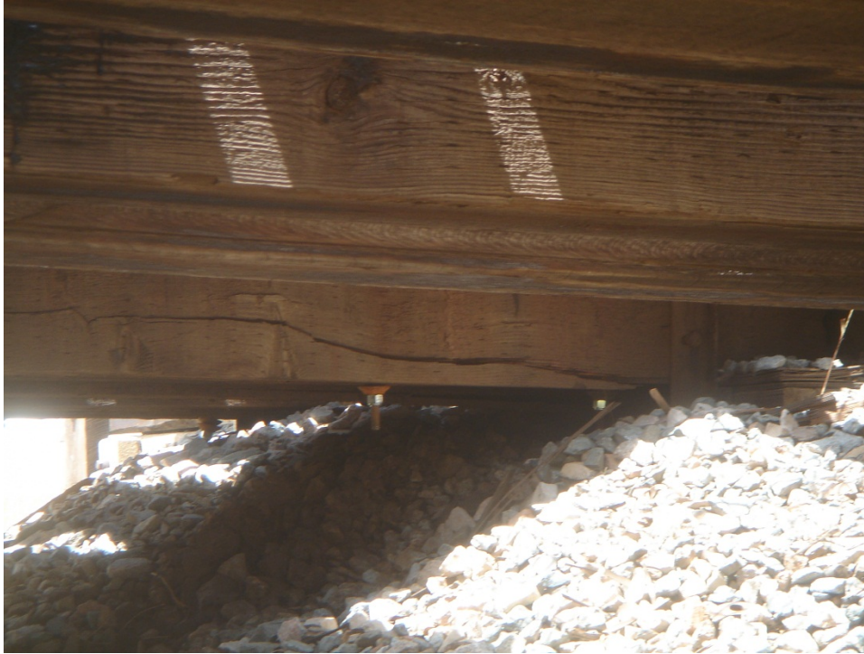
Figure C.5 Span 1, Stringer 1, badly cracked due to large knots and split near the abutment.
