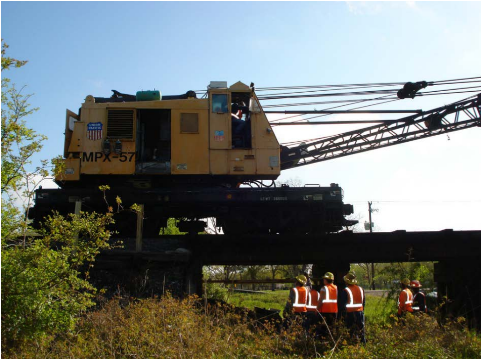
Figure B.16 Crane for loading bridge – Glidden Sub 69.11
