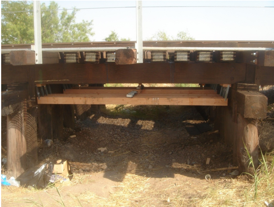
Figure C.27 Instrumentation setup for Bridge No. 2
