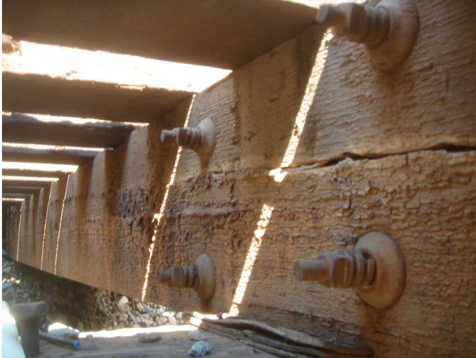
Figure C.13 Split at mid depth between lateral tie rods at Pier 2, stringer 4, spans 1 and 2.
