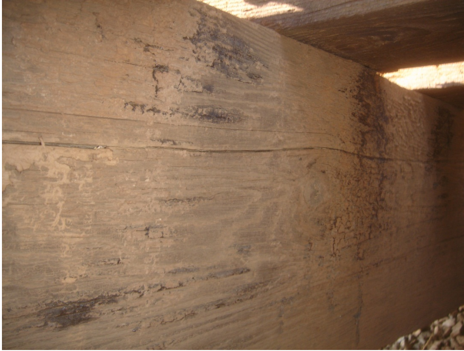
Figure C.17 Stringer 5, Span 1 – Horizontal crack looking away from the pier toward the abutment.
