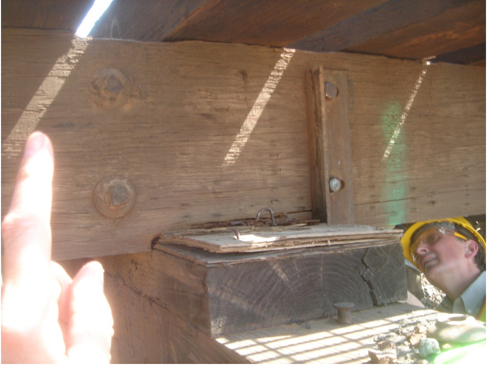
Figure C.32 Stringer 8 – Close up of damage over pier
