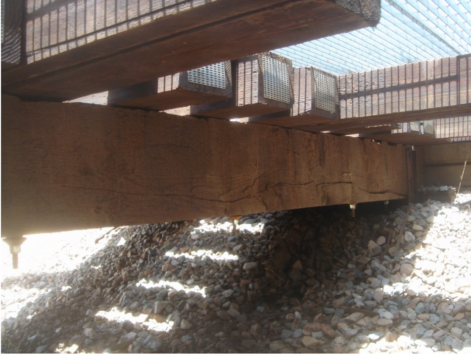
Figure C.3 Span 1, Stringer 1, badly cracked due to large knots and split near abutment.
