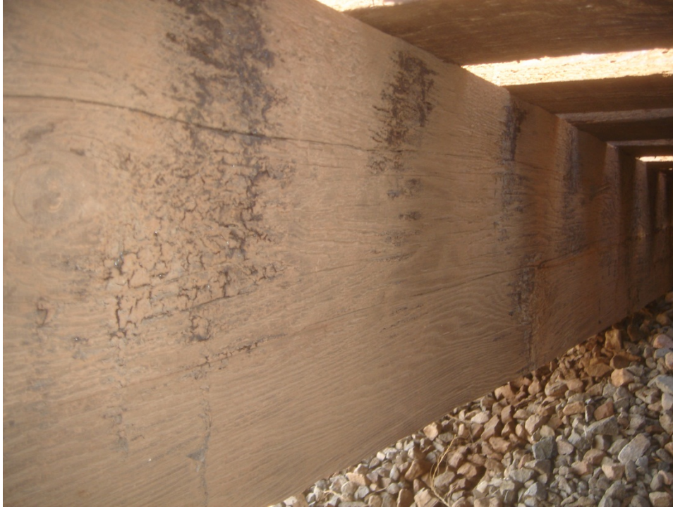
Figure C.23 Stringer 5, Span 1 – Horizontal crack near abutment
