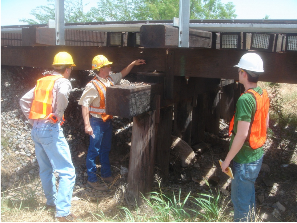
Figure C.31 Stringer 8 – Gap over pier between Span 1 and Span 2
