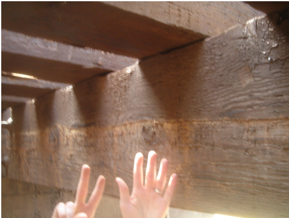
Figure C.16 Shear crack in Stringer 5, Span 2
