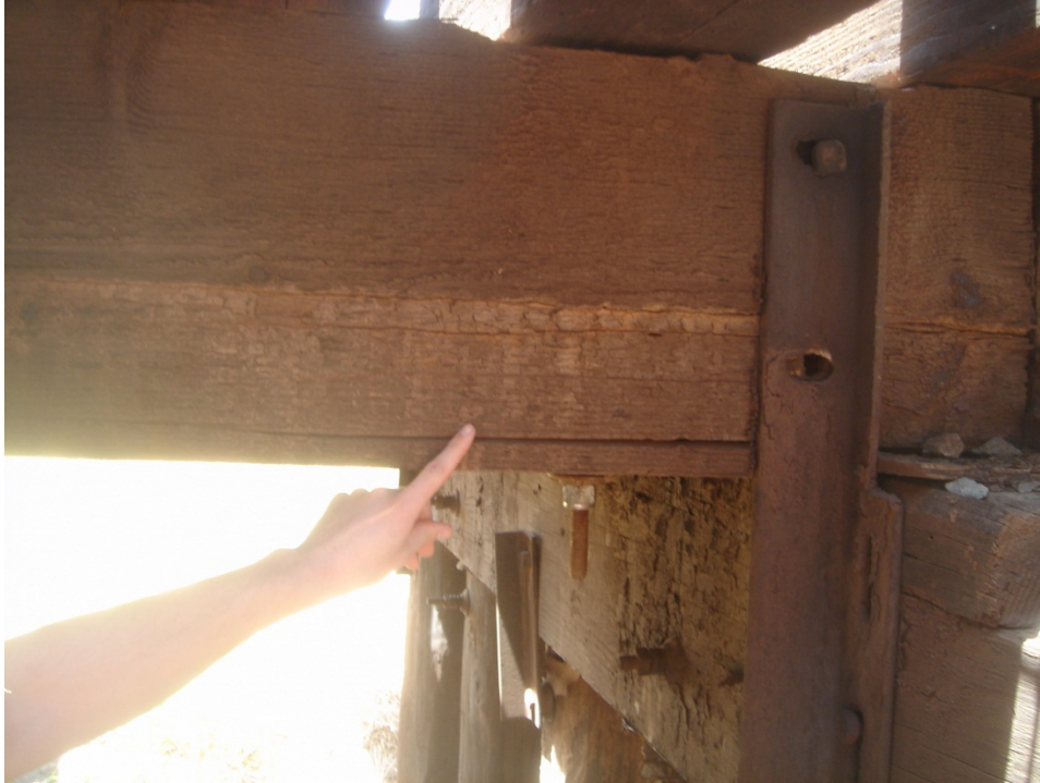
Figure C.9 Stringer 1, Span 2 - split in bottom of beam emanating from right end, notched bottom of beam at shimmed cap.
