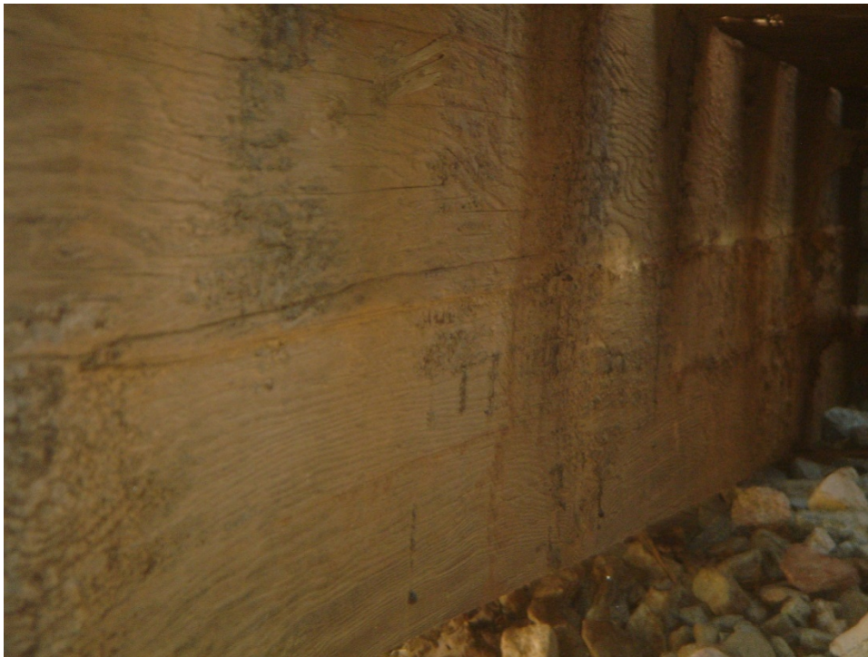
Figure C.22 Stringer 5, Span 1 – Horizontal Crack by abutment
