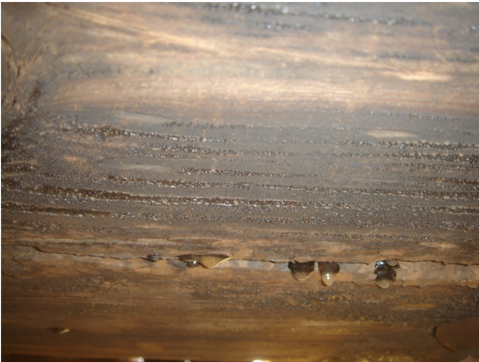
Figure C.40 Epoxy pushed out of cracks in beams
