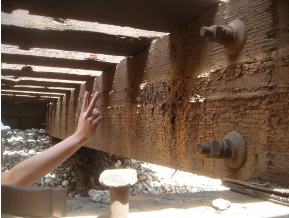
Figure C.11 Nathan pointing (2 fingers) to shear crack in stringer 4 , Span 1. Coded 4A
