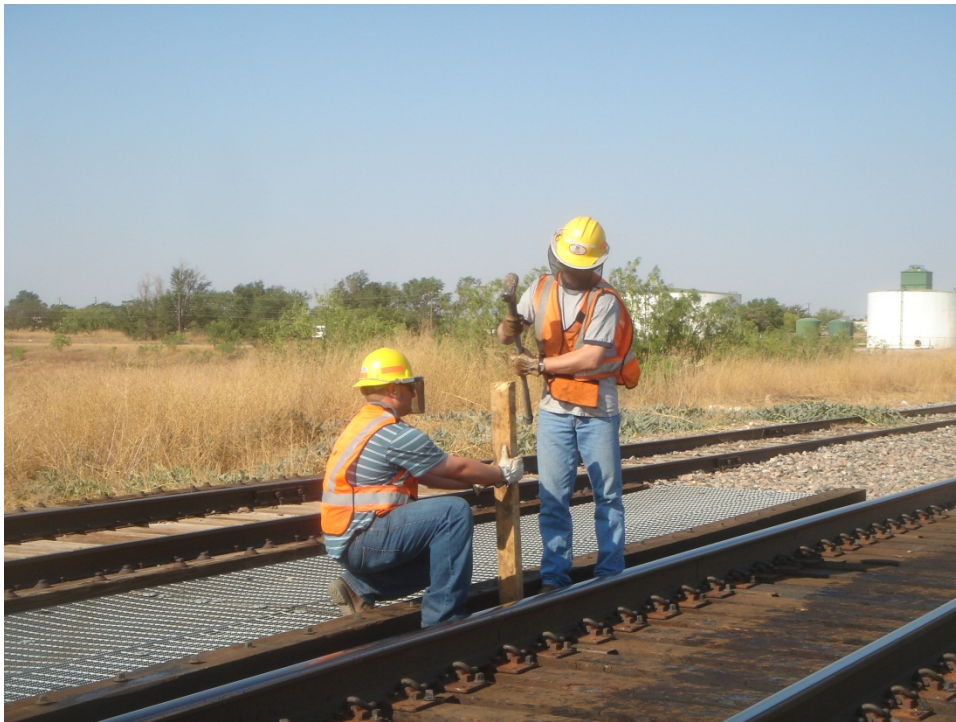
Figure C.46 Spikes inserted by UPR employees.
