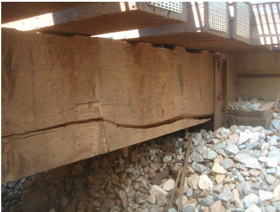
Figure C.6 Bad knots, flexural cracks - Span 1, abutment end of Stringer 1.
