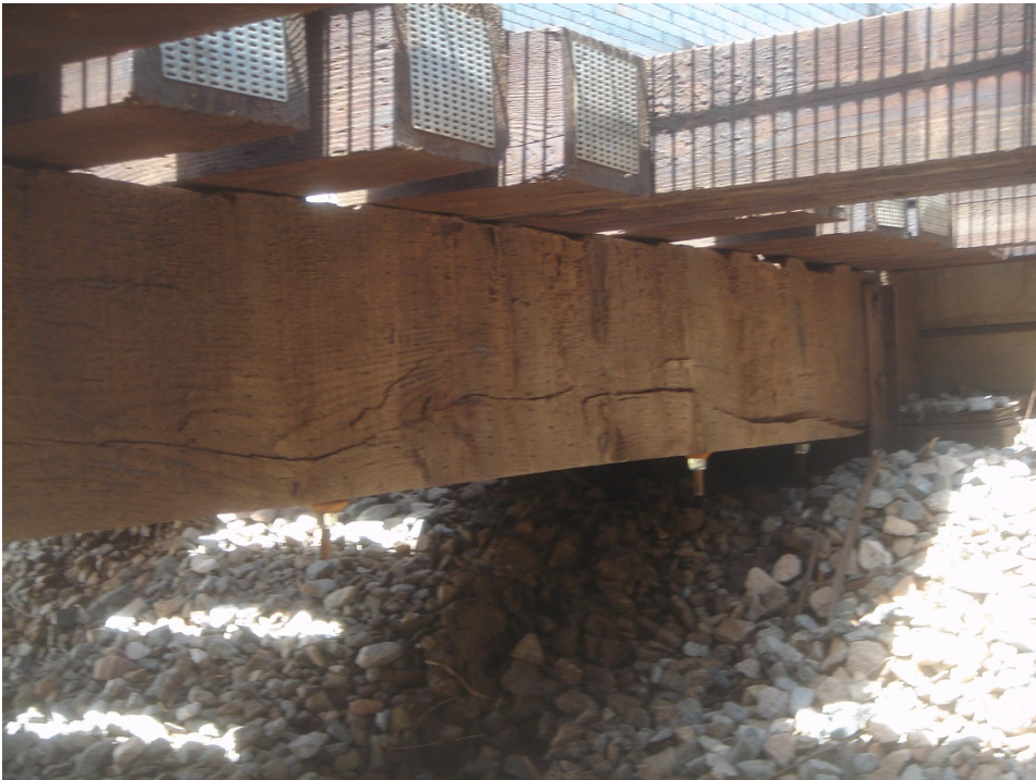
Figure C.4 Span 1, Stringer 1, badly cracked due to large knots and split near the abutment.
