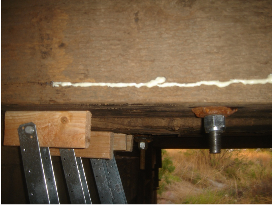
Figure C.37 Spray foam used to fill cracks
