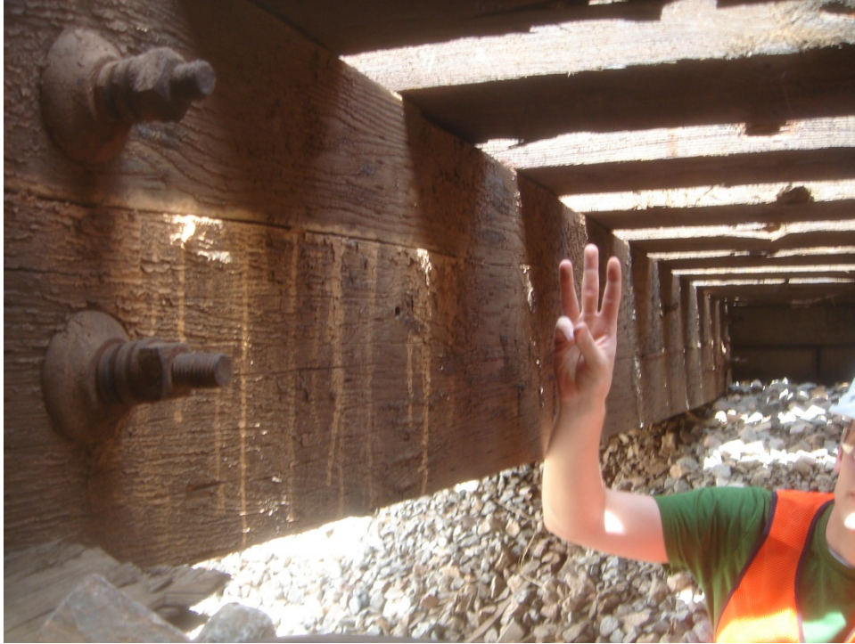
Figure C.15 Stringer 5, Span 1 - Split between tie rods at interior pier. Coded 4A
