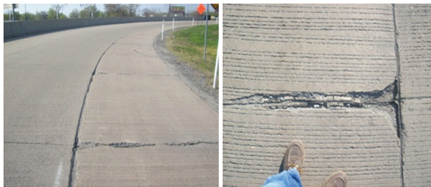
Figure 3.1 Photograph of field observation showing damage in pavement joints
