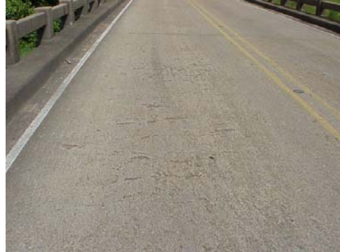
Figure 3.3.6. Cracking due to thermal expansion and contraction.
