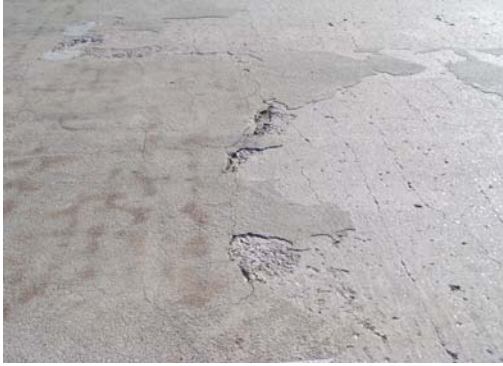
Figure 3.3.30. Scaling and discoloration of bridge deck due to underlying corrosion.
