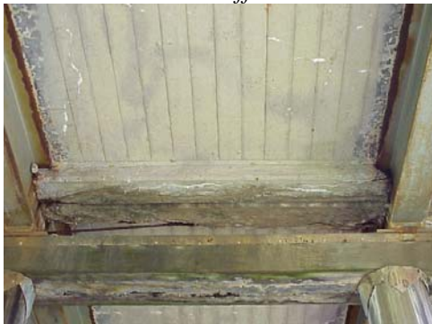
Figure 3.3.4. Corrosion of reinforcement.
