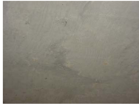
Figure 3.3.12. Underside of bridge deck showing initial signs of delamination.
