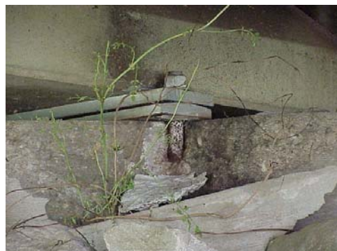
Figure 3.3.9. Loss of concrete mass.
