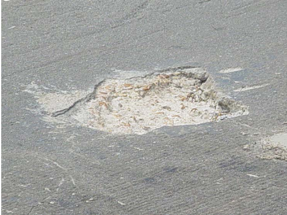
Figure 4.3 Spalling of repair material from parent concrete
