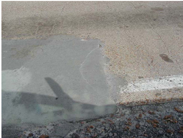
Figure 4.2 A case study of failure in repair material due to the size of repaired area.
