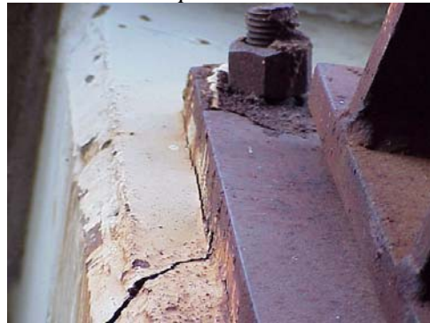
Figure 3.3.7. Cracking due to corrosion.
