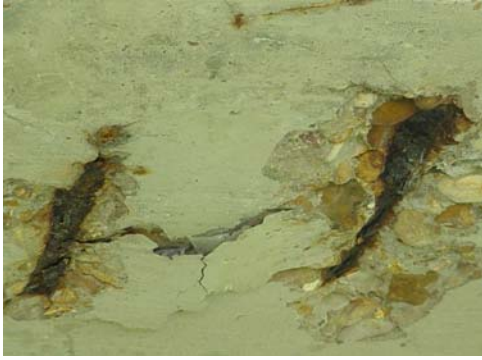
Figure 3.3.2. Loss of concrete mass due to corrosion.
