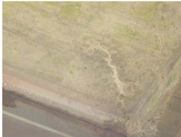
Figure 3.1.15 Shear Crack observed in a bridge deck in MDOT District VI.
