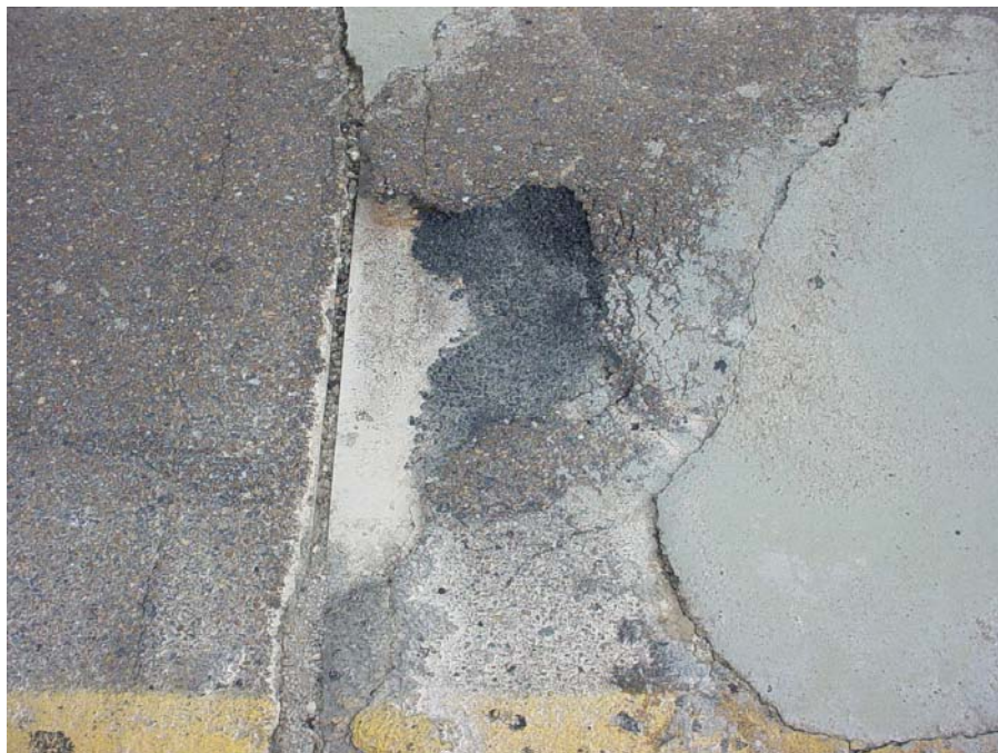
Figure 4.5 Abrasion of repair materials
