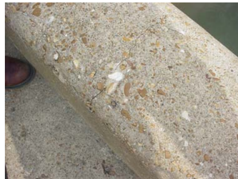
Figure 3.3.15. Pop-outs on bridge rail.
