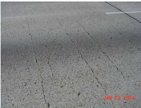
Figure 3.3.40. Cracking due to Underlying corrosion.
