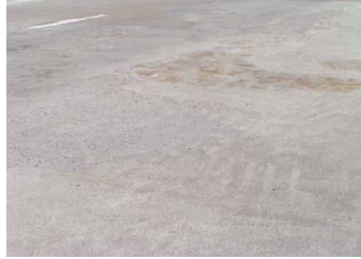
Figure 3.3.32. Discoloration of bridge deck indicating corrosion of steel reinforcement.
