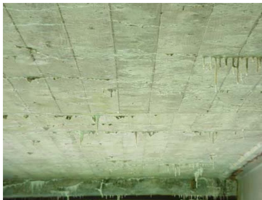
Figure 3.1.9 Efflorescence observed in MDOT District I.
