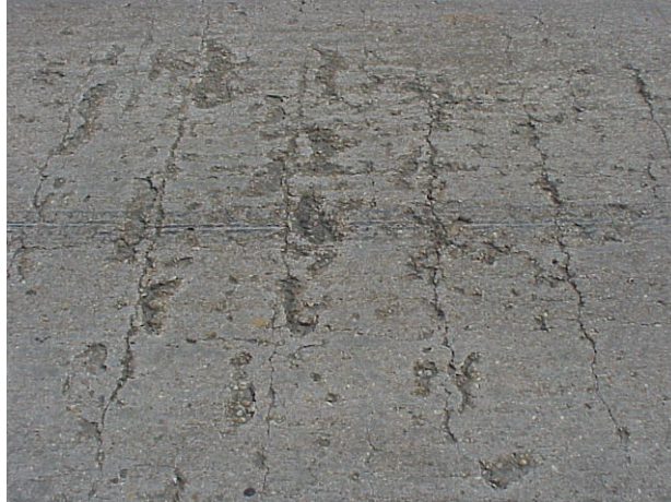
Figure 3.1.1 Non-structural cracking due to thermal expansion and contraction observed in MDOT District I.
