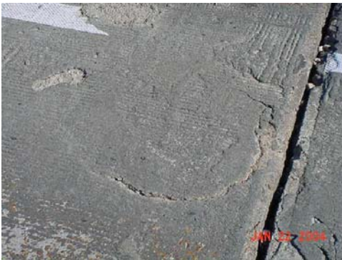
Figure 3.3.35. Scale and joint failure.
