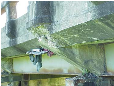
Figure 3.3.3. Loss of concrete mass due to efflorescence.
