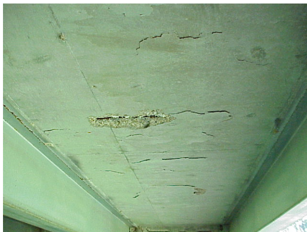
Figure 3.1.4 Delamination and spall (due to corrosion) observed in MDOT District I.
