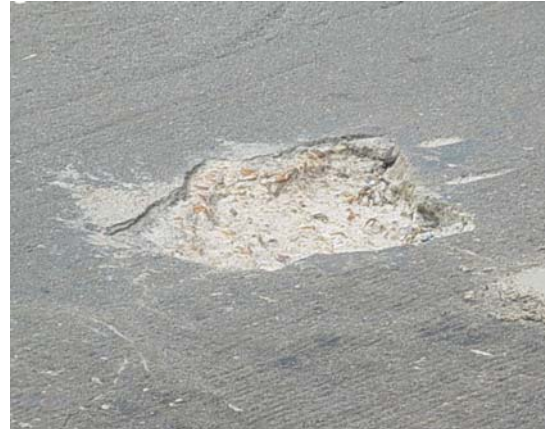
Figure 3.1.7. Spall observed in MDOT District II.
