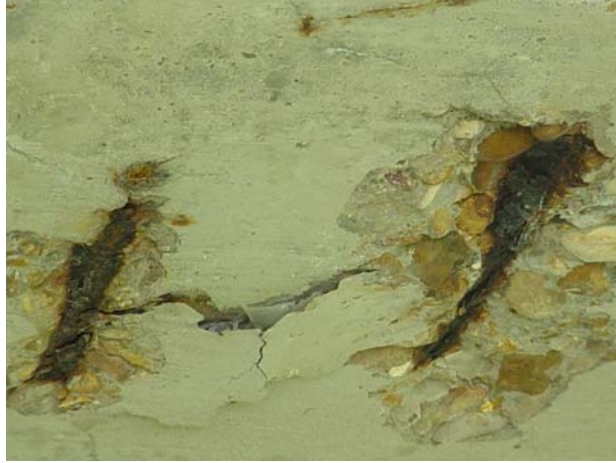
Figure 3.2.12 Example of corrosion of reinforcement in a bridge deck in District 1.
