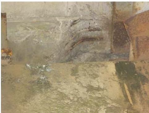
Figure 3.3.47. Discoloration and staining indicating corrosion.
