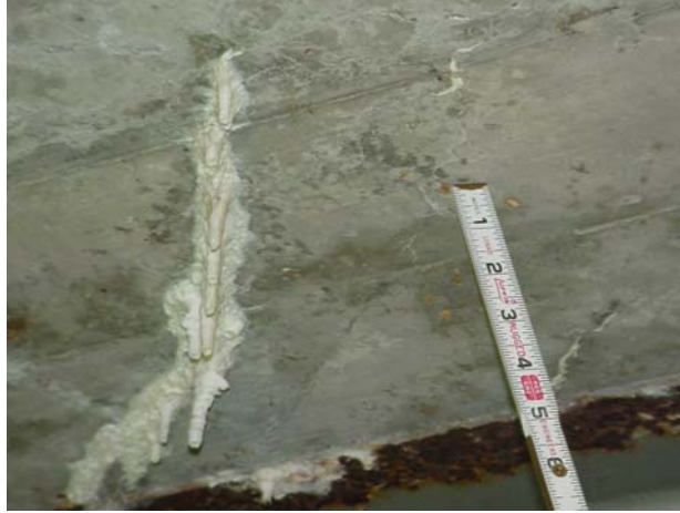
Figure 3.2.13. Example of efflorescence in District 1.
