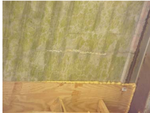
Figure 3.3.49. Leaching of Calcium Hydroxide.
