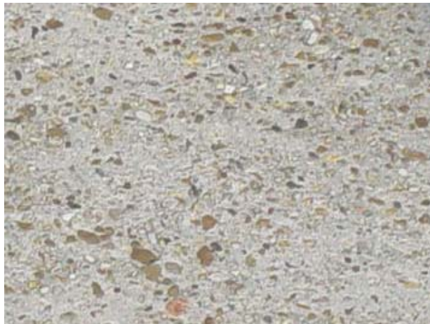
Figure 3.1.13. Wear observed in MDOT District VI.
