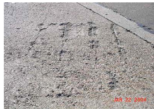
Figure 3.3.43. Severe exposure of steel reinforcement.
