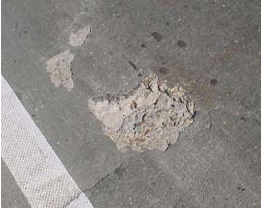
Figure 3.1.6. Spall observed in MDOT District V.
