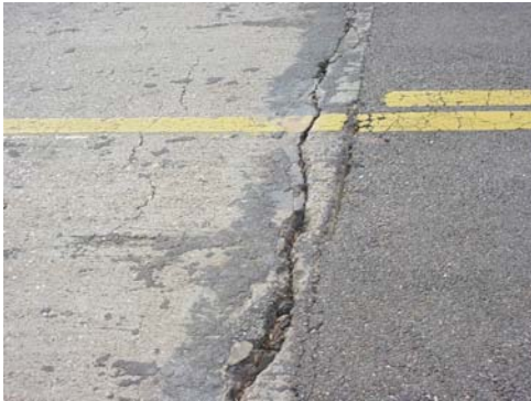
Figure 3.3.46. Severe cracking and separation of bridge deck from roadway.
