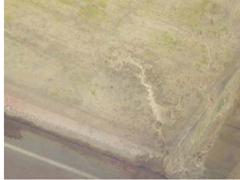
Figure 3.3.48. Structural shear crack due to overloading (under-designed case)
