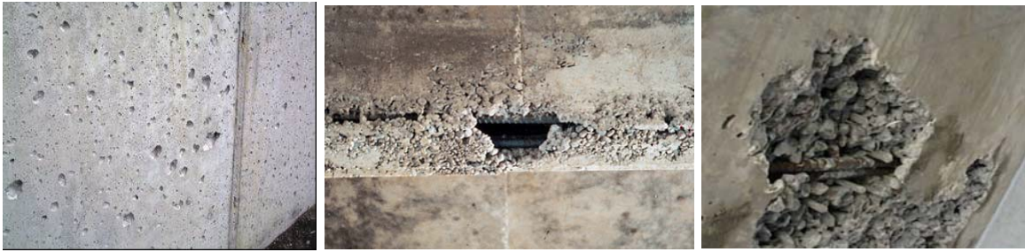
Figure 3.1.10 Examples of construction defects.
