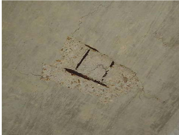
Figure 3.1.5 Non-structural cracking and loss of mass due to corrosion observed in MDOT District V.
