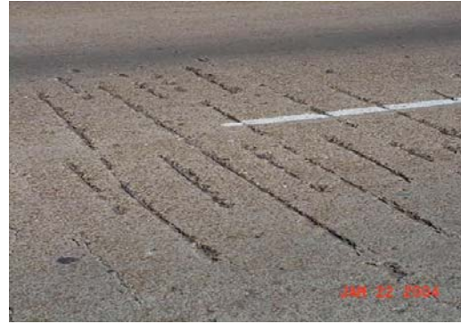
Figure 3.3.42. Exposure of steel reinforcement.
