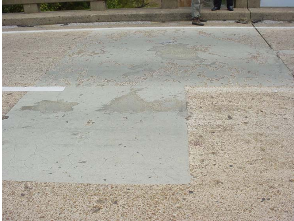
Figure 4.6 Cracking of repair materials
