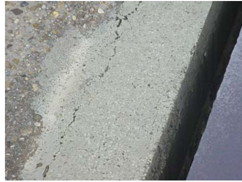
Figure 3.3.53. Cracking and separation of bridge joint repair from roadway.
