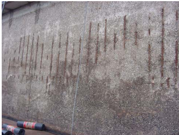
Figure 3.1.11 Example of construction defects (insufficient concrete cover).
