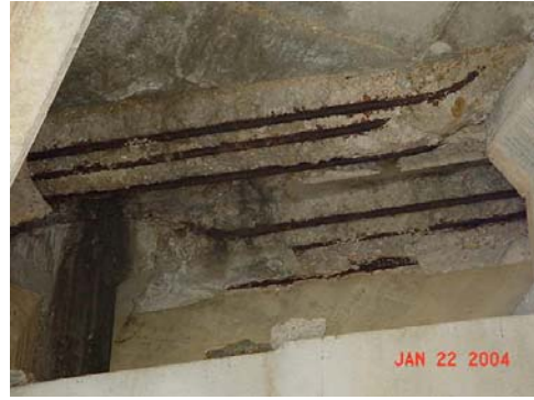
Figure 3.3.38. Severe loss of mass due to corrosion of reinforcements.
