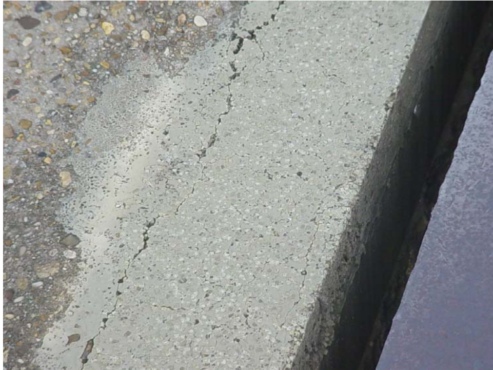
Figure 4.7 Repair of joint failure due to continuous dynamic impact of traffic
