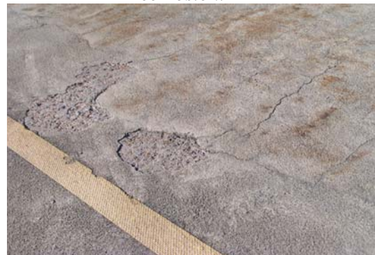
Figure 3.3.29. Spalling and discoloration of bridge deck due to underlying corrosion.
