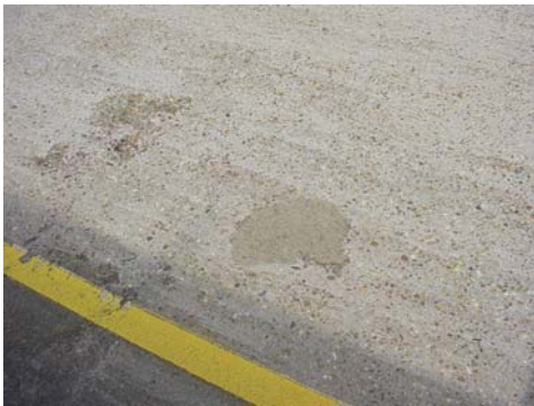
Figure 3.3.52. Light scale and spalling.
