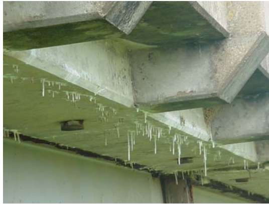
Figure 3.1.8 Efflorescence observed in MDOT District I.
