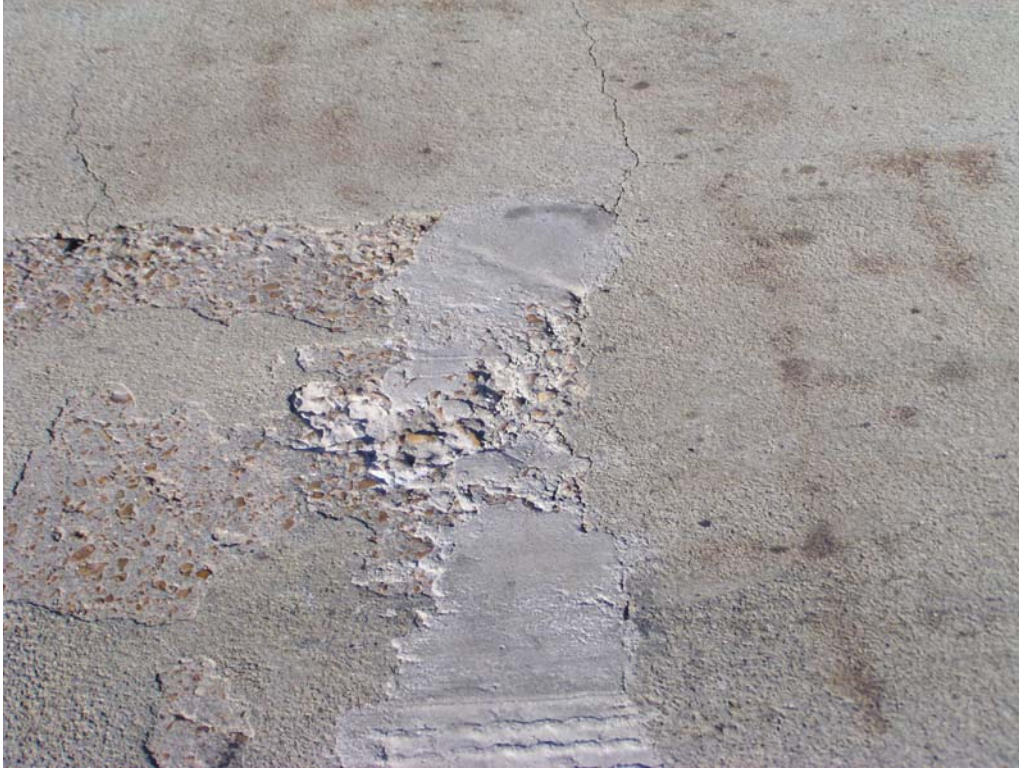
Figure 4.4 A case study showing improper use of repair technique
