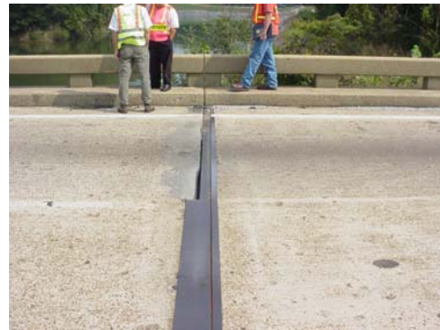
Figure 3.3.14 Joint failure due to traffic impact.
