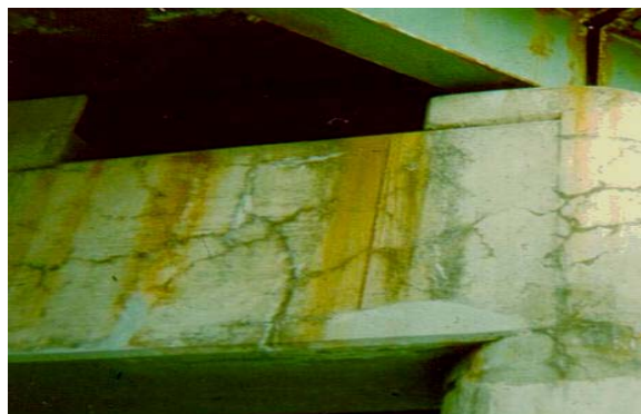
Figure 3.2.16. Result of aggregate expansion on bridge supports.
