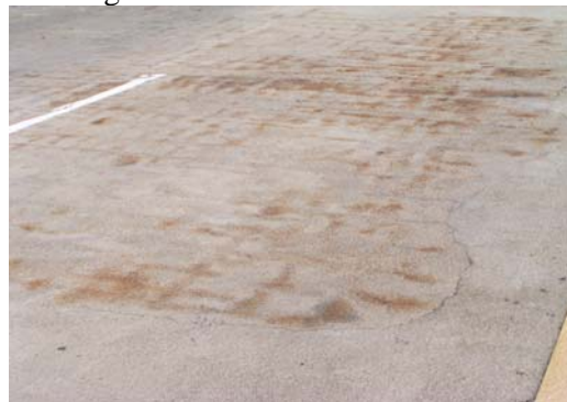
Figure 3.3.28. Discoloration of bridge deck due to underlying corrosion.
