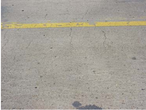
Figure 3.3.45. Cracking due to thermal expansion and contraction.
