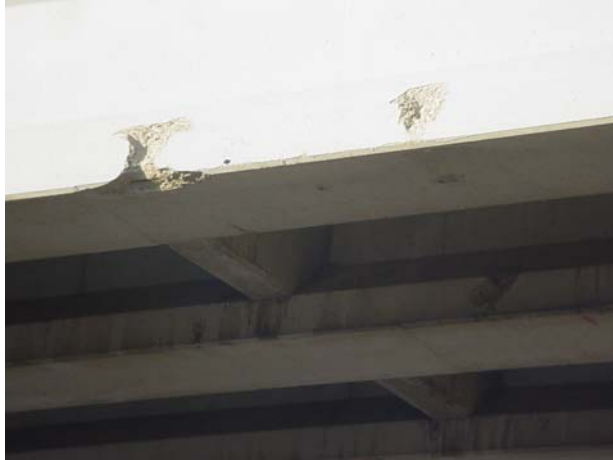
Figure 3.1.14. Collision damage observed in MDOT District VI.
