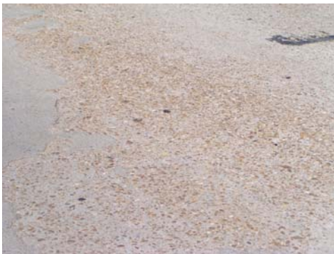
Figure 3.3.24. Wear due to traffic.
