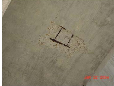
Figure 3.3.37. Loss of mass due to Corrosion of reinforcement.
