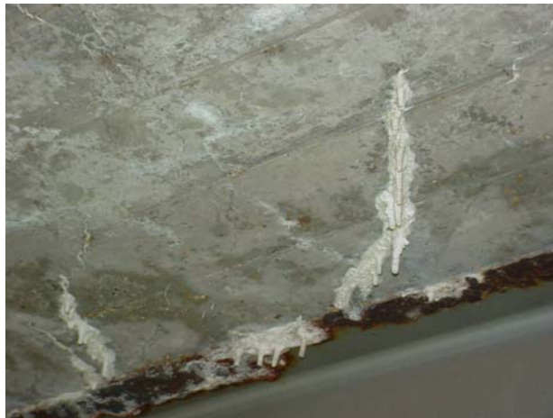
Figure 3.1.2 Non-structural cracking leading to efflorescence observed in MDOT District I.
