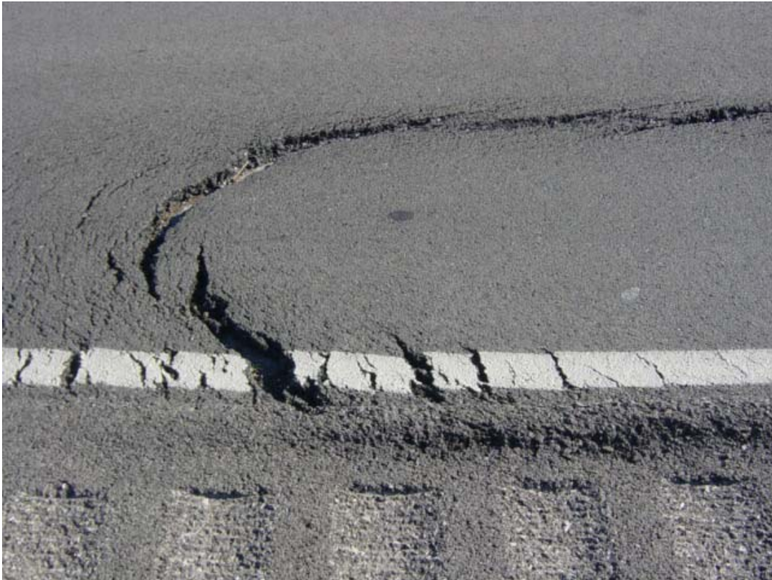
Figure 2.1 Slippage Cracking (View 1) [4]
