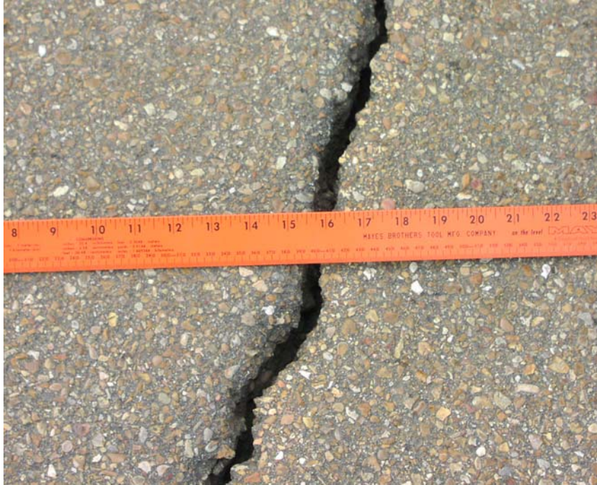
Figure 4 –Existing Reflective Crack Width
