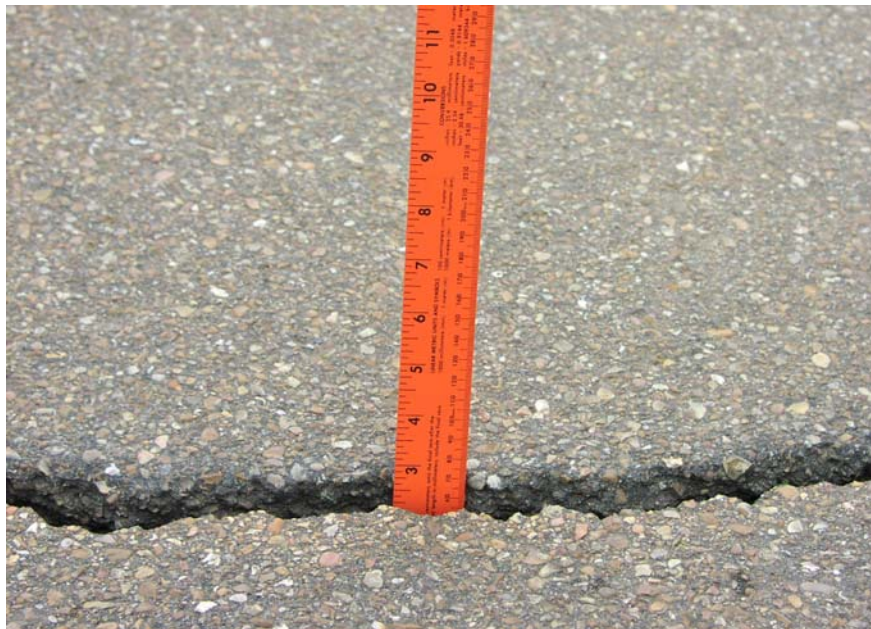
Figure 5 – Existing Reflective Crack Depth
