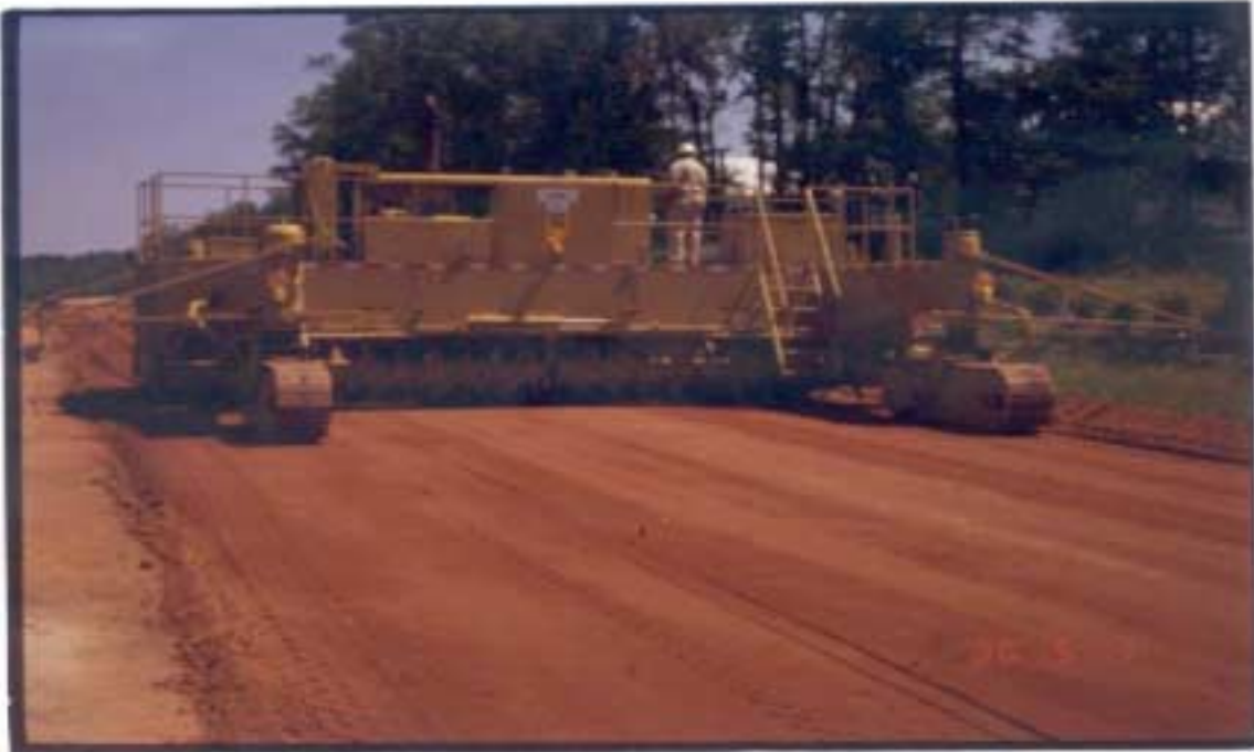
Figure 44. Use of Autograde Trimmer to Control Extent of Surface Undulations in the Base Layer (Photo courtesy of Halsted)
