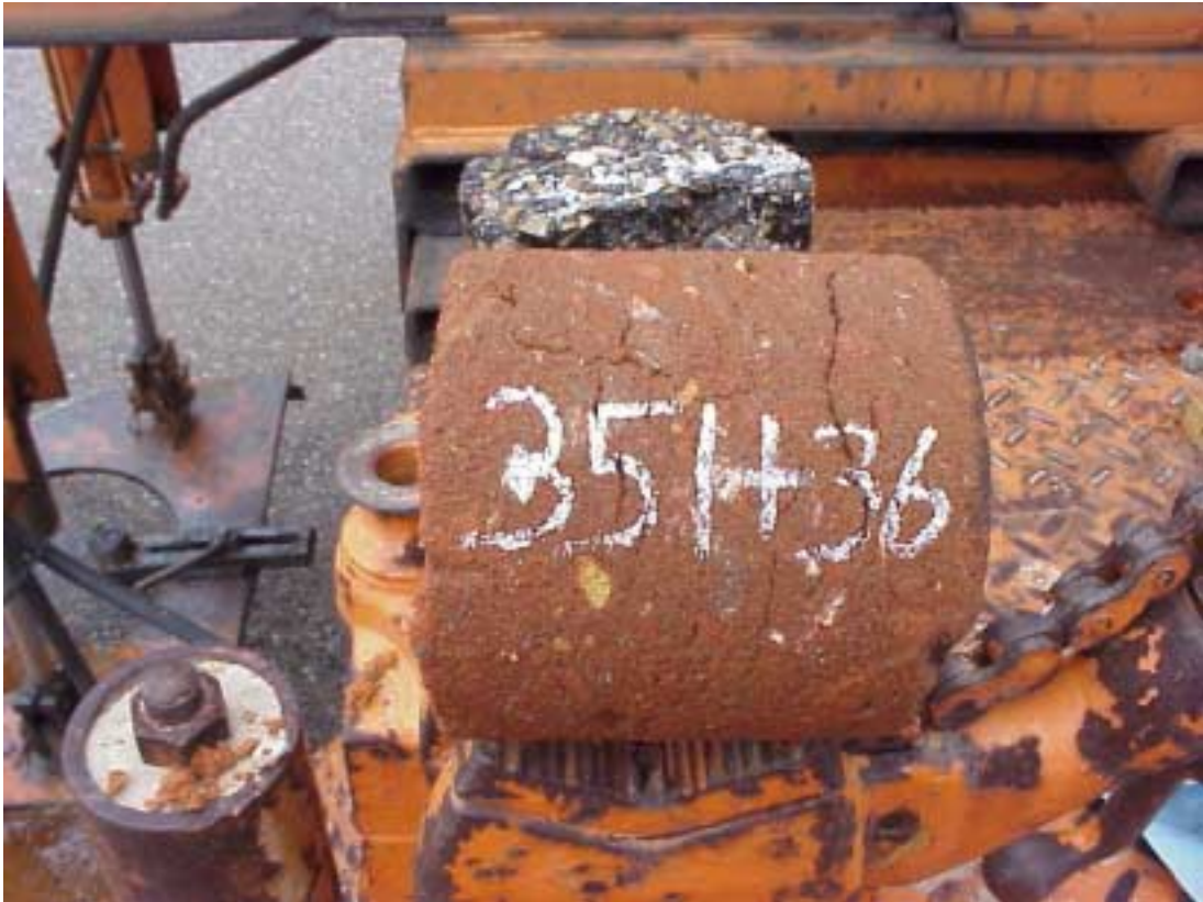
Figure 45. Cracking in LFA Base Layer Due to Inadequate In-Situ Base Layer Thickness
