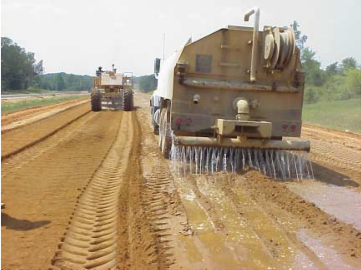
Figure 37. Current Gravity Feed Distribution Truck Method Used for Placement of Water Across the Roadbed
