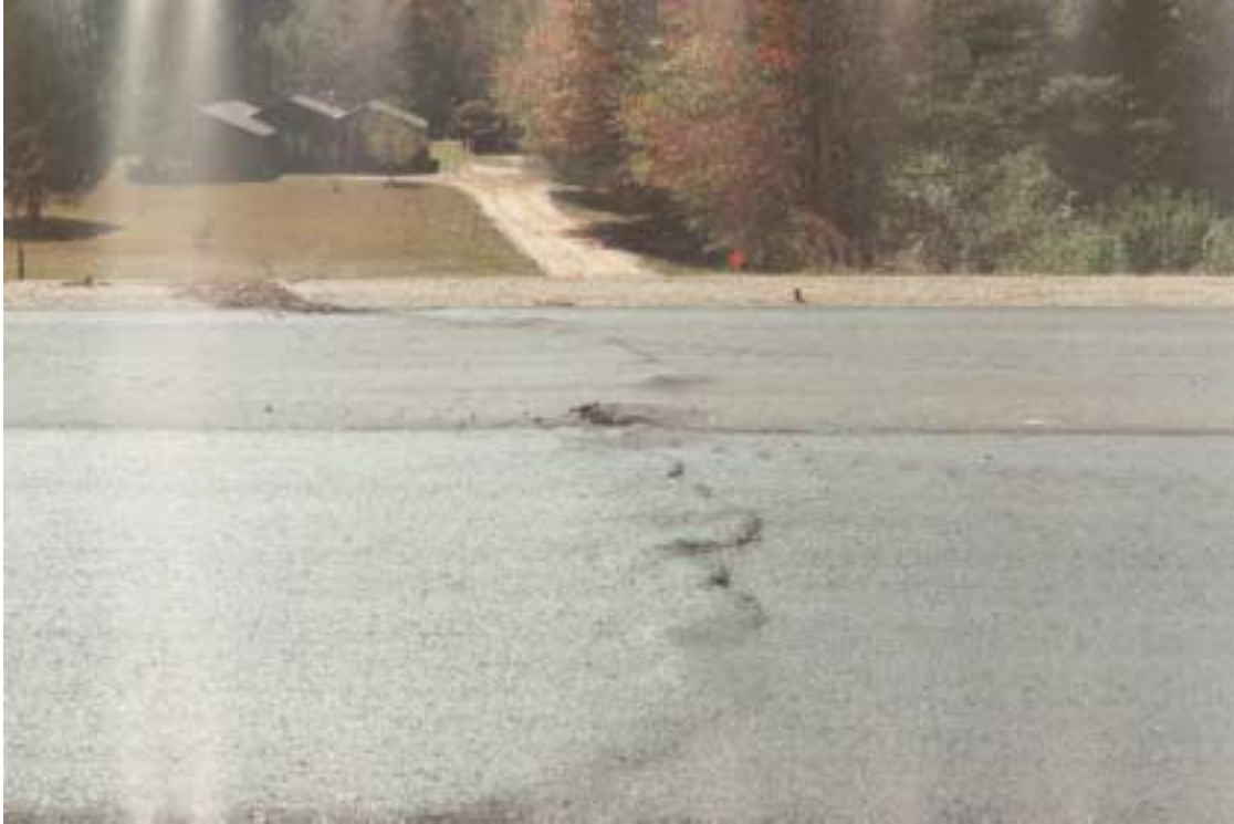
Figure 26. Surface Deformation Associated with a Blow-Up On U.S. 84 in Wayne County
