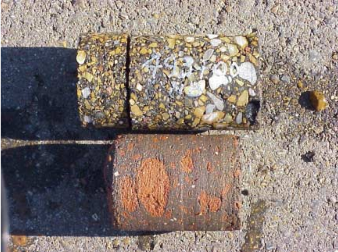
Figure 40. Clod of Unmixed Soil Within the LFA Base Layer Due to Inadequate Field Mixing
