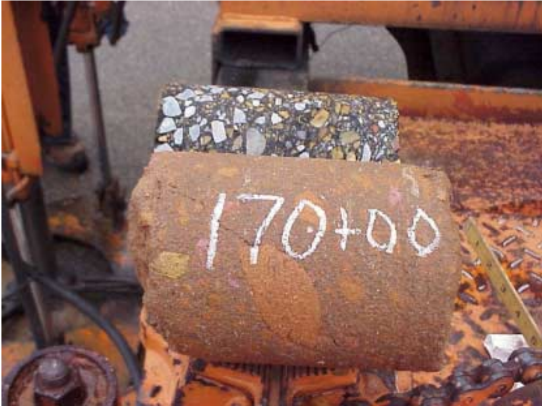
Figure 41. Cracking of LFA Base Layer Adjacent to an Unmixed Clod
