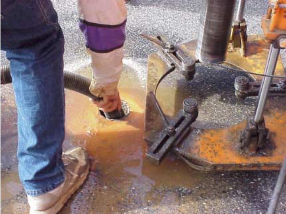
Figure 14. Shop Wet Vacuum Used to Remove Stone from Top of LFA Layer Prior to Coring
