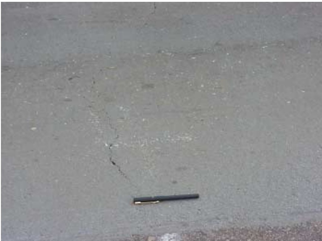
Figure 20 – Cracking in E-Krete approximately three months after application
