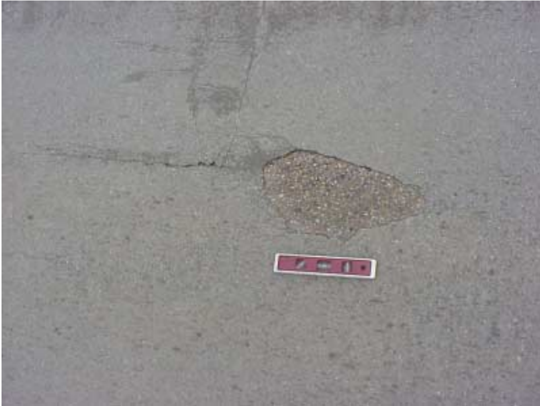
Figure 19 – Delamination in multiple application with priming area approximately one year after E-Krete application
