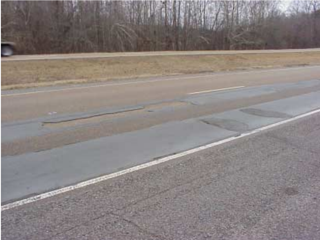
Figure 3 – Patches and delamination in Winona test site
