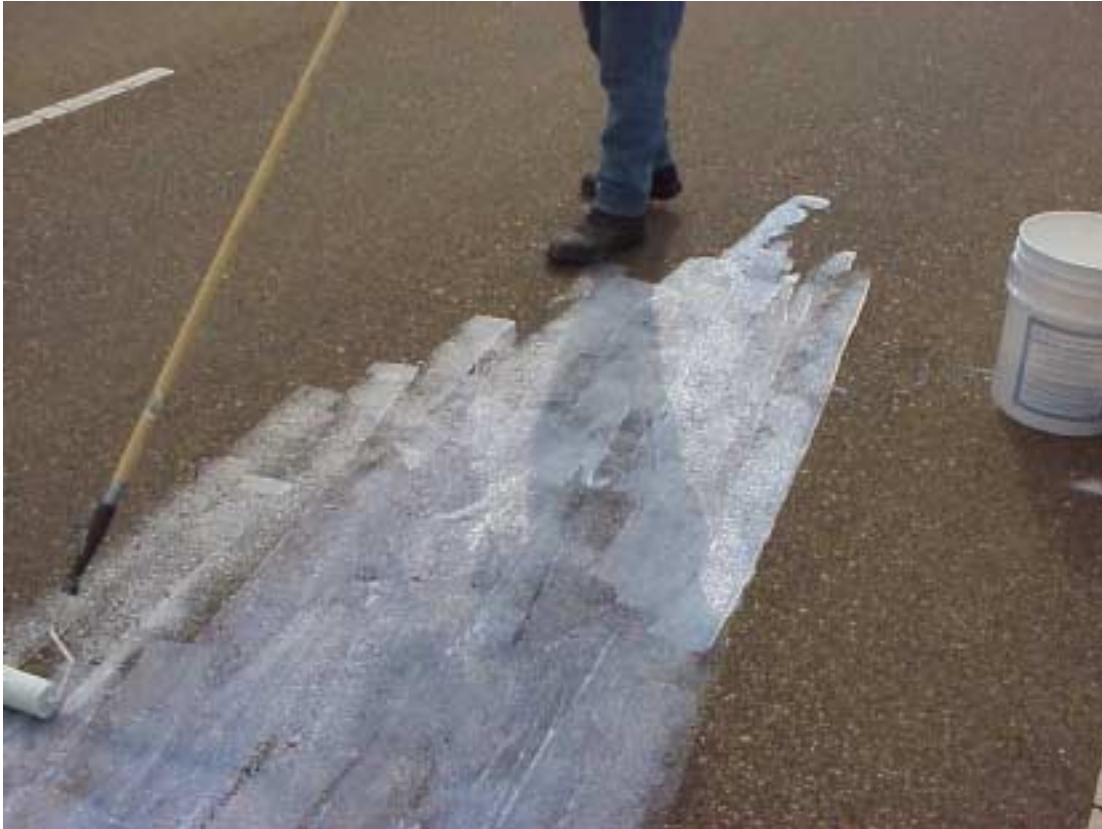
Figure 7 – Priming of the asphalt surface with the liquid solution component of E-Krete's three part system (liquid, dry mix & aggregate)
