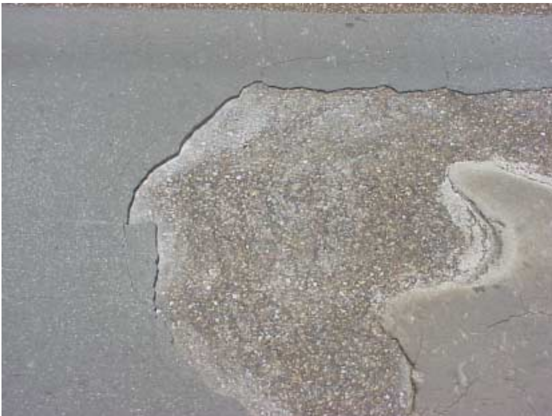
Figure 4 – Close-up of delaminated area
