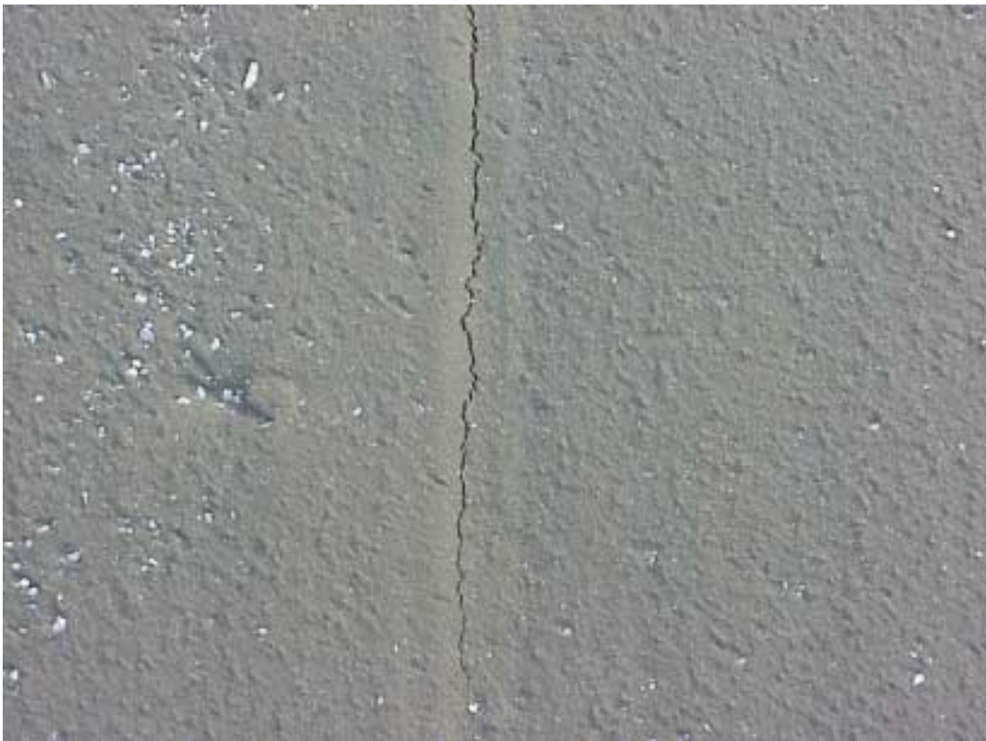
Figure 9 – Transverse crack at a screed stoppage during the previous days pour
