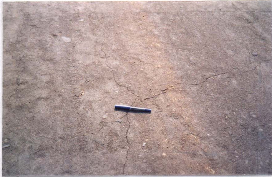
Figure B4 Transverse and longitudinal cracks in section 2 (precracked), nineteenth day.
