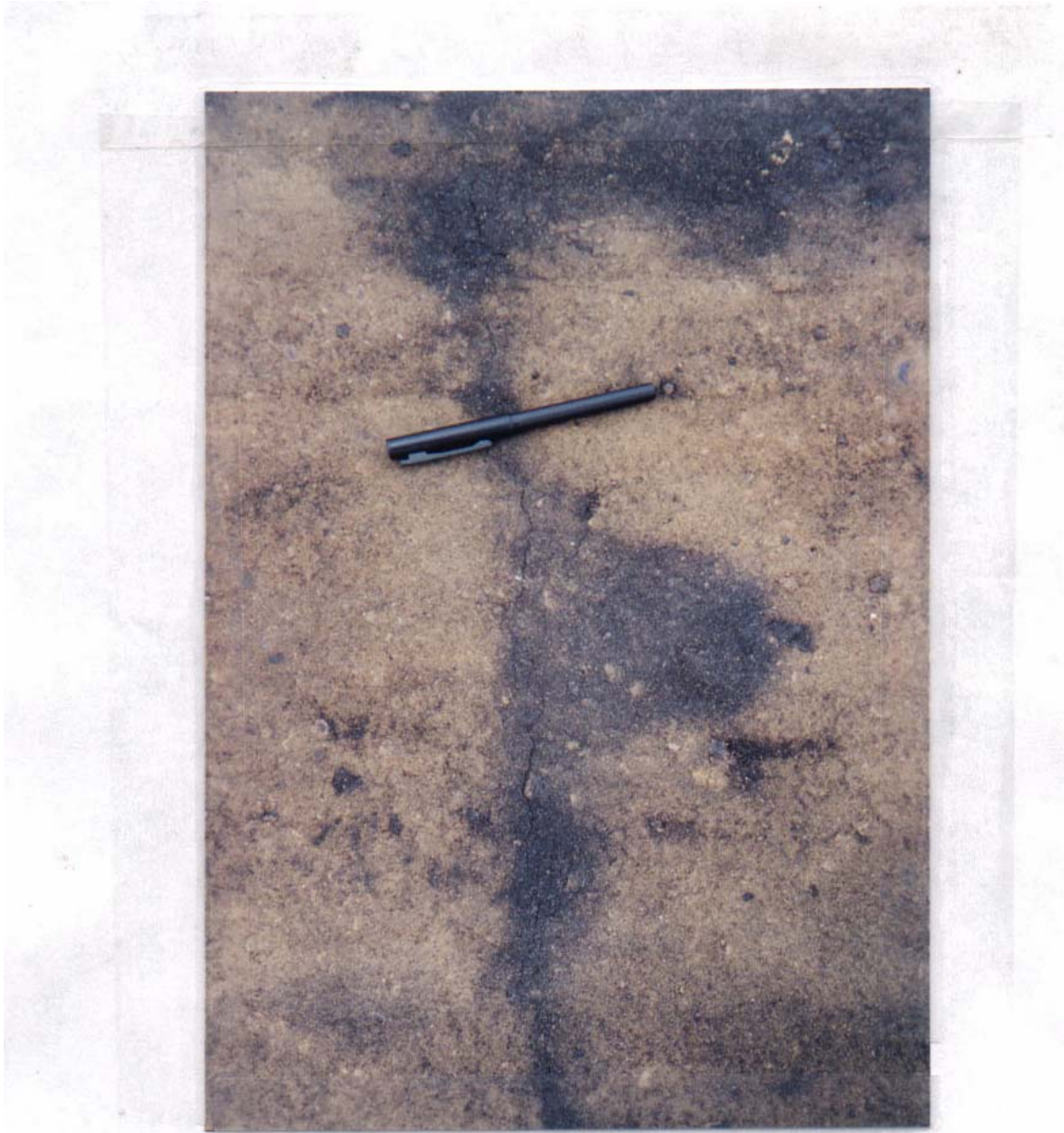
Figure B3 Transverse crack along a precut groove, section 1B, seventh day.
