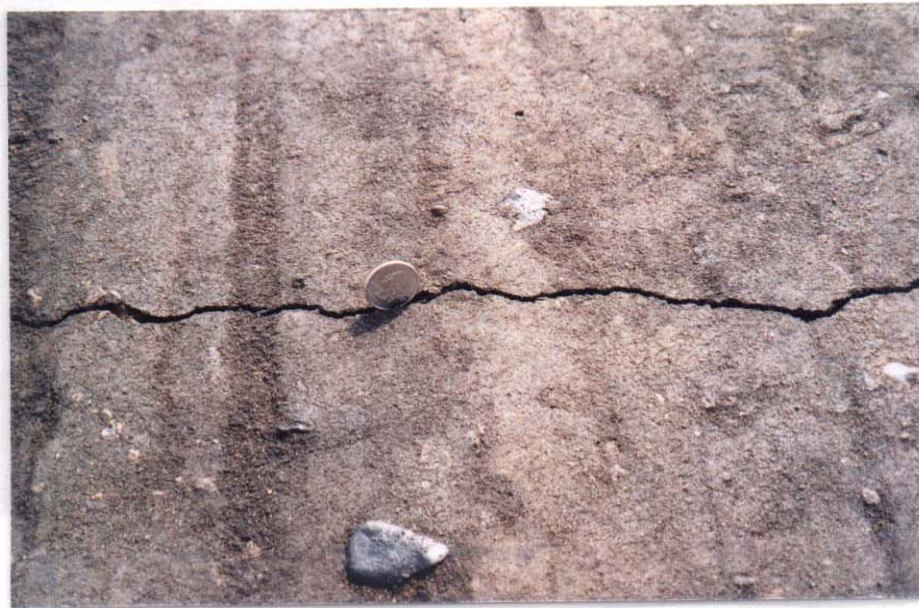
Figure B5 High severity longitudinal crack in section 4, cement – fly ash, 221 + 50, nineteenth day.
