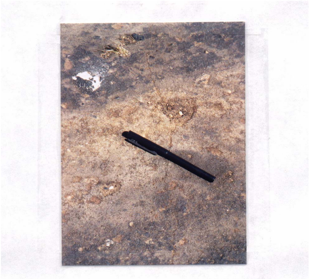
Figure B9. Fine crack in lime – fly ash section, section 6 (alternate), twenty eight days.
