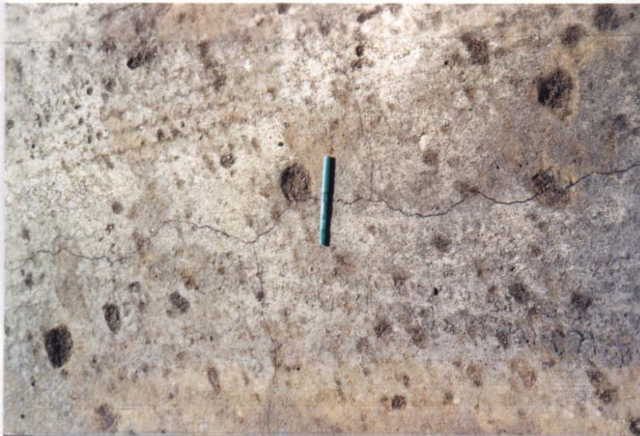
Figure 4.25 Typical crack in lime – fly ash section, 189 + 50, approximately twentieth day.
