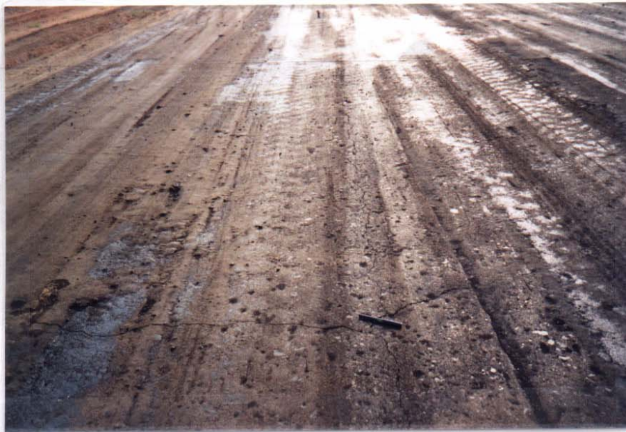
Figure B2. Medium severity crack in section 1A, control cement, nineteen days.
