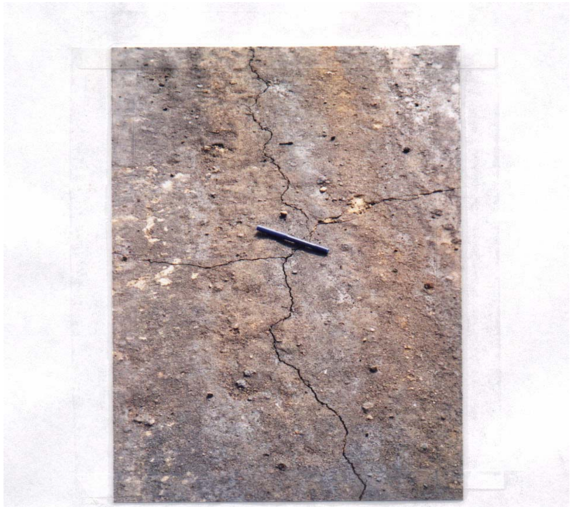
Figure B6. Medium severity crack in section 5, lime – GGBFS, nineteenth day. Curing compound completely vanished.
