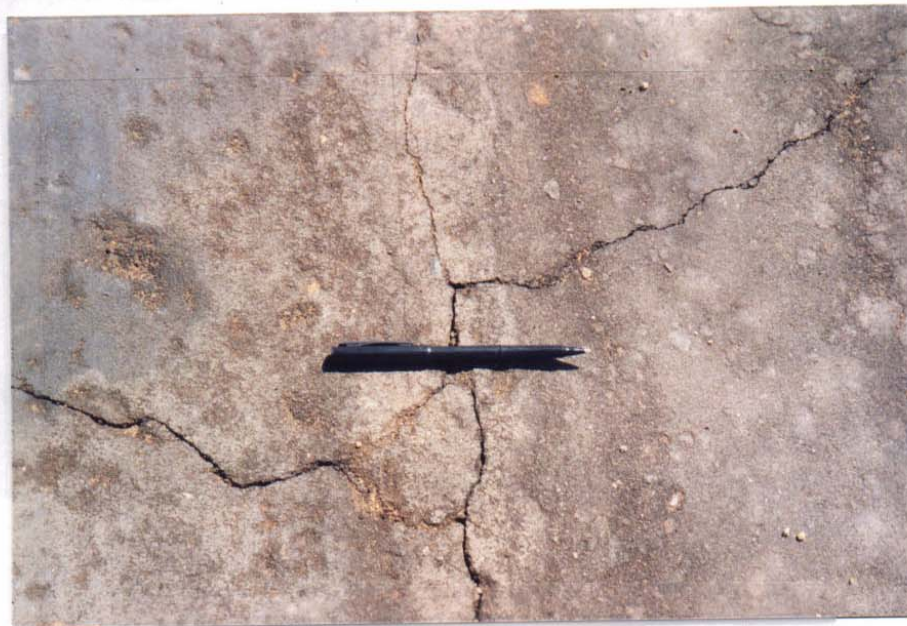
Figure 4.23 High severity cracks in section 4, cement-fly ash, twenty-eight day.
