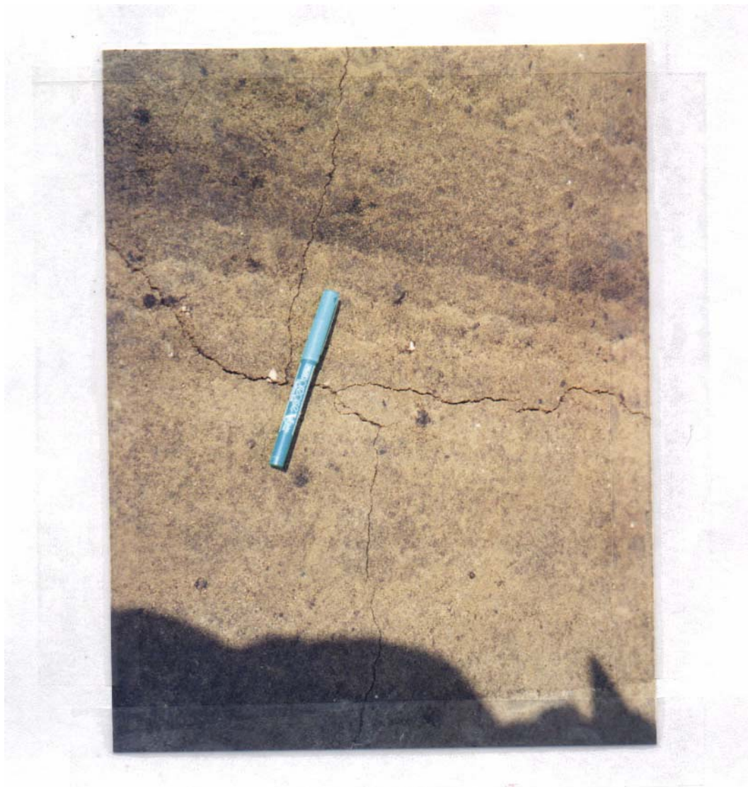
Figure B7. Meandering cracks in lime – fly ash section, 14 days.
