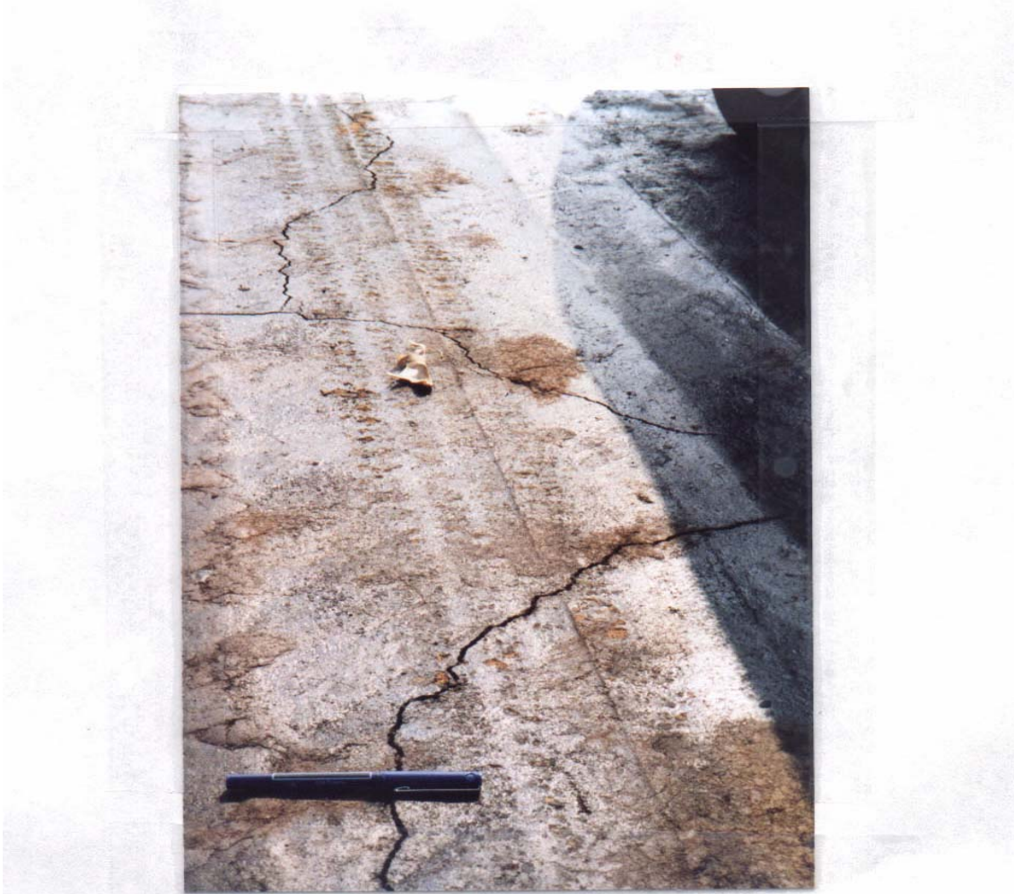
Figure B8. High severity cracks in lime – fly ash section, 241 + 50, nineteen days.
