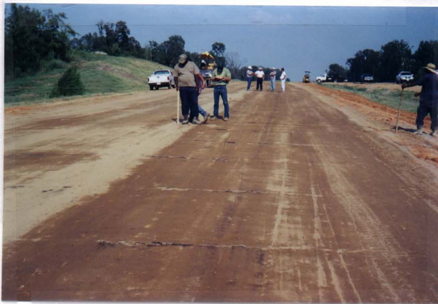
Figure 4.14 Visible precut joints after final grading and compaction.
