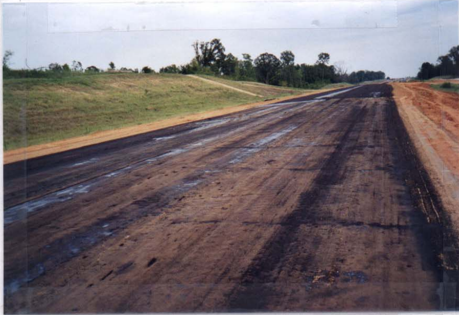
Figure B1 Section 1B (precut) in the foreground and section 2 in the background. Contrast in emulsion application.
