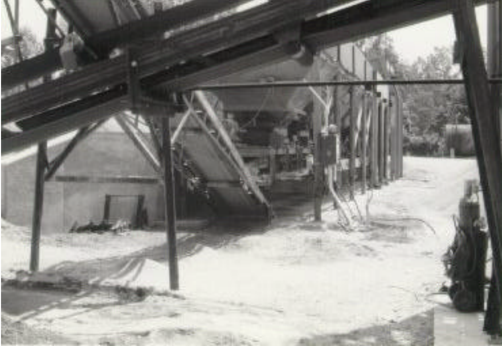
Figure 2.9 Aggregates feeder belt to shaker screen.
