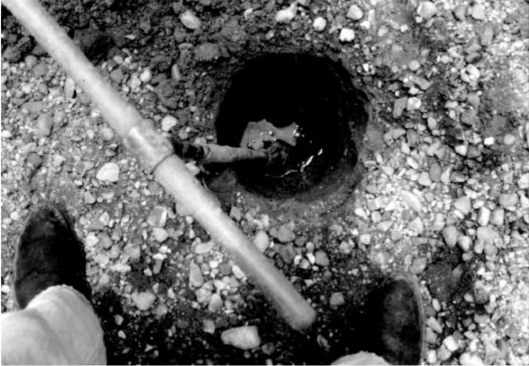
Figure 11. Water standing at moisture barrier.
