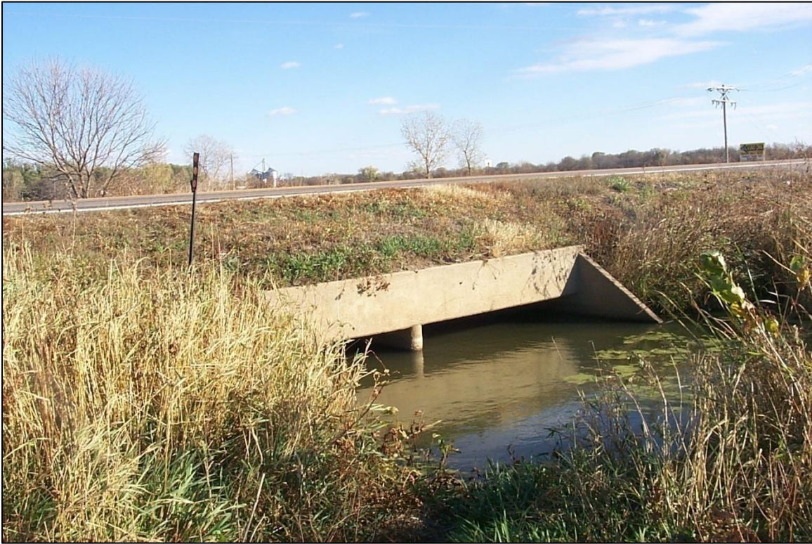
Figure 6. Unprotected roadside culvert
