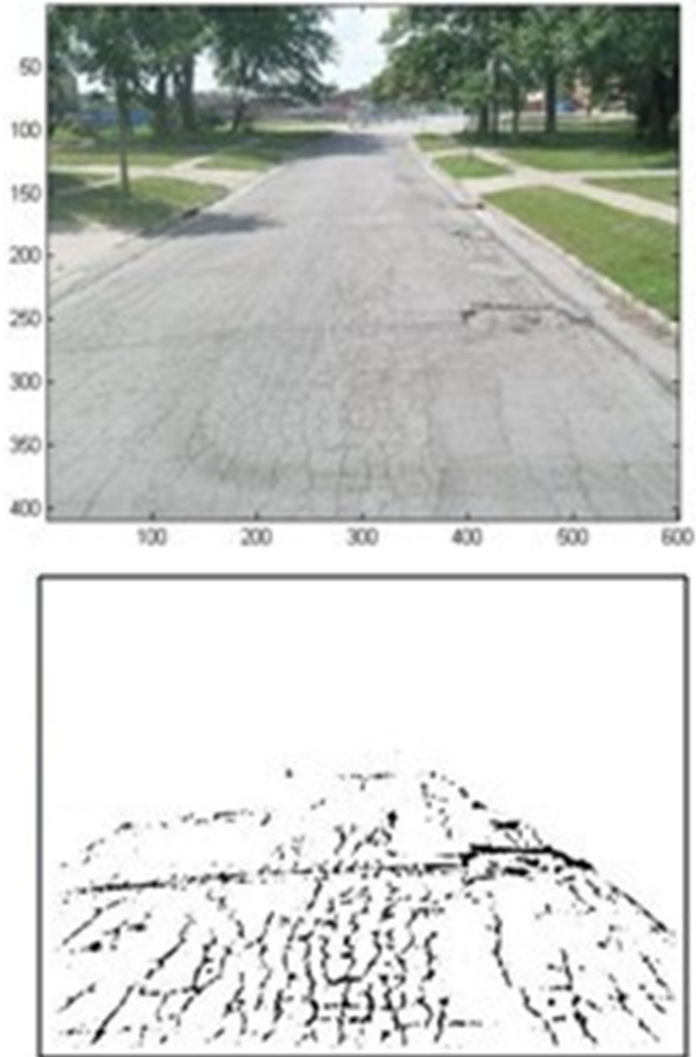
Figure 16: Pavement distress detection result No.2
