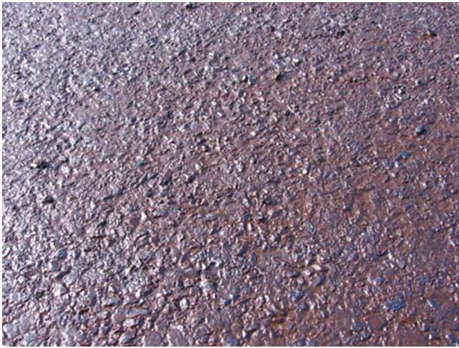
Figure 3.3 Close-up of Pavement Surface after Fog Seal
