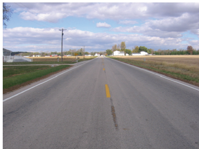
Figure 2.2 Photo of a Typical Fog-Chip Seal Pavement after 24 Months of Service
