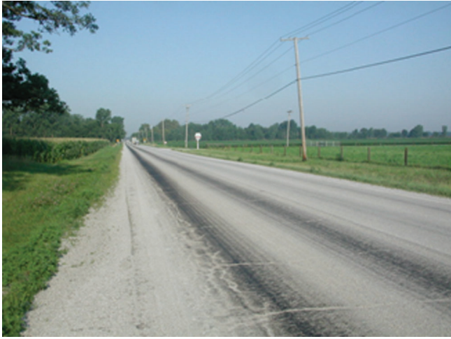
Figure 2.10 Photo of a Chip Seal on SR-10 after 36-Months of Service
