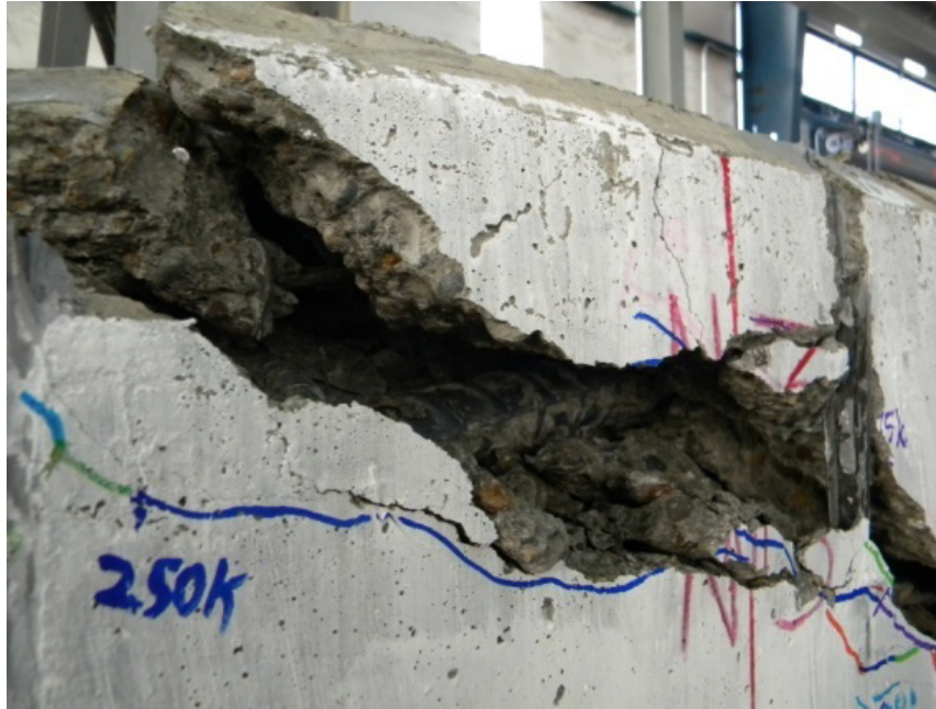
Figure 6.13: Specimen IT.7.18.12.S detachment of concrete cover between grid lines N1 and N3
