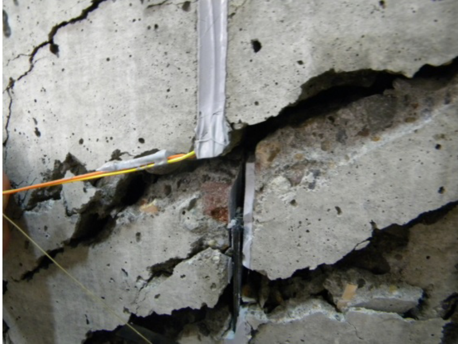
Figure 6.17: IT.7.22.6.FT/FTG CFRP rupture
