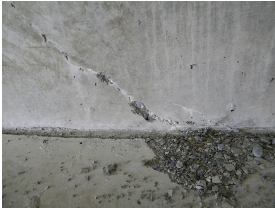
Figure 6.16: Specimen IT.7.22.6.FT/FTG typical raveling along a diagonal crack, scaling of concrete on flange soffit, and associated debris
