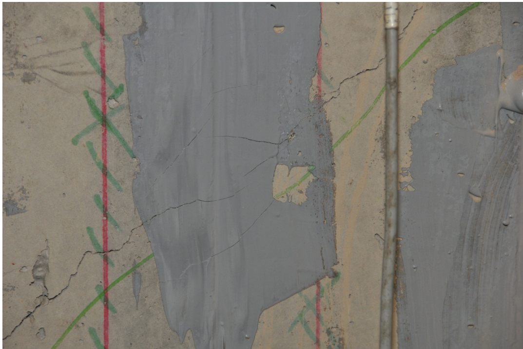
Figure 6.15: Example of crack feathering at NSM locations
