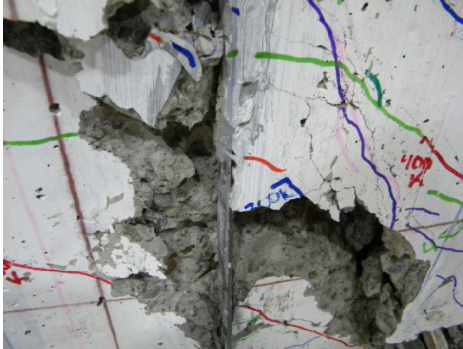
Figure 6.12: Example of debonding of NSM-CFRP
