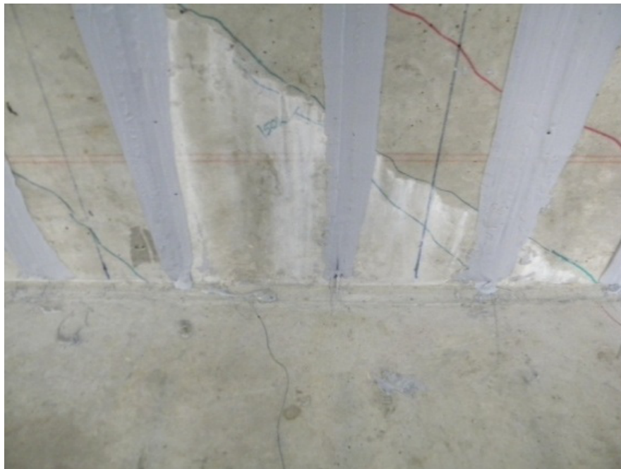
Figure 6.14: Specimen IT.7.22.6.FTG typical efflorescence
