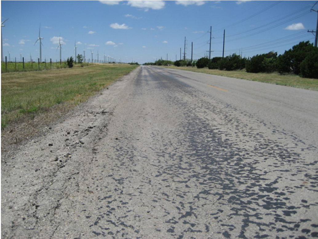
Figure 32. Failures, Alligator Cracks, Flushing (FM 89, Abilene District).
