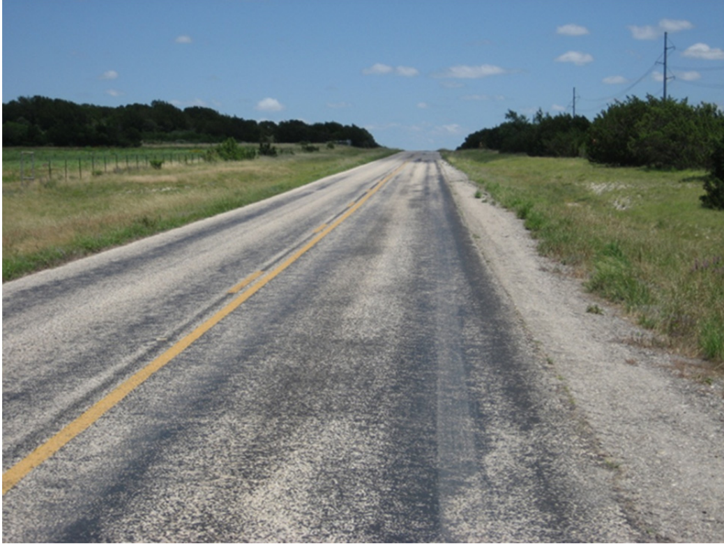
Figure 30. Flushing (FM 89, Abilene District).
