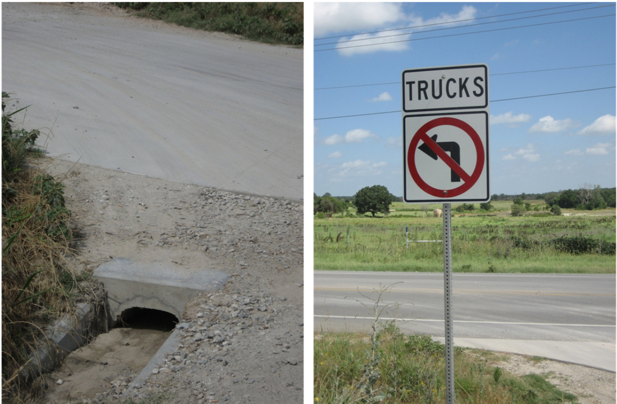
Figure 72. Tire Tracks on Driveway End Treatment and Illegal Left Turns (Fort Worth District).
