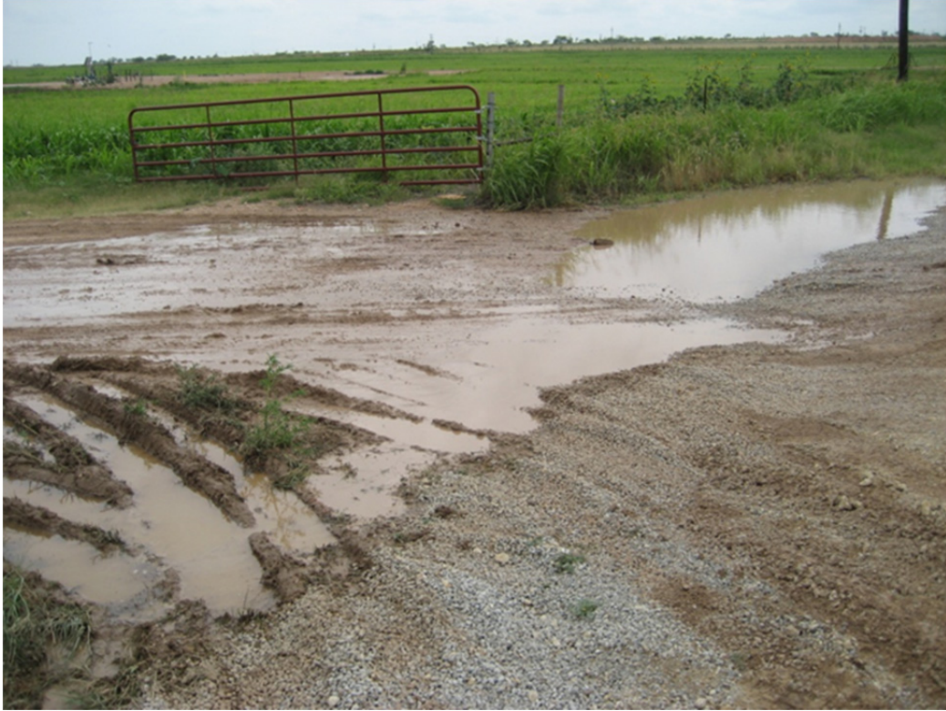
Figure 36. Drainage Problems (FM 1611, Abilene District).
