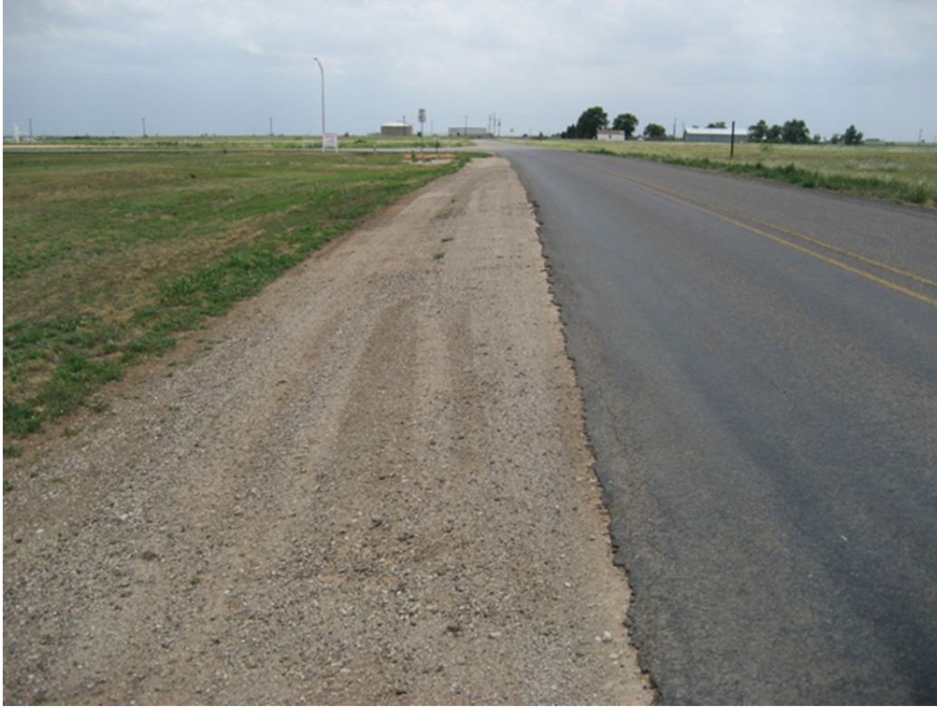
Figure 26. Edge Failure, Tire Tracks on Unpaved Shoulder (FM 2646, Lubbock District).
