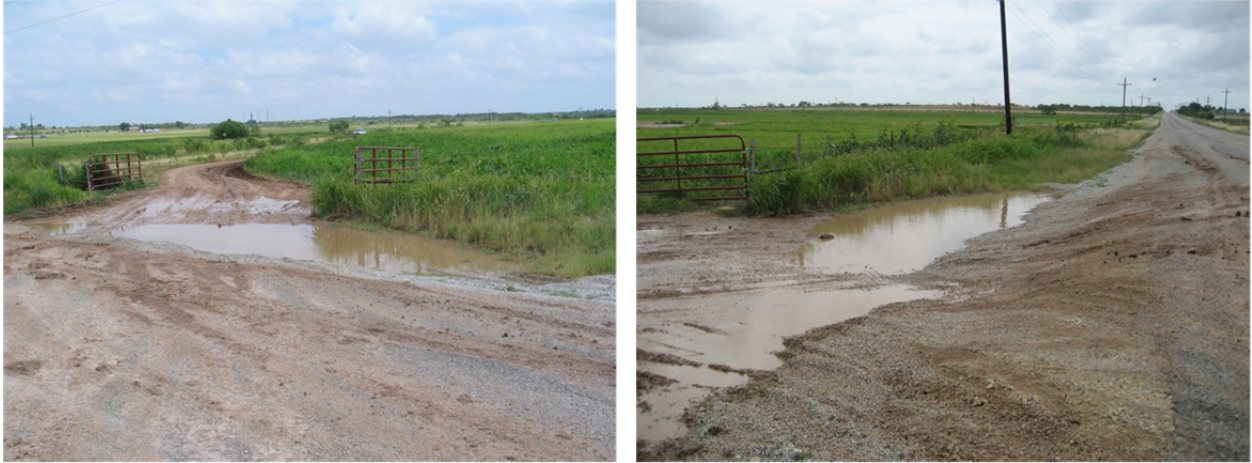
Figure 71. Drainage Problems and Mud Tracking (Abilene District).
