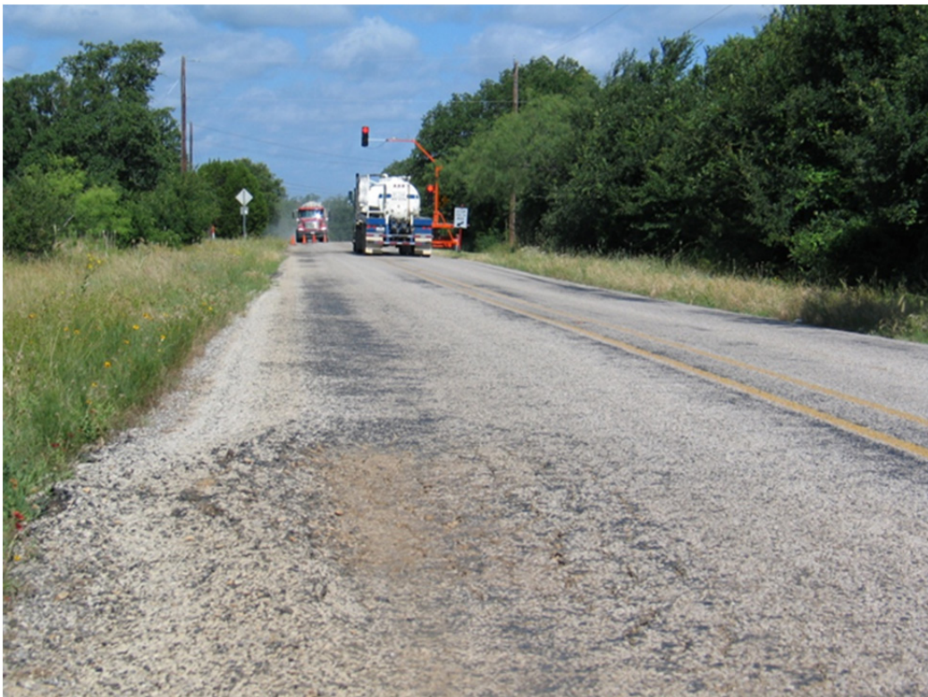
Figure 39. Failure, Flushing (FM 52, Fort Worth District).
