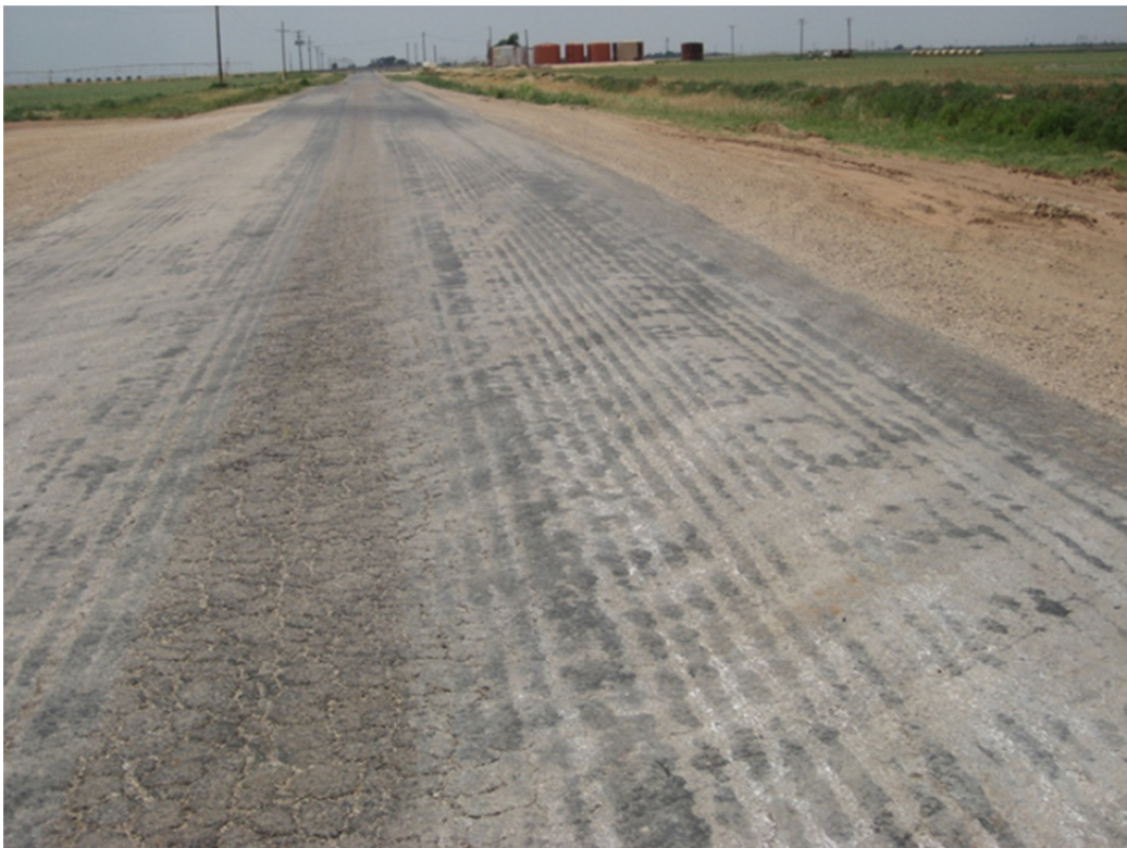
Figure 21. Pavement Failure, Surface Ripples (FM 1585, Lubbock District).
