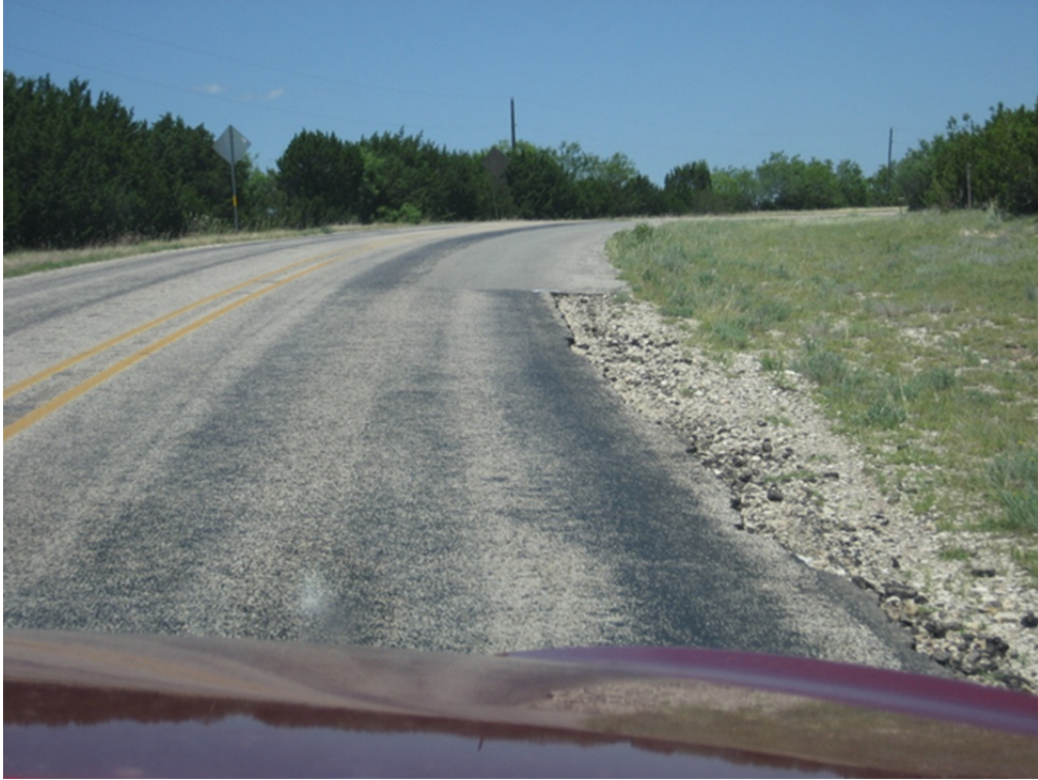
Figure 28. Edge Failure (FM 89, Abilene District).
