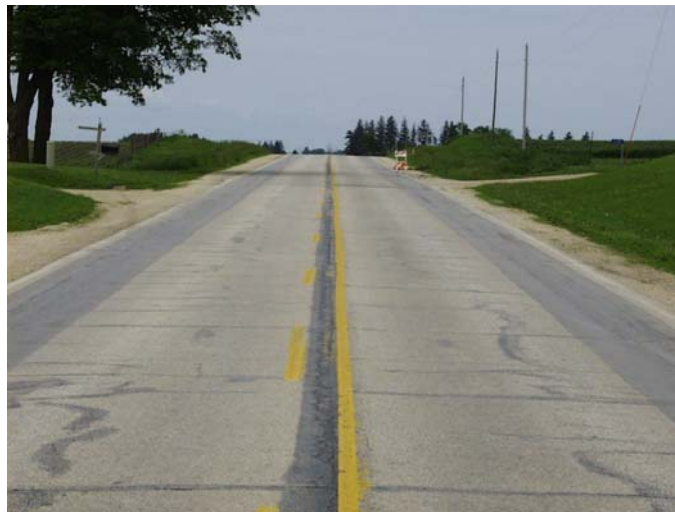
Figure 3. Longitudinal cracking and current condition of the roadway
