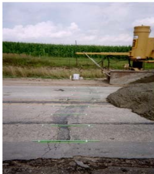
Figure 8. Tied transverse crack
