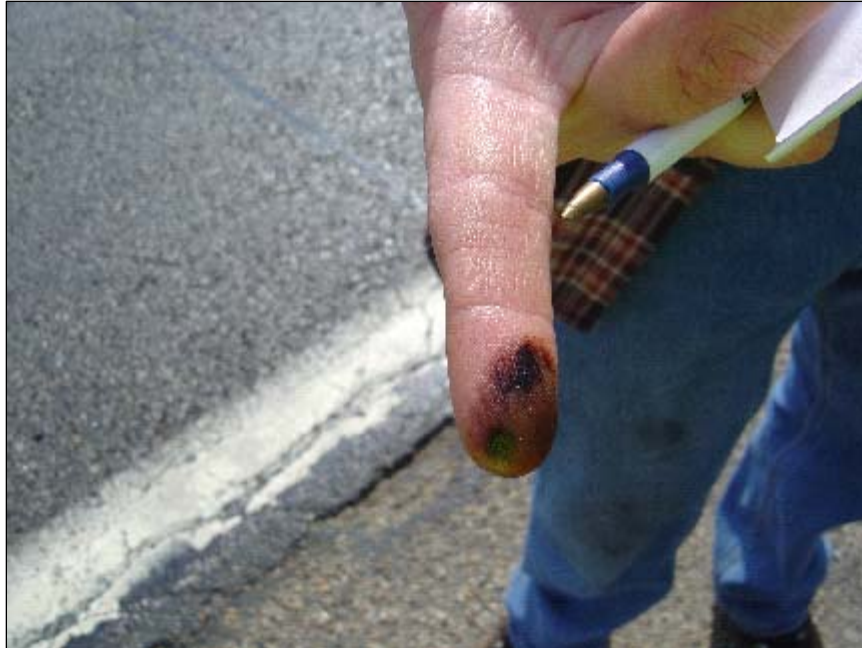
Photo 4, Softening of Joint Sealant
