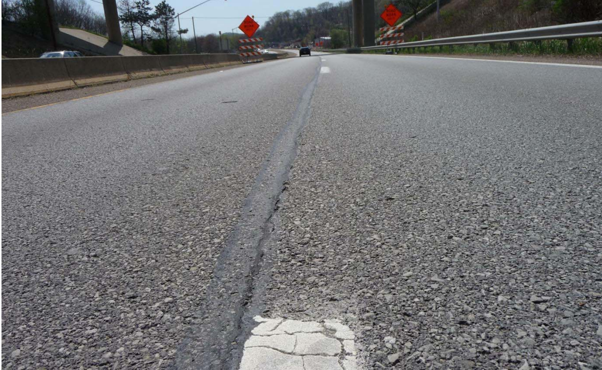
Photo 7, Close-up view of the pavement in April 28, 2009 (358 days after the application) Traveling lane (right in the Photo) was treated with RePlay, passing lane (left in the Photo) was untreated
