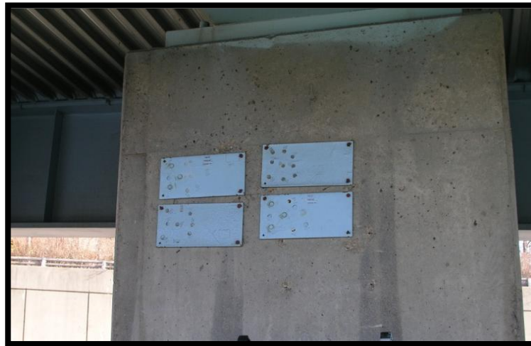
Photo 3, Control Panels attached to the Bridge
