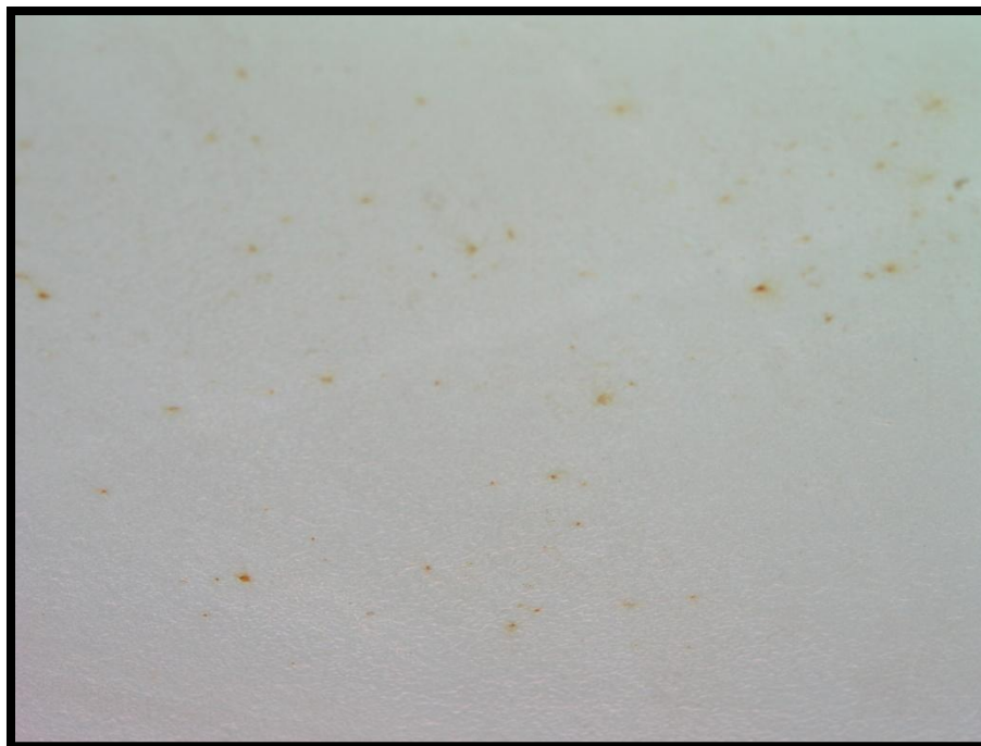
Photo 4, Spot surface rust on experimental area
