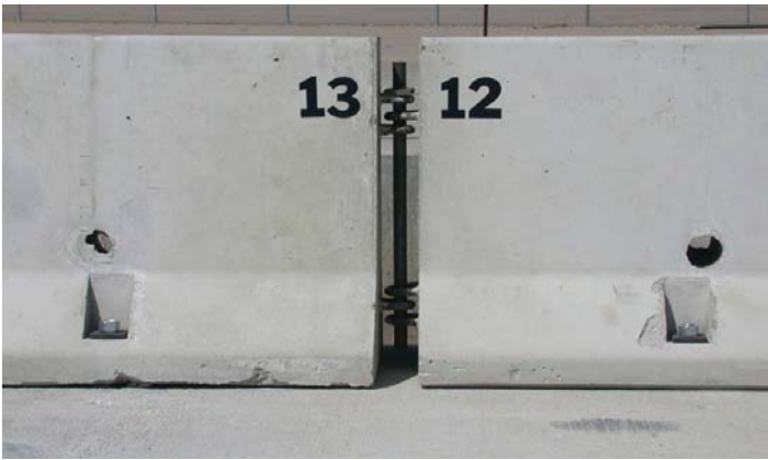
Above: Test K-barriers at the MwRSF in Lincoln, Nebraska. The barrier bases are attached to the concrete roadway surface by injecting epoxy into a drilled hole, inserting anchor bolts through each toe hole and into the drilled hole, and securing the bolts with a washer and nut above the toe hole.
