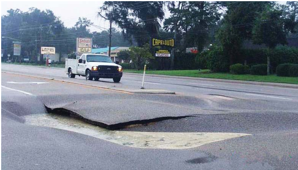
In August 2008, Tropical Storm Fay dropped 18-24 inches of rain in the Tallahassee, Florida, area. A section of Capital Circle Northeast/U.S. 319 buckled and collapsed when underground drainage pipe failed.
