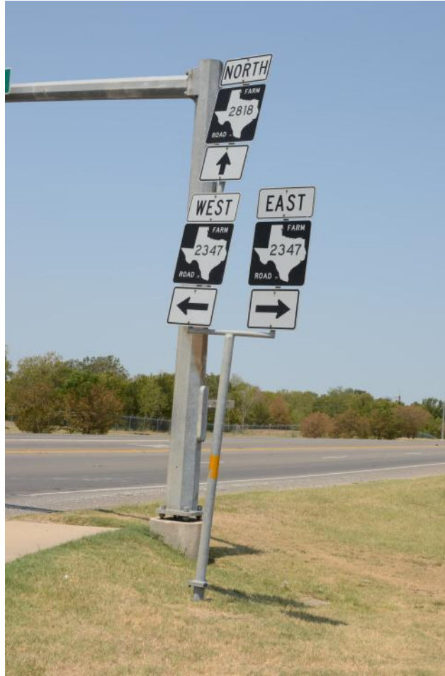
Figure 11.1. Example of U-Bracket Failure.
