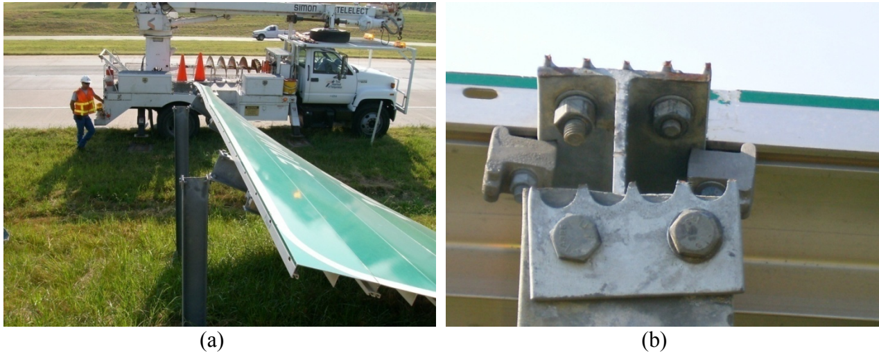
Figure 5.7. Typical Fuse Plate Failure Mode Reported by Districts.
