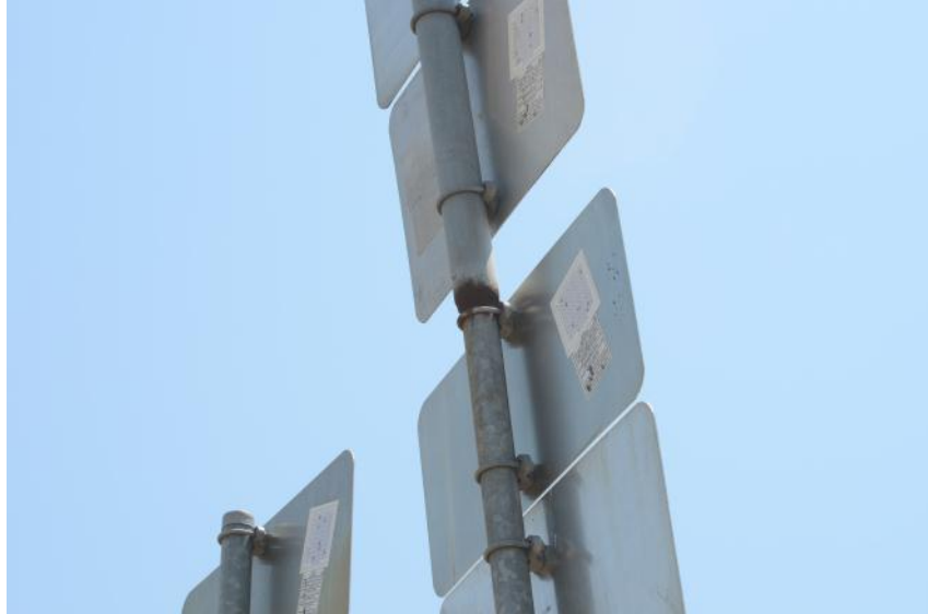
Figure 11.3. Improper Installation of U-Bracket Extension Tube.
