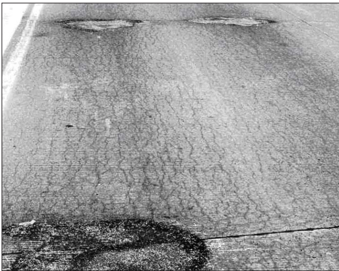
Figure 3.3 Deficient air-void system resulting in freeze-thaw damage
