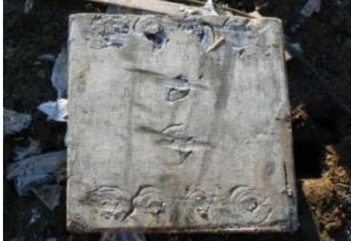
Figure 5.13. Condition of pile head at the end of driving pile P1
