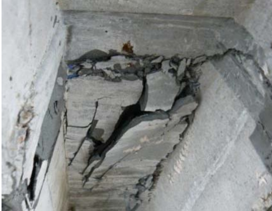
Figure 5.47. Damaged region of UHPC Pile 1 at the end of the lateral load test
