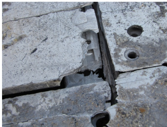
Figure 124 – Severe damage to top plates and webs
