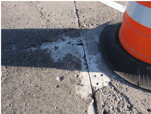
Figure 123 – Wearing surface damage at intersecting panels
