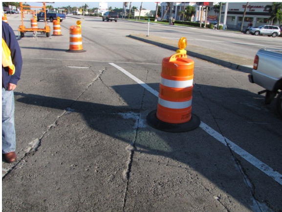
Figure 122 – Wearing surface damage at panel joints
