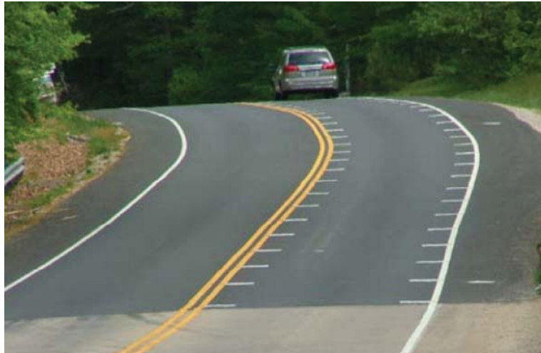
Figure 73. Optical Speed Bars Used to Reduce Vehicle Speed. (Courtesy of Virginia Department of Transportation)
