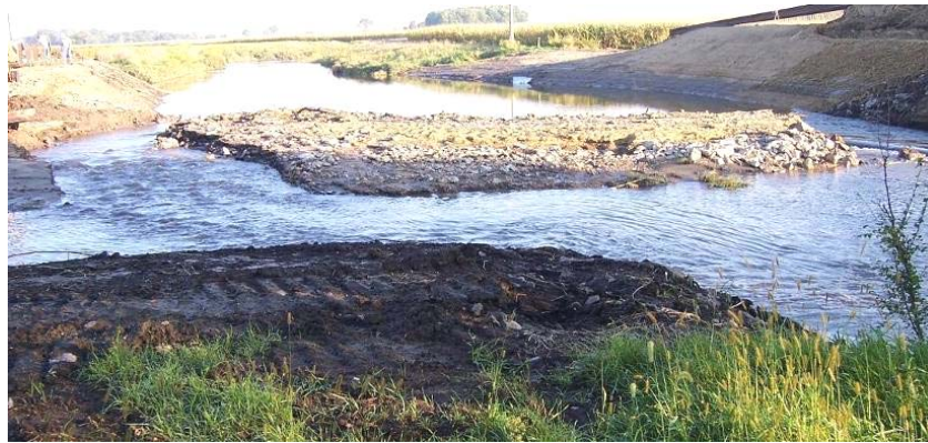
Figure 106. Washed out access road, September 15
