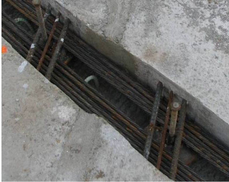
Figure 2.17. Photograph of longitudinal post-tensioning channel prior to casting concrete in the field
