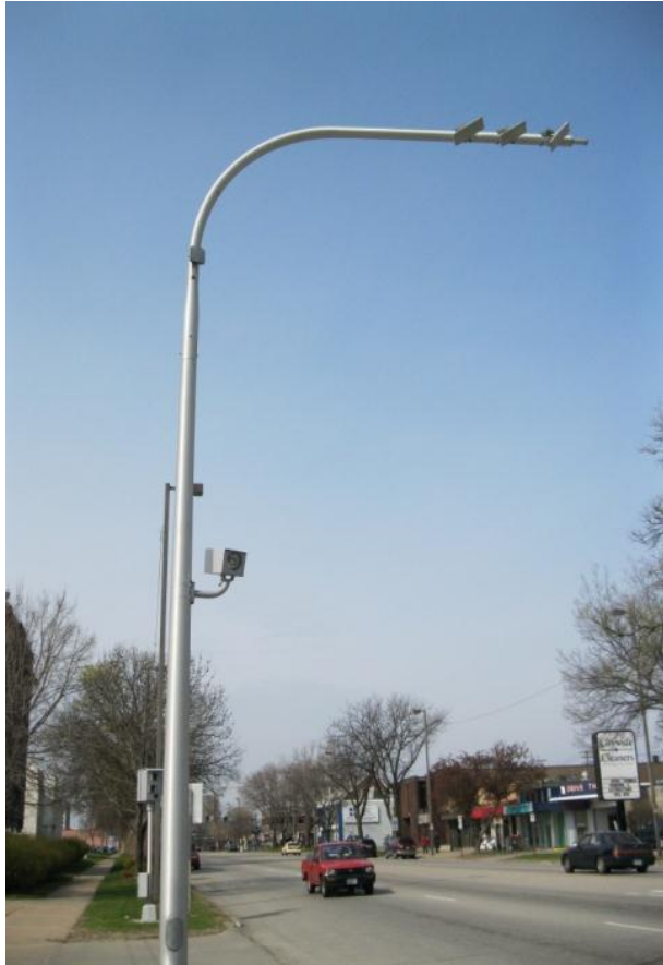
Figure 2.8. Mast arm and RF antenna setup
