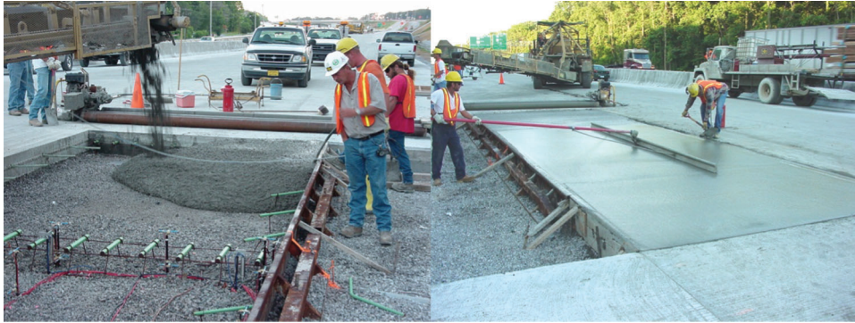
Figure 2.5 Concrete placement of the 14-inch thick and 18-foot joint spacing slabs (north)
