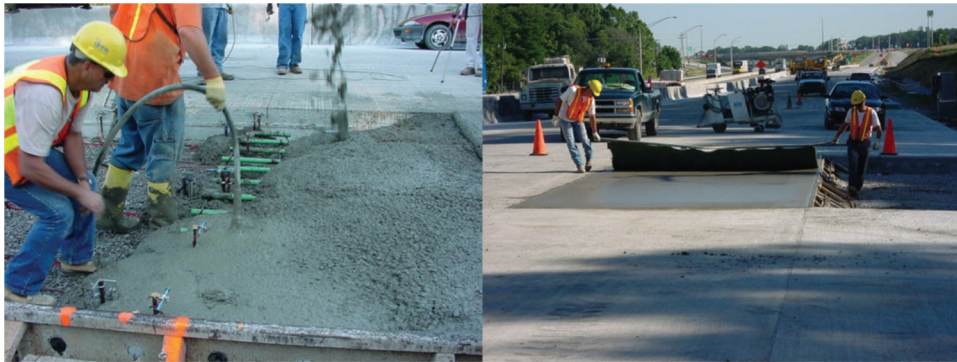
Figure 2.6 Concrete placement of the 15-inch thick and 18-foot joint spacing slabs (mid)
