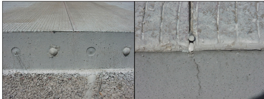
Figure 2.9 Joint saw cut conditions the day after saw cutting
