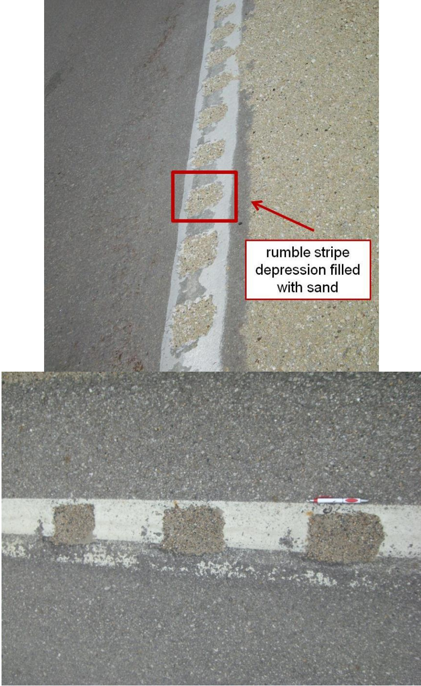
Figure 3.4. Rumble stripe depression filled with material
