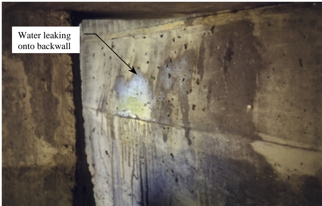
Figure 6.27 Backwall below left gutter at G2 of Bridge 7 (8561.5L030)
