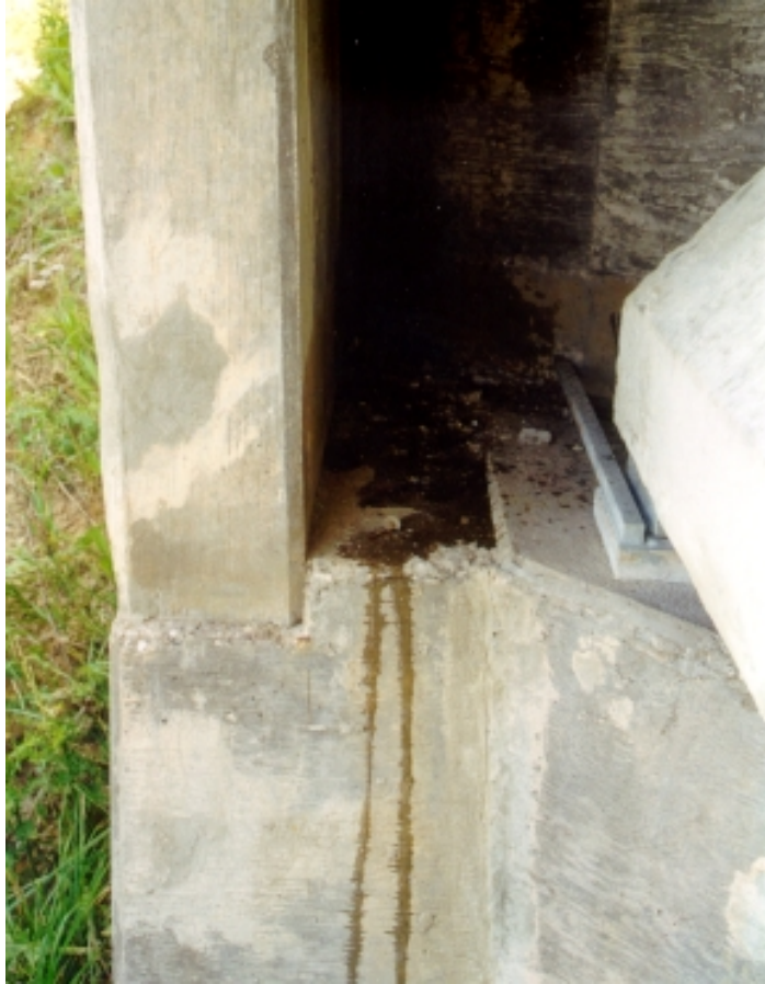
Figure 6.41 Leakage observed underneath G2 for Bridge 11 (6403.6L014)
