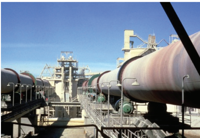
Figure 4.1 A cement kiln (photo courtesy of PCA)
