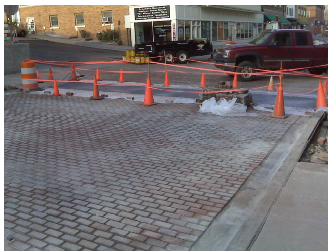
Figure 3.6 Vehicular interlocking concrete pavers being placed in a historic downtown area (note the use of colored concrete to provide a visual offset for the crosswalk) (photo courtesy of Tom Van Dam, CTLGroup)
