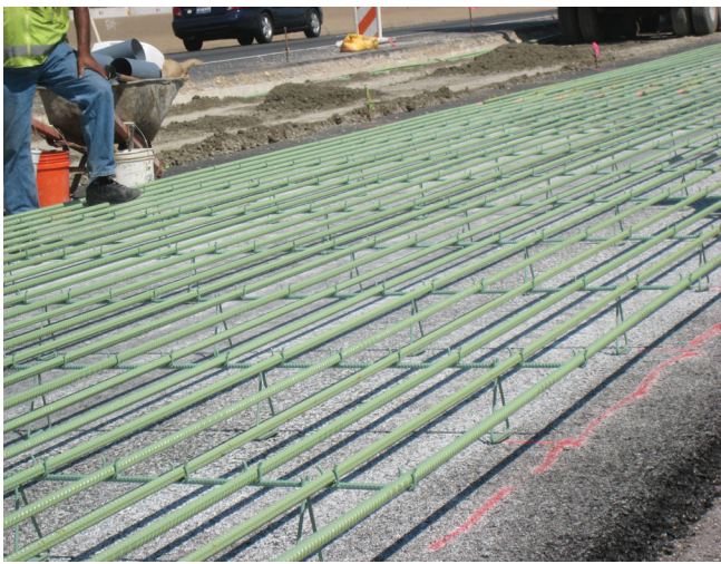
Figure 4.10 Reinforcing for CRCP (photo courtesy of Mike Ayers, American Concrete Pavement Association)
