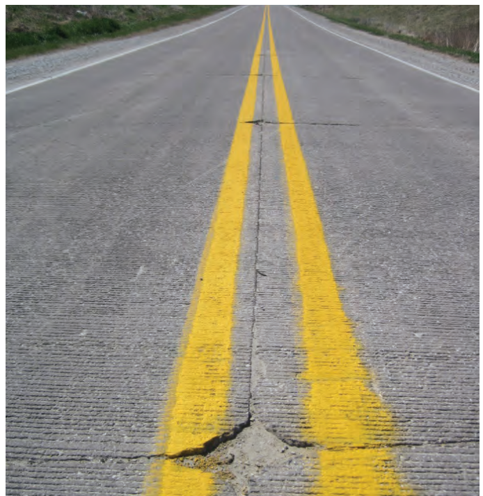
Figure 23. Damage starting at joint intersections
