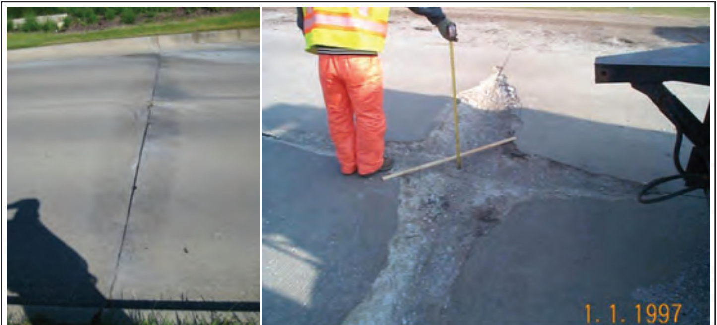
Figure 6. Evolution of joint deterioration from shadowing (left) to high severity (right)
