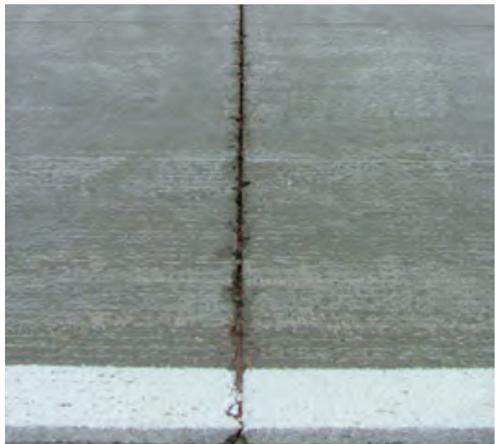
Figure 22. Joint deterioration due to raveling from improper saw-cut procedures
