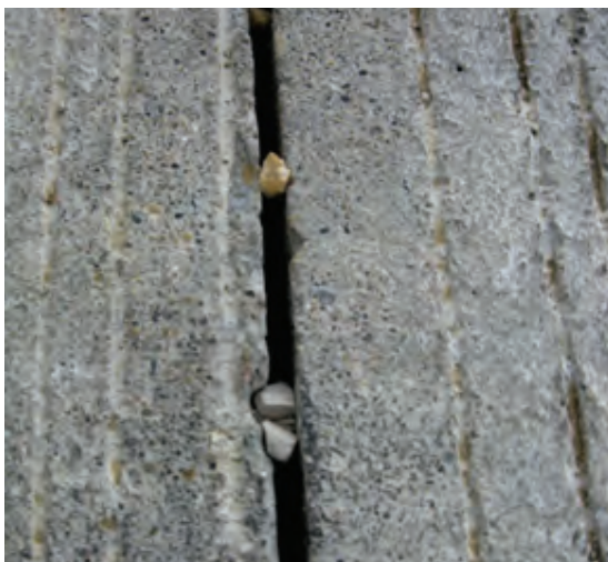
Figure 1. Incompressibles causing mechanical damage, which can lead to further distress
