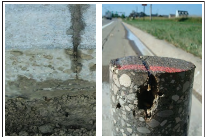
Figure 15. Saturated soils due to inadequate drainage and roadside irrigation (left) leading to joints showing frost damage (right) (Source [left]: Snyder and Associates)
