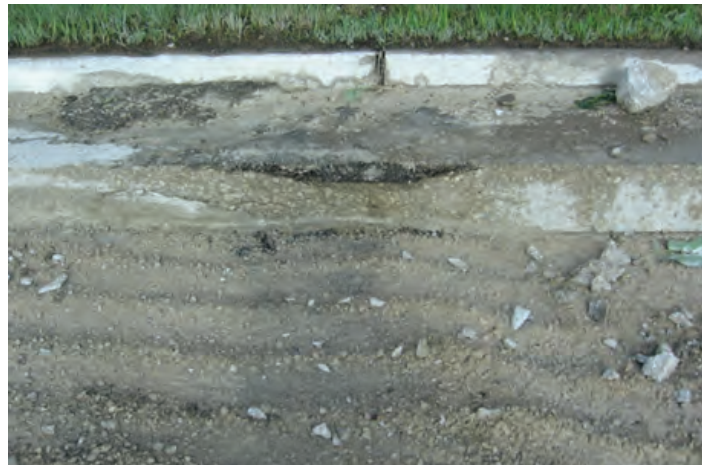
Figure 7. Typical saturated foundations under a shadowed section (Source: Snyder and Associates)
