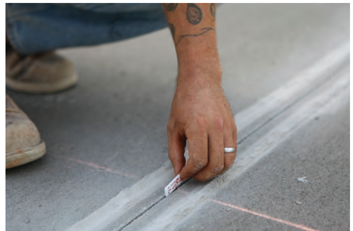
Figure 28. Using temporary joint spacers to protect and minimize damage due to early entry sawing (Source: Husqvarna)
