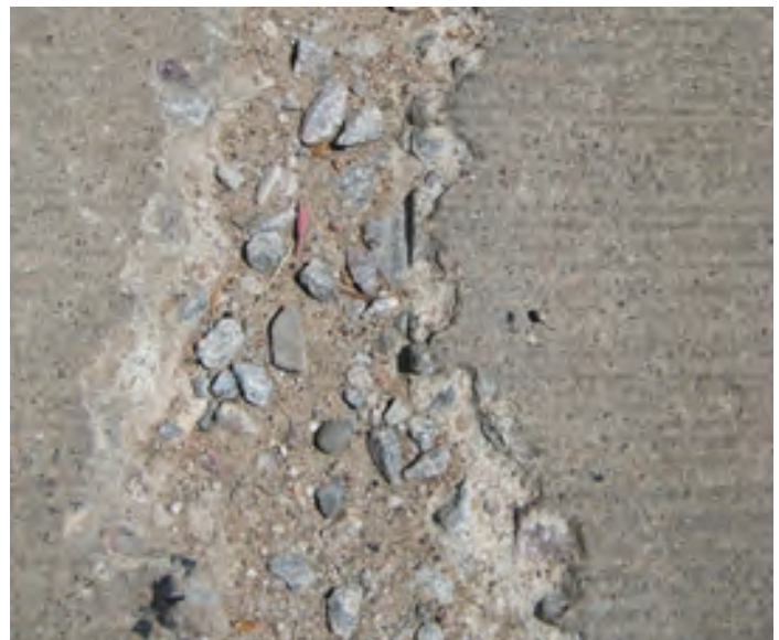
Figure 11. Shallow joint damage
