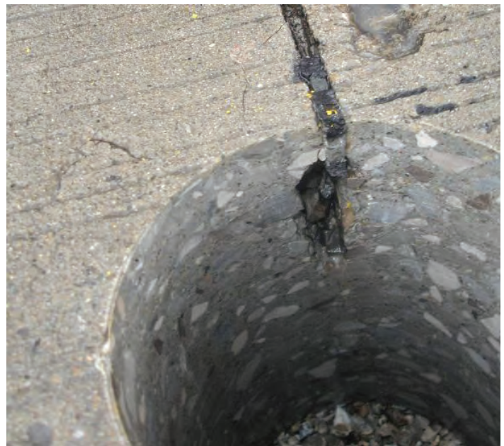
Figure 29. Evidence of saturation within joint beneath seal (Source: Purdue)
