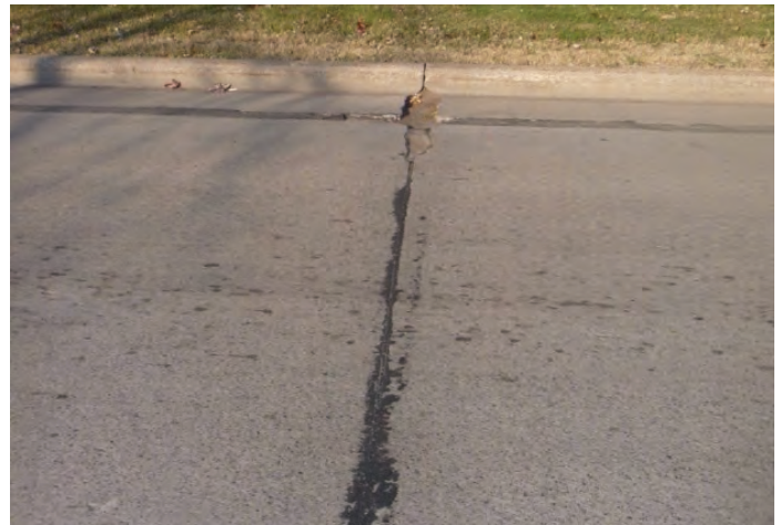
Figure 31. Failing transverse joint associated with poor drainage at gutter
