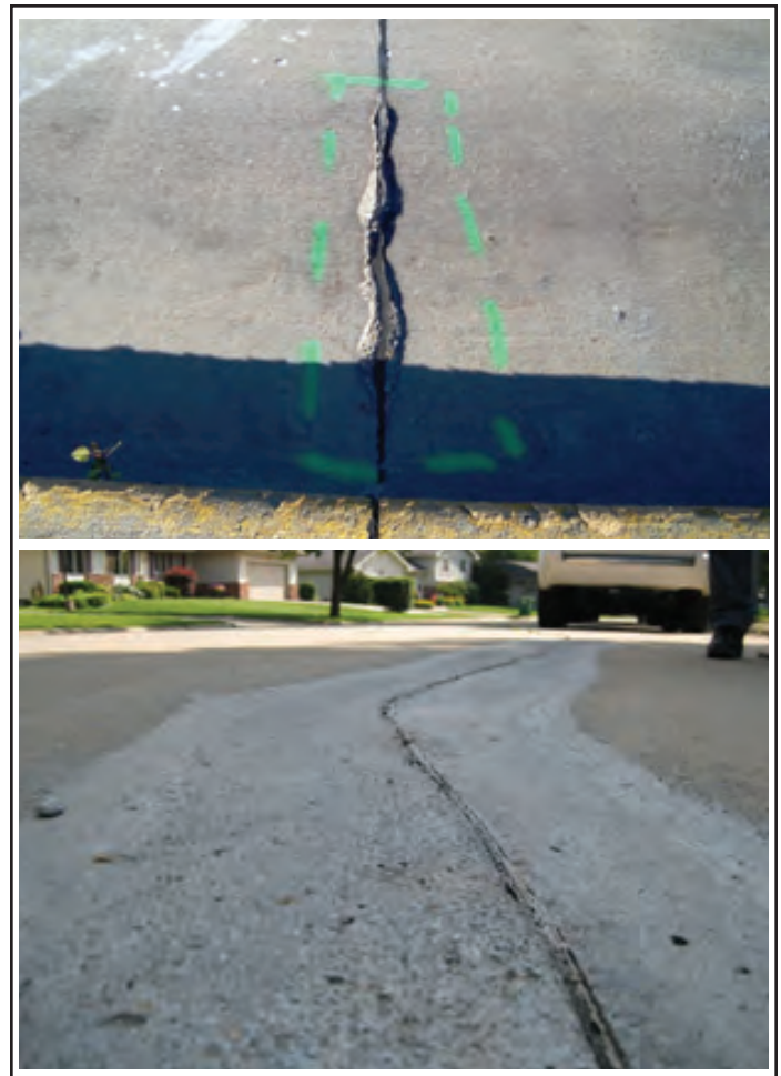
Figure 37. Delineation of spalled area for partial-depth repair (top) and a completed patch (bottom) (Source [bottom]: The Transtec Group)
