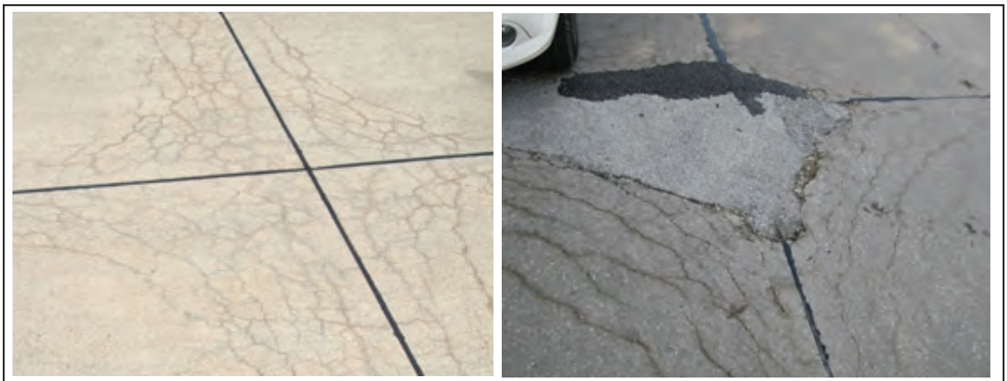
Figure 5. D cracking of low severity (left) and high severity (right) (Source: The Transtec Group)
