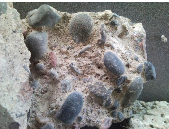
Figure 10. Coarse aggregate exposed by damage to the paste
