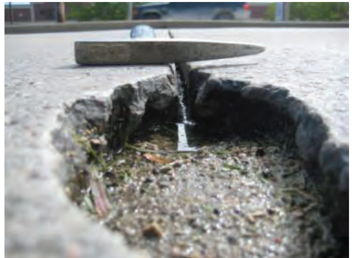
Figure 25. Example of a poorly draining pavement
