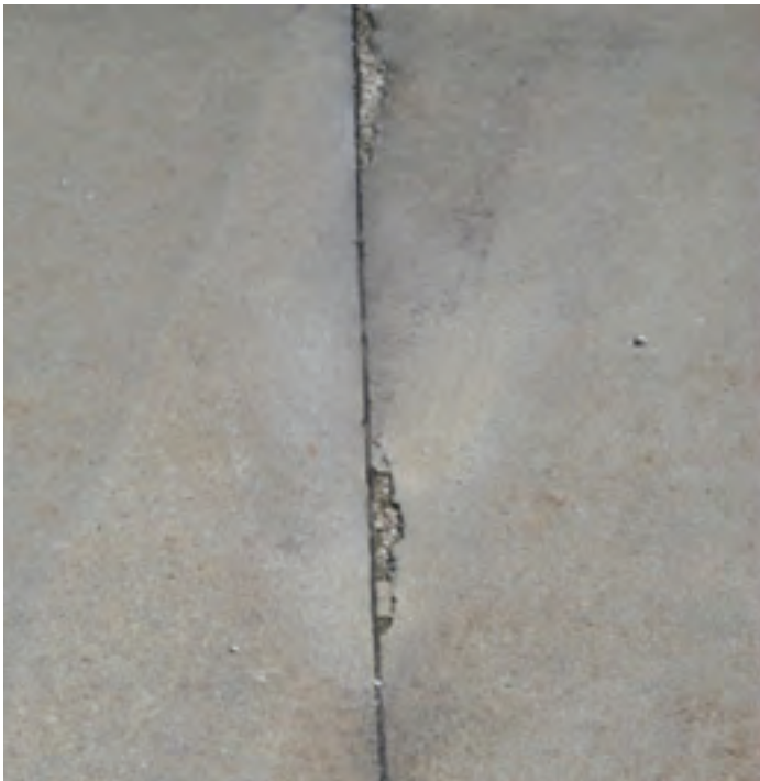
Figure 13. Water flow through joints from a high water table (bottom-up moisture); note staining on surface
