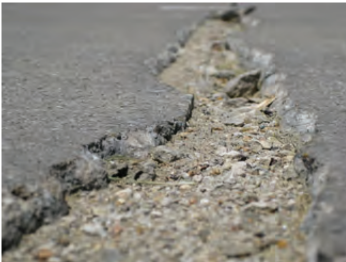
Figure 18. Top-down joint distress, with vertical edges and shallow depth
