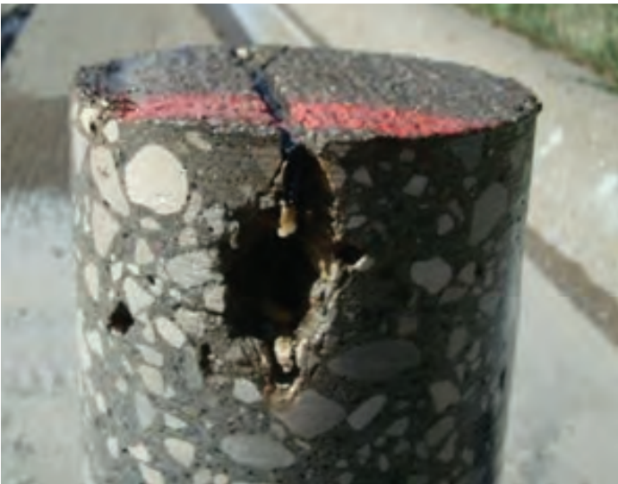
Figure 19 Joint deterioration evident below the joint sealant
