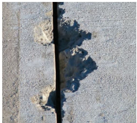
Figure 2. Raveling due to poor sawing practice (Source: Iowa Department of Transportation)
