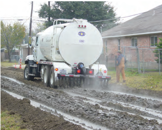
Figure 7-4. Applying cement slurry on grade prior to mixing (cement slurry is applied the same way for CTB applications)
