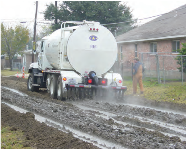
Figure 6-5. Applying cement slurry on grade prior to mixing (cement slurry is applied the same way for FDR and CMS applications)
