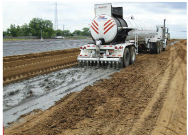
Figure 8-2. Cement slurry added to subgrade material (cement slurry is applied the same way for CTB and FDR applications)
