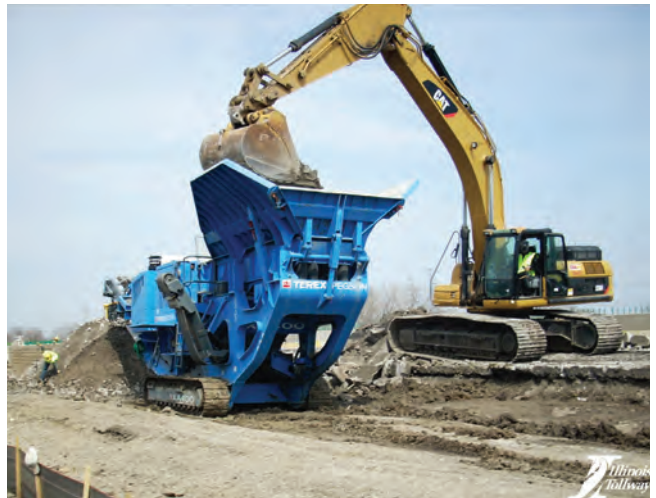
Figure 9-4. Existing concrete recycled in-place and reused for base material on the Tri-State Tollway in Illinois
