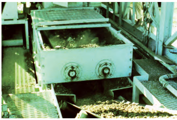
Figure 5-12. Mobile RCC pugmill mixing plant and mixing chamber
