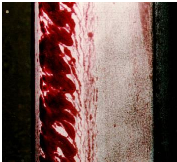
Figure 18. Hydraulic Mechanism Is No Doubt Contributing to Shelling on This High Rail; Cracking Is Enhanced by Dye Penetrant
