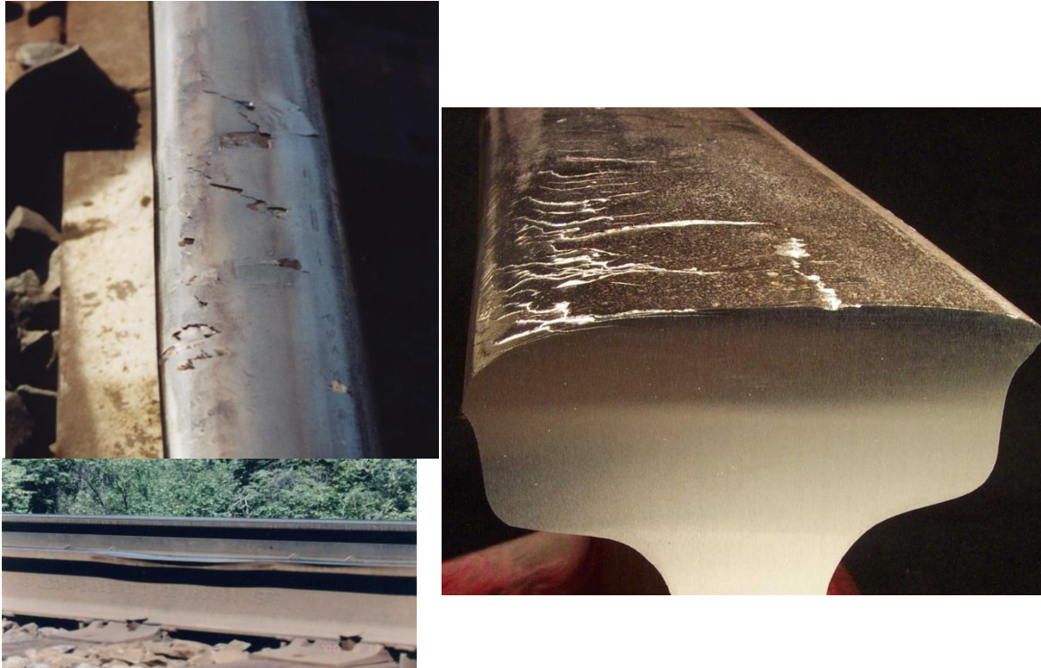
Figure 13. The Crushed Head Defect Is Associated with Collapse and Deformation of the Underside of the Rail Head as a Result of Cracks That Initiate at the Mid-Gauge and Propagate to the Center of the Rail
