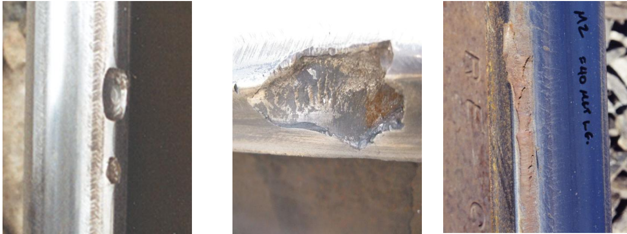
A) Loss of rail cant due to rail seat abrasion resulted in overloading of the gauge corner B) Well-lubricated rail with a sharp gauge corner C) Gauge corner collapse in a dry environment
