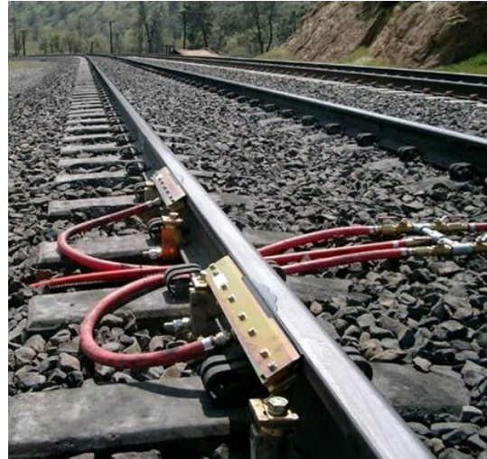
Wayside systems dispense a product to the running surface of the rail which is picked up by the wheel and dispersed along the rail length.
