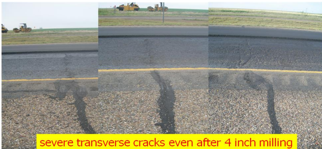
Figure 17. Existing Pavement Conditions of IH40 after Milling.
