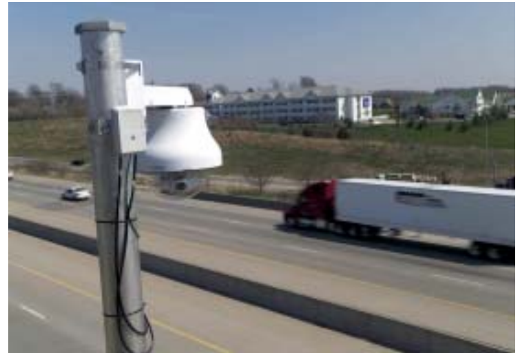
Pole-mounted camera on I-235 in Des Moines
