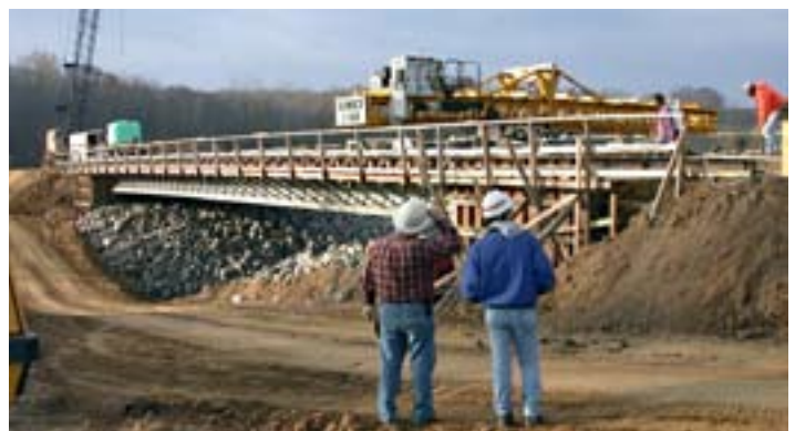
Figure 10 - The United States' first UHPC bridge was built in Wapello County (deck placement after UHPC I-shape girders placed).
