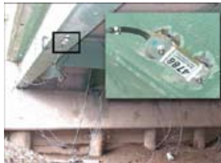
Figure 2 - Multiple BDI strain gauges placed on bridge girders for load rating test.
