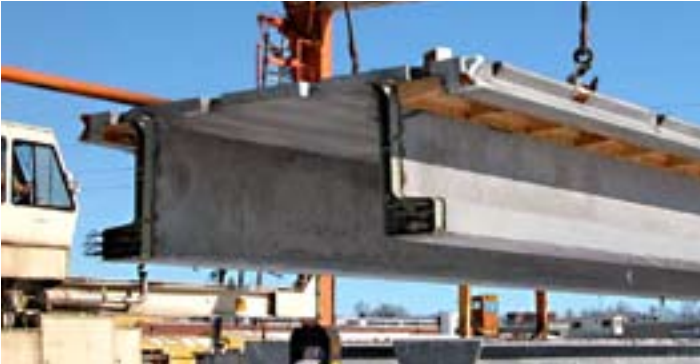
Figure 11 - The first bridge in the United States to use new generation Pi-shaped girders will be constructed in Buchanan County.
