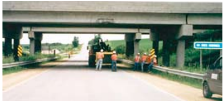
Figure 17 - View of damaged exterior girder in the center span of the Beebeetown bridge, westbound on I-680 in western Iowa; damage was restricted to the exterior and first interior prestressed girders.
