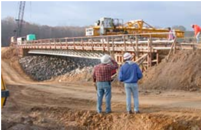
Figure 27 - Deck placement after UHPC pi-shaped girders are in place; this was the first UHPC bridge designed and constructed in the United States and is maintained by Wapello County.
