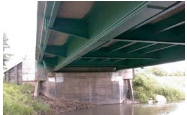
Figure 5 - Two-girder bridge system with cover plates and strengthening angles on the two girders
