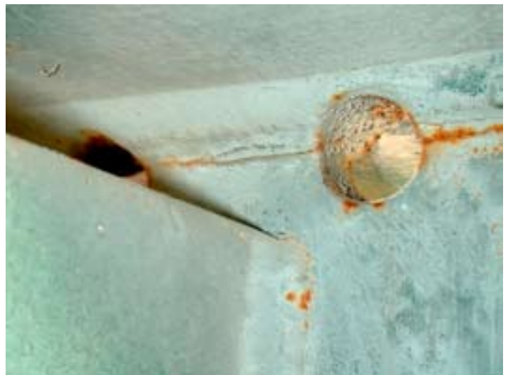
Figure 22 - A web gap on the I-35 bridge showing previously developed cracks; for the initial retrofit, holes were drilled at the ends of the crack. However, cracking continued to spread beyond the hole retrofit.
