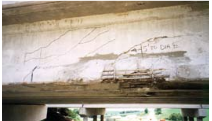
Figure 18 - Close-up view of damaged exterior and interior girders; the damage included loss of section properties and severe cracking, as well as damage to prestressed strands.
