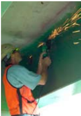
Figure 2 - Preparation of surface for bonding sensors requires more effort on painted steel than on concrete; the paint and primer must be completely removed on steel and surface made flat for good bonding.
