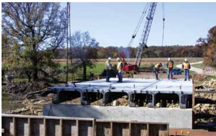
Figure 7 – Field instrumentation and monitoring were used in a live-load field testing process to assess the condition of the recently constructed Jakway Park Bridge.
