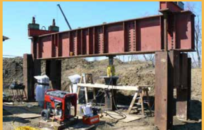
Vertical load test of the steel pile at the Oskaloosa test site
