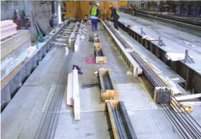
Figure 10 – Layout of UHPC units for the first of two pours at Coreslab Structures Inc. near Omaha, Neb.
