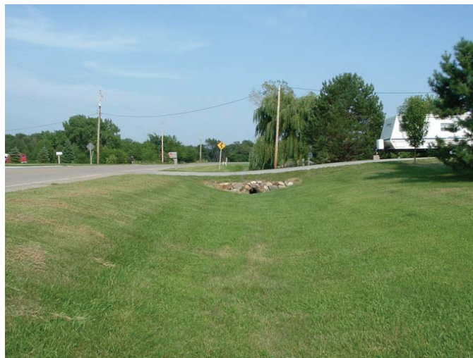
An example of a well designed drainage system
