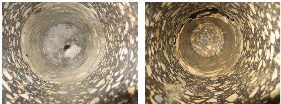
Layer condition underneath HMA after coring - (Right) PCC layer without rubblization on IA-139 in Winneshiek County, Iowa and (Left) Rubblized PCC layer on IA-3 in Delaware County, Iowa
