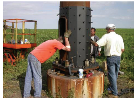
A bolted reinforcing jacket was placed on a tower in the I-35 & US 18 Interchange near Clear Lake.
