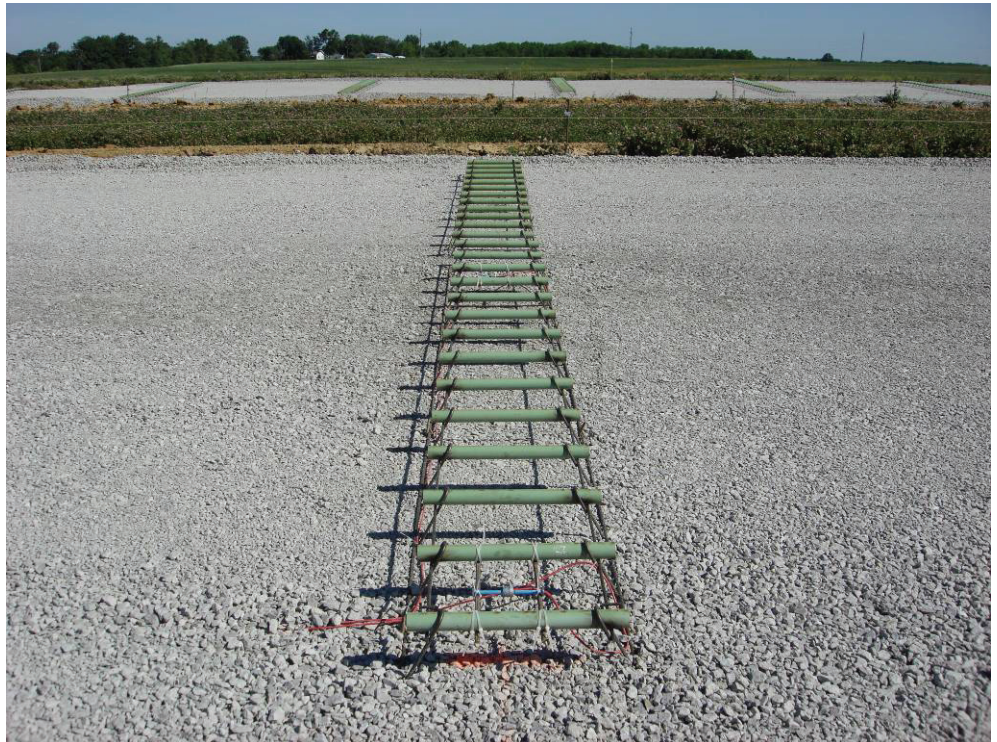
Strain gages installed at joints just before paving to monitor the stress resulting from concrete shrinkage (US 34 Fairfield bypass)
