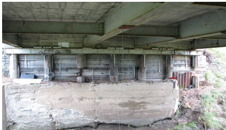
During removal of a bridge in Humboldt County, testing of the super- and sub-structure is made - instrumentation on the piling is visible
