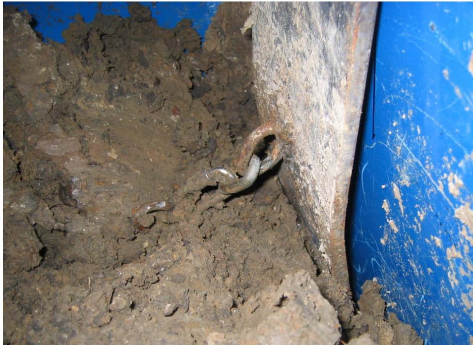
FIGURE 5.15 Anchor plates pulled out from the rear face of the wall
