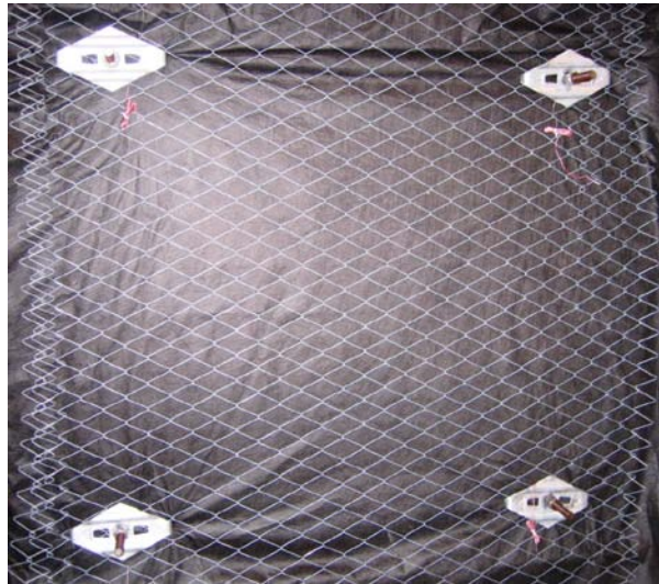
FIGURE 4.9 Galvanized wire mesh and geotextile at the front face of the soil nailed wall
