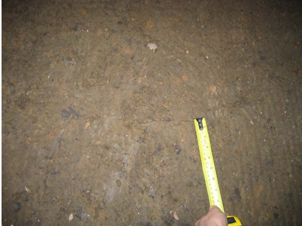
FIGURE 5.18 Crack seen on the top surface close to the front face of the nailed wall
