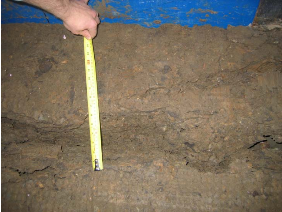
FIGURE 5.16 Crack developed at failure at 1 ft from the rear face of the wall
