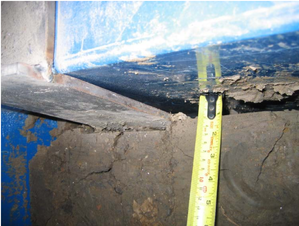
FIGURE 5.17 Movement of soil mass out of the rear face of the wall
