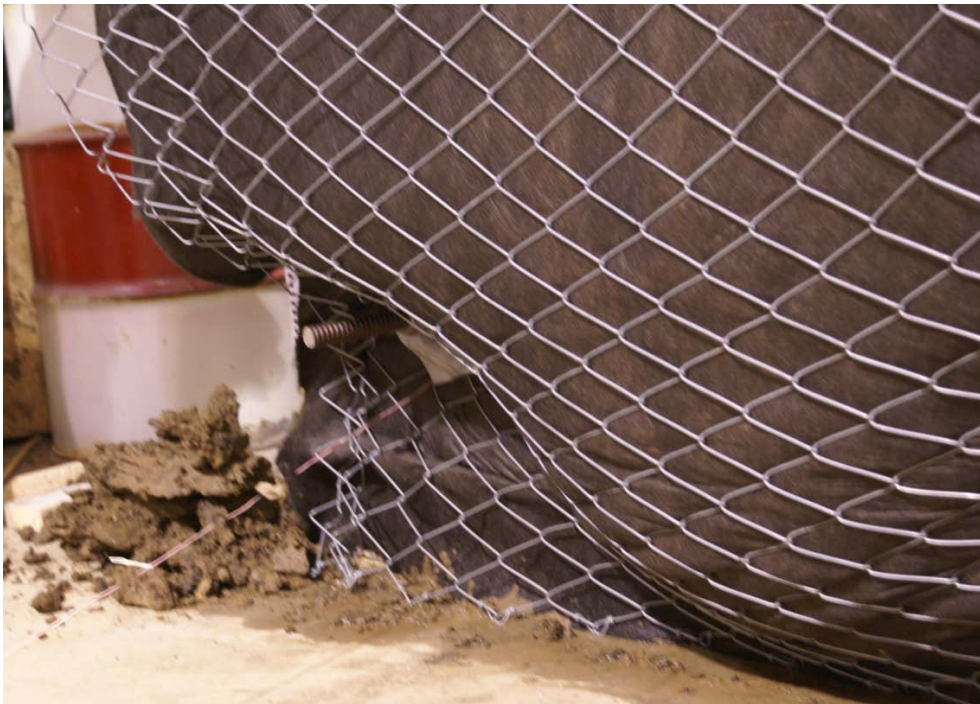
FIGURE 5.12 Lower left nail after failure
