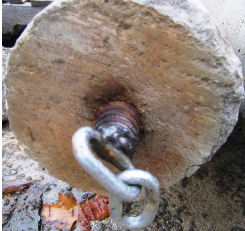
FIGURE 4.7b Chain link on the soil nails
