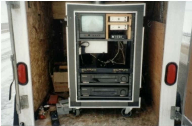
Figure 6 AutoScope™ Equipment and Data Collection Trailer
