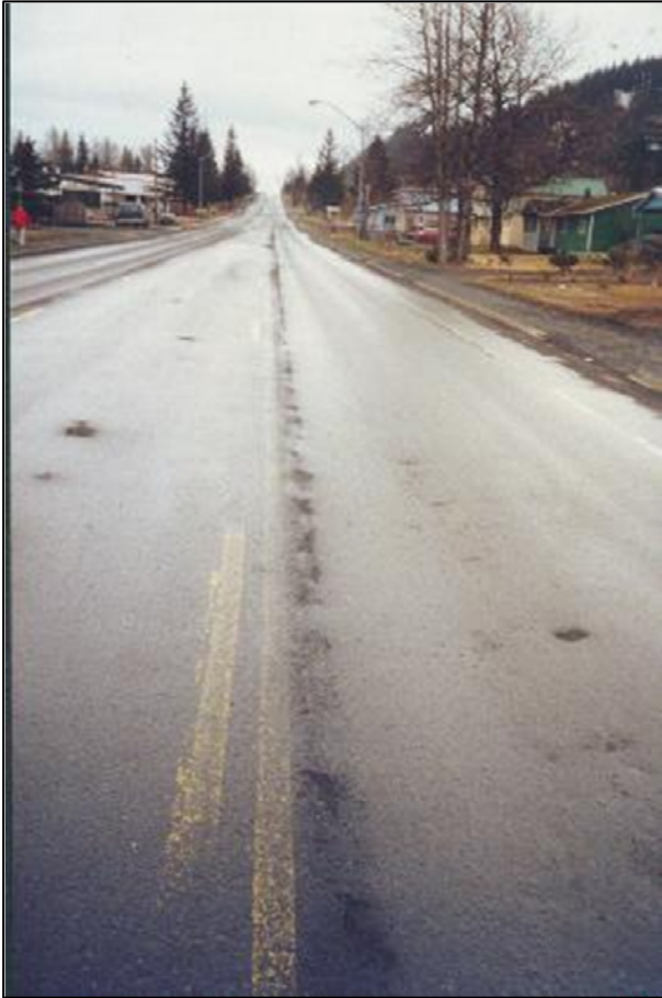
Figure 1. Photograph Showing an Example of Accelerated Deterioration Along a Longitudinal Centerline Joint that was Inadequately Constructed
