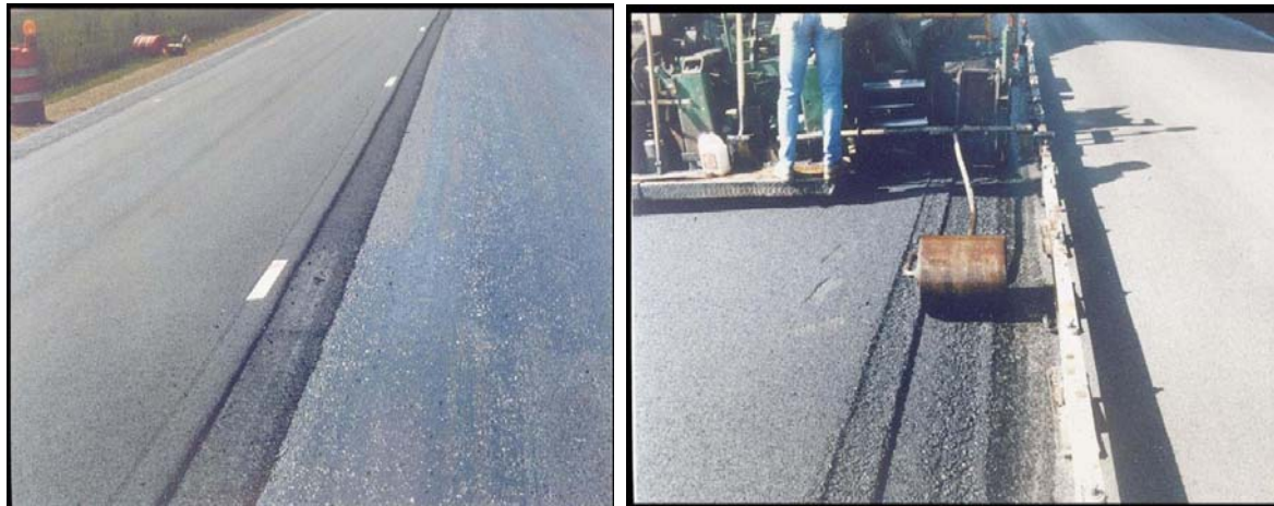
Figure 8. Notched Wedge Joint (a small steel drum is attached to paver to roll the wedge behind the paver)
