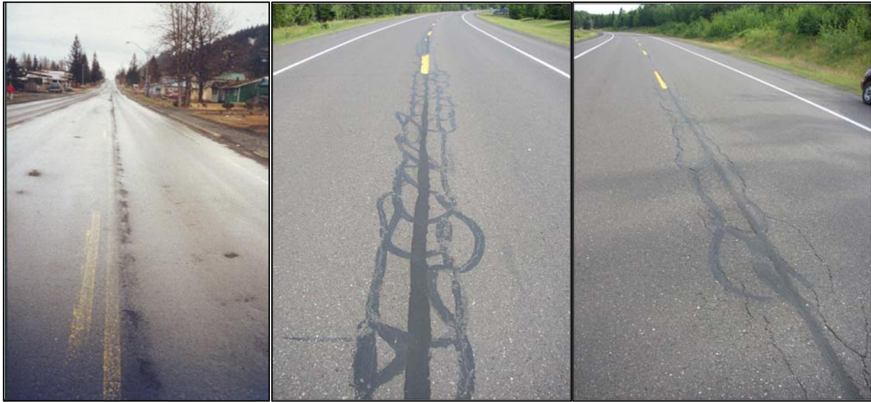
Figure 49. Cracking and Accelerated Deterioration Along Longitudinal Centerline Joints that were Inadequately Constructed
