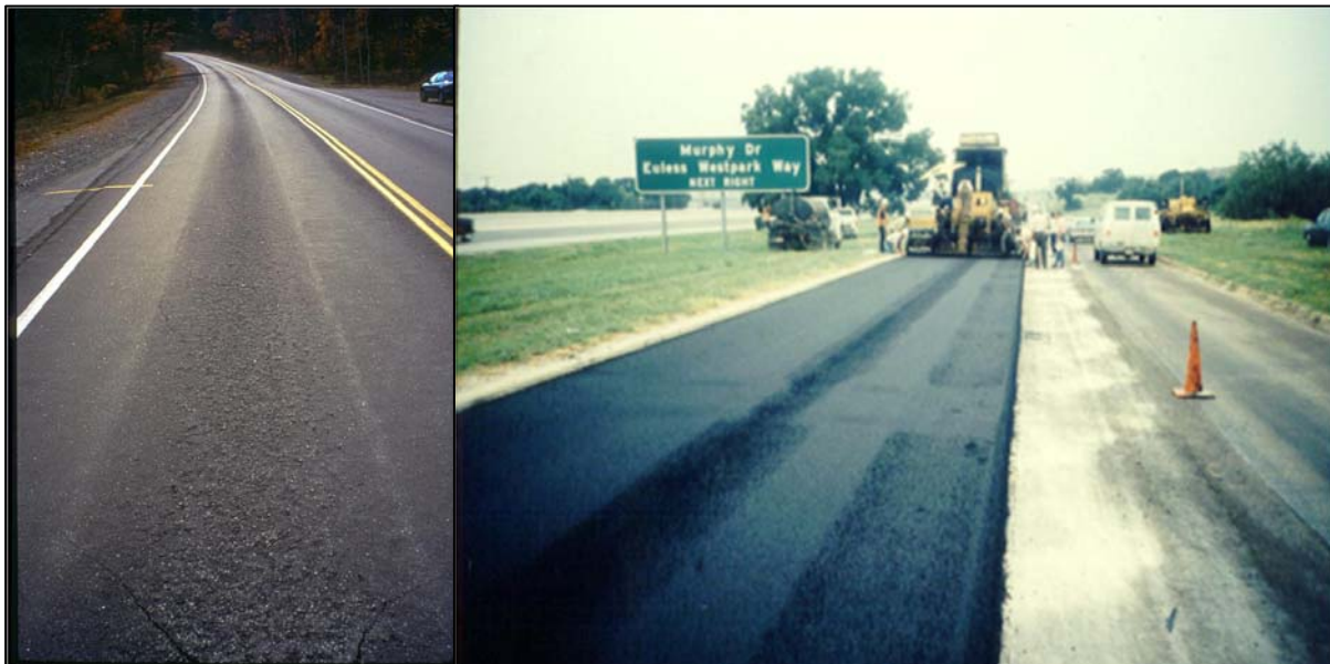
Figure 50. Cracking and Deterioration Along the Center of the Lane where the HMA was Improperly Placed
