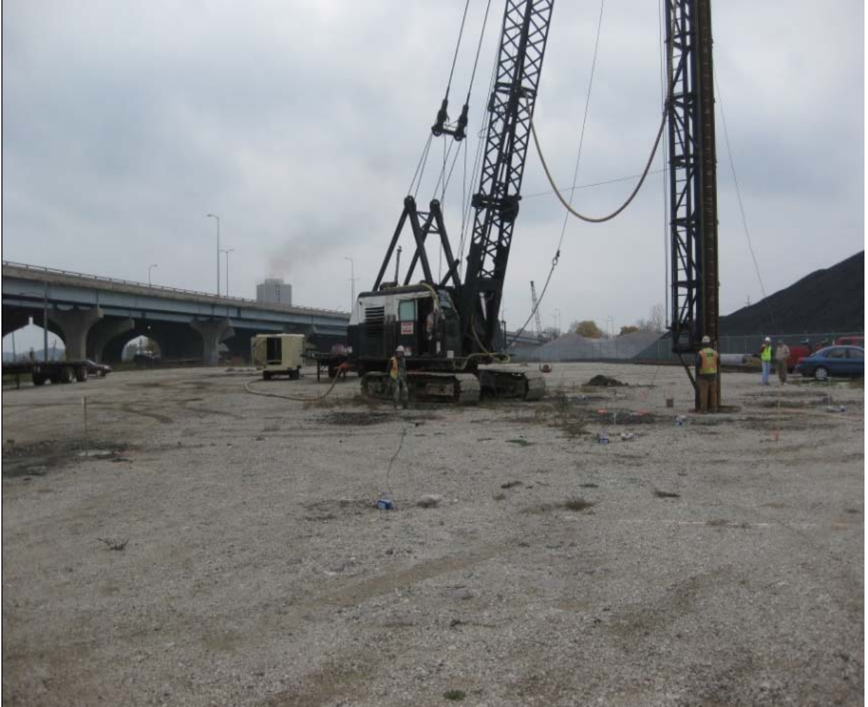
Figure 6.7 View of Edward E. Gillen Co. Pile driving hammer, crane and compressor during vibration monitoring at Test Pile #1
