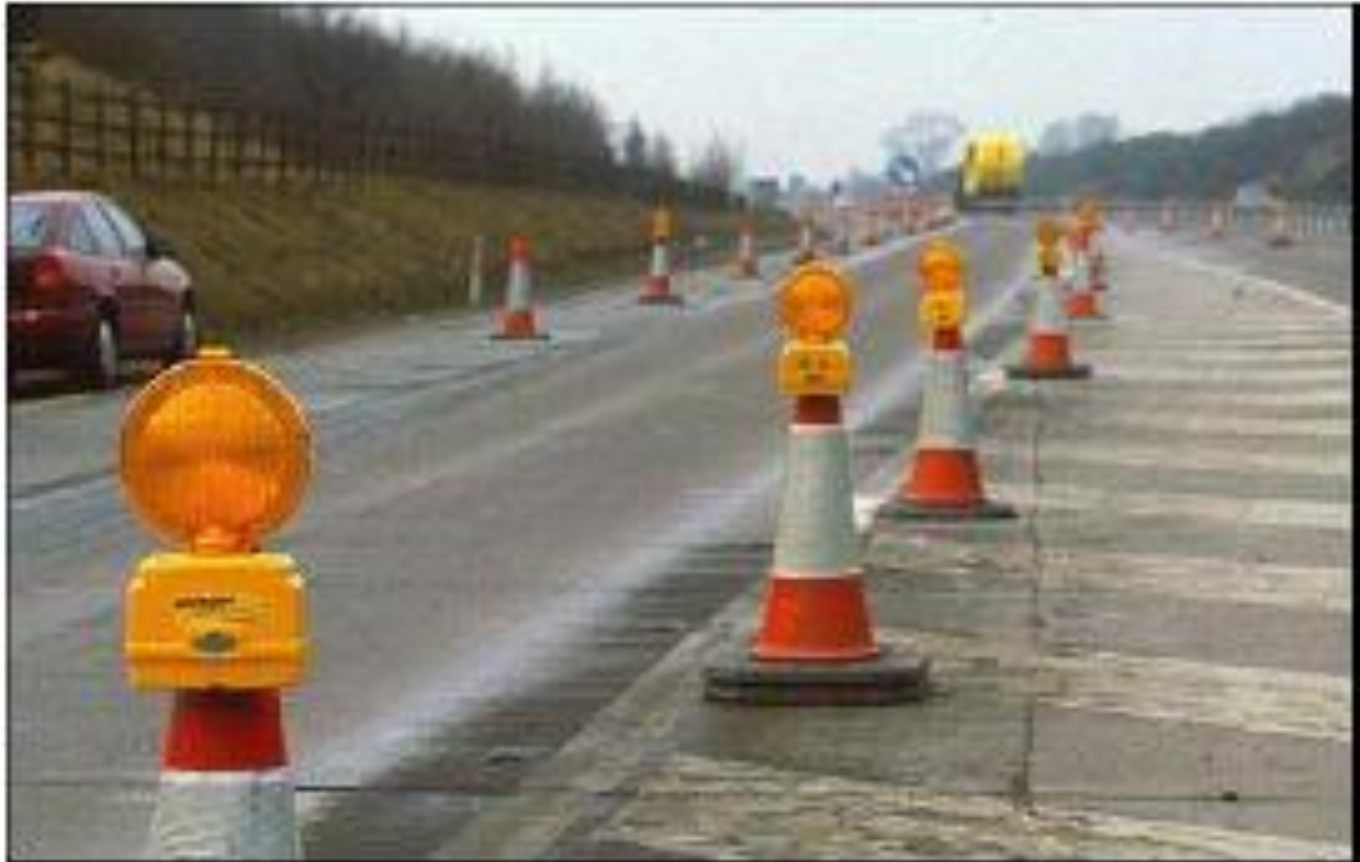
FIGURE 2 Sequential warning light (HA, 2005b).
